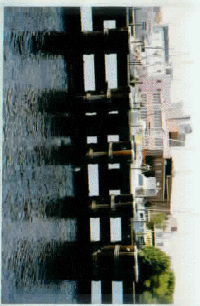
WOOD PIER FENDER - SMOKE
