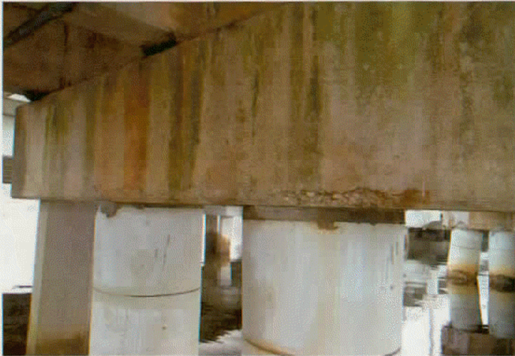
BENT #6 CAP BOTTOM EDGE OVER PILE #2 AND #3 CRACKED, SPALLED AND DELMINATED
