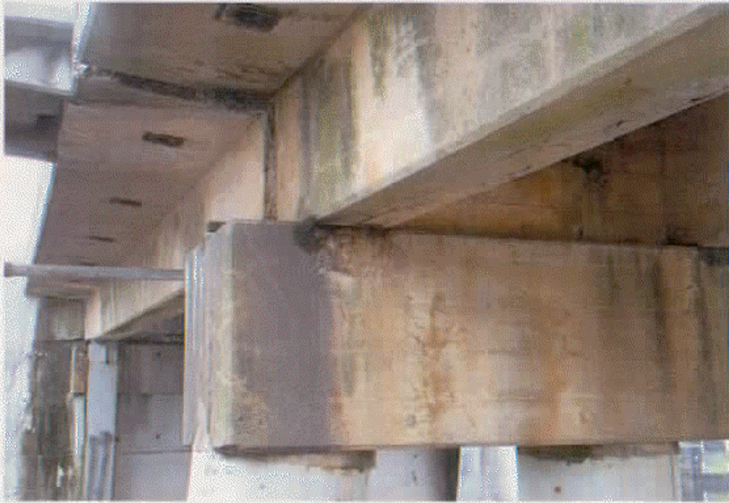
BENT #5 CAP SPALLED UNDER GIRDER #1
