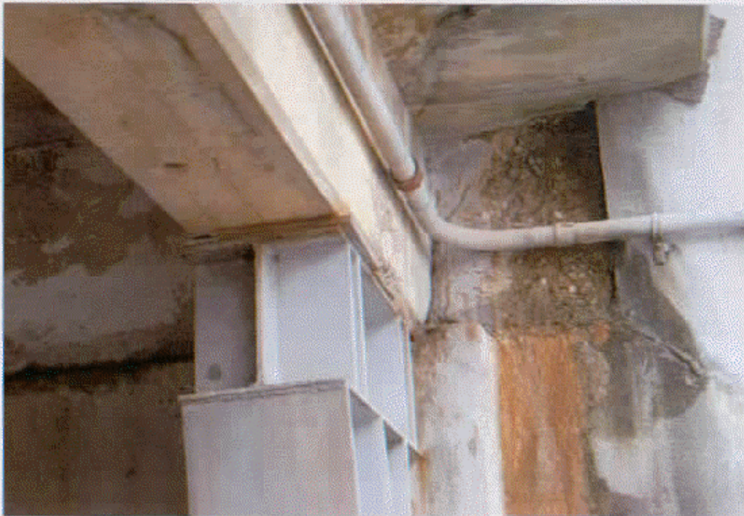
REST PIER #1 RIGHT SIDE OF GIRDER #1 CRACKED, SPALLED AND DELMINATED
