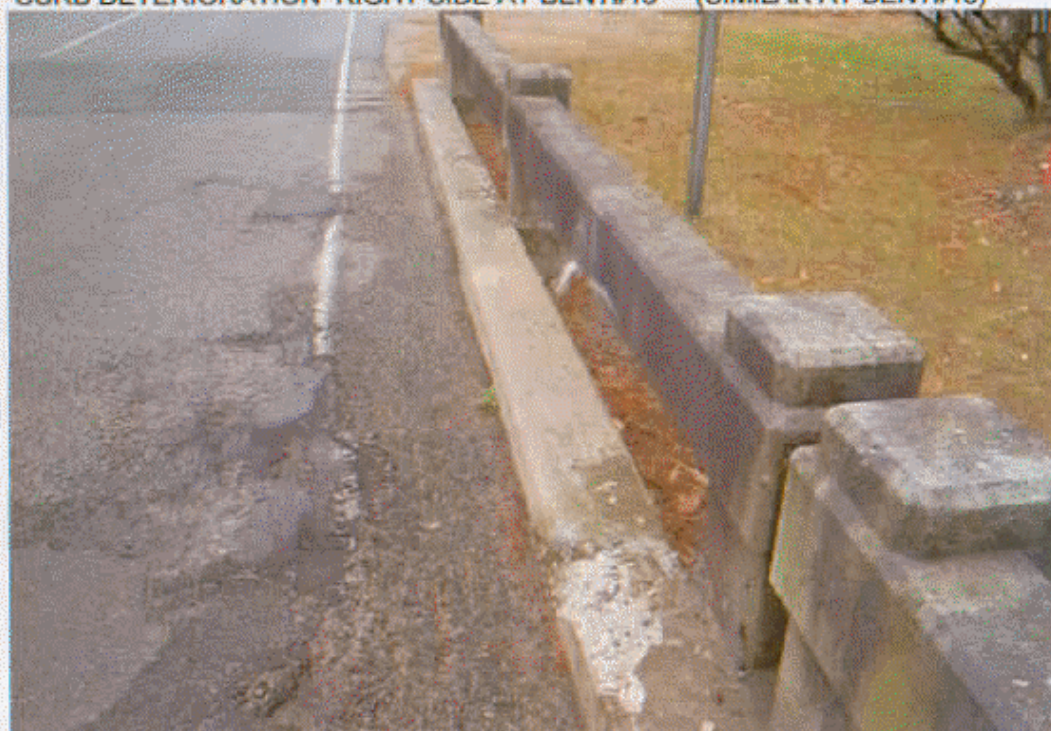
CURB DETERIORATION AT RIGHT SIDE LAST THREE SPANS
