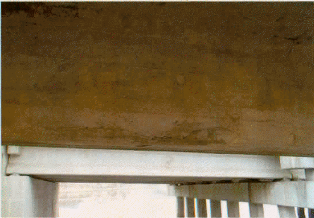
RIGHT BOTTOM EDGE OF GIRDER #1 SPAN #7 CRACKED & DELMINATED FROM REST PIER #2 TO MID SPAN
