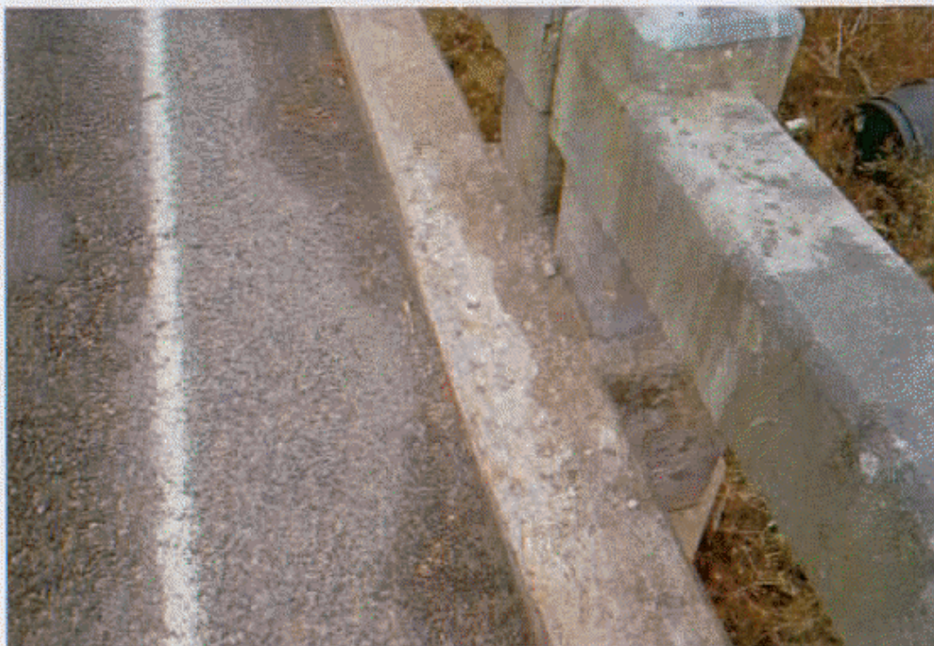
CURB DETERIORATION RIGHT SIDE AT BENT#16 (SIMILAR AT BENT#18)
