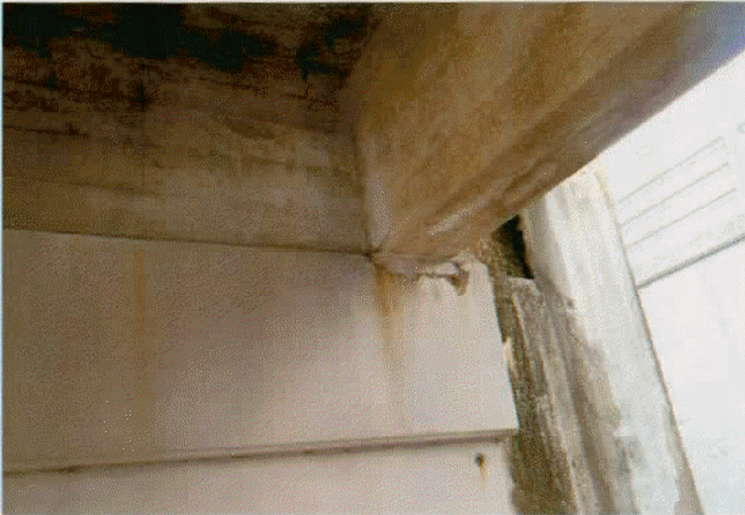
AT REST PIER #2 UNDER GIRDER #1 CRACKED, SPALLED AND DELMINATED
