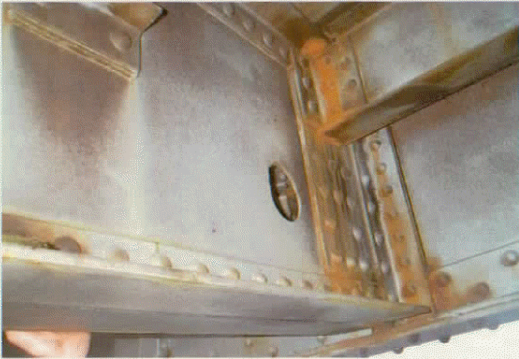
HOLE IN FLOORBEAM WHERE ARM WENT THRU
