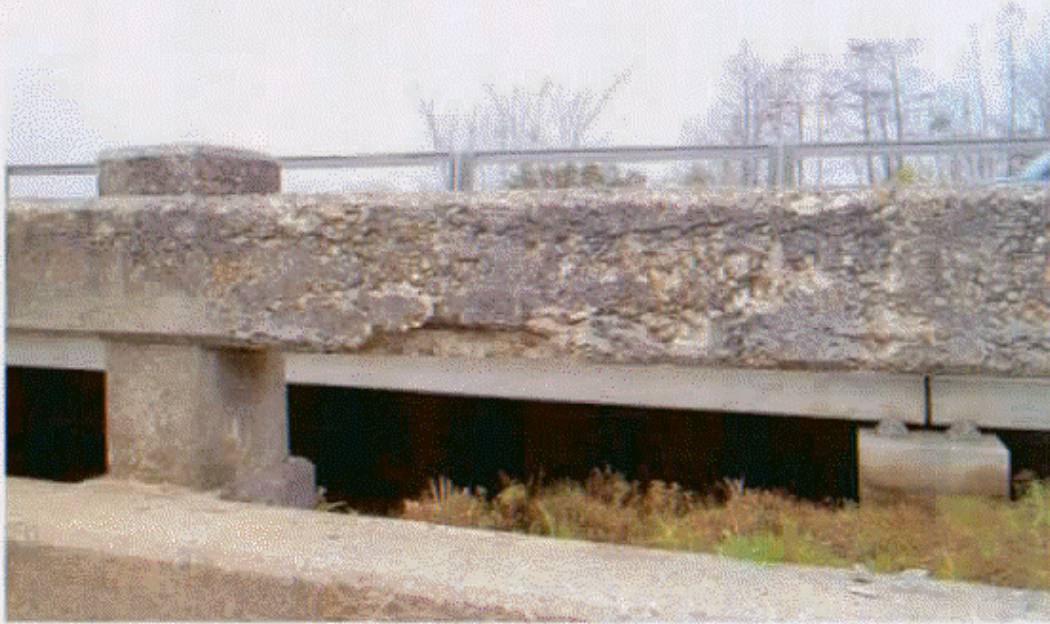
EXTERIOR OF LEFT CURB BETWEEN BENT #14 AND BENT #15 HEAVY DETERIORATION WITH RE-STEEL EXPOSED
