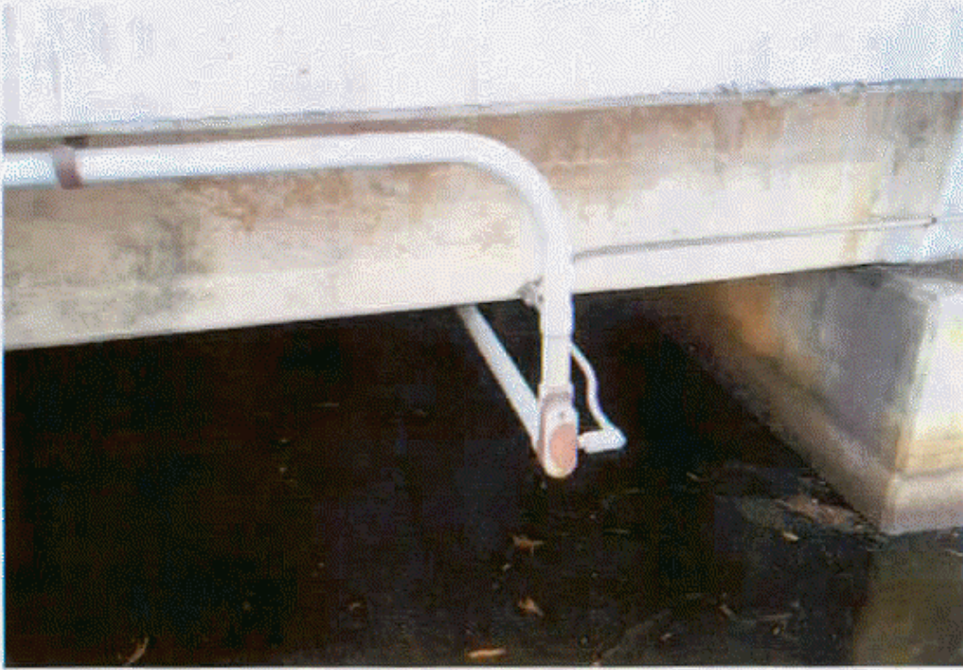
UTILITIES RIGHT SIDE
