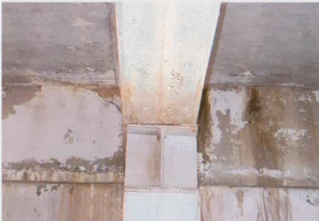
BOTTOM OF GIRDER #2 SPAN #6 AT REST PIER#1 AT SUPPORT BEAM PLATE AND CRACK AT BOTTOM OF GIRDER
