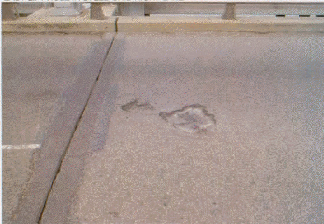
WEARING SURFACE SPALLED LEFT LANE SPAN #7 AT BENT#6
