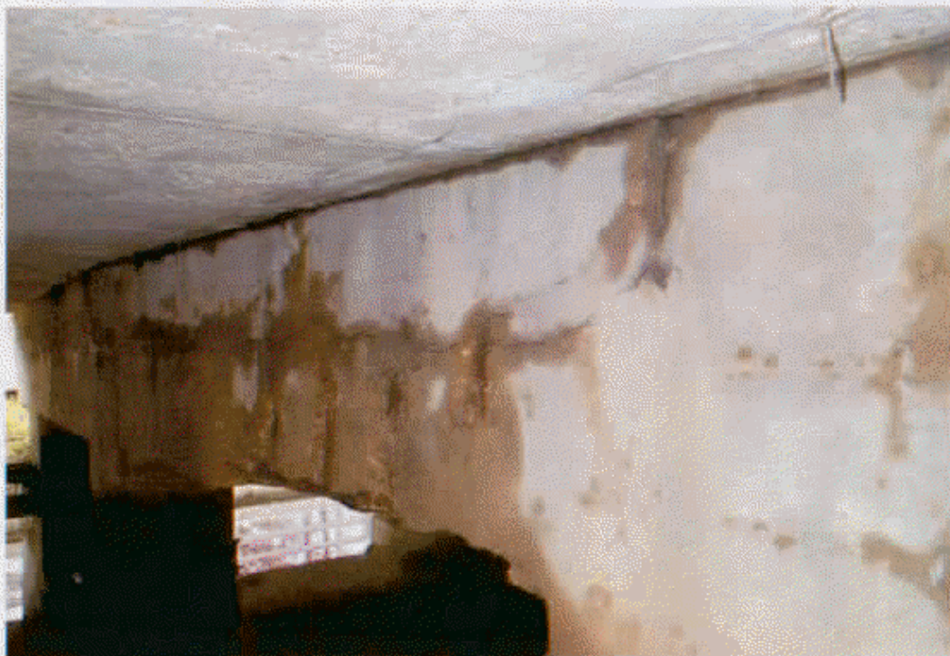
WEST FACE OF BENT #25 CAP (CRACKED, SPALLED AND DELMINATED WITH RE-STEEL EXPOSED)
