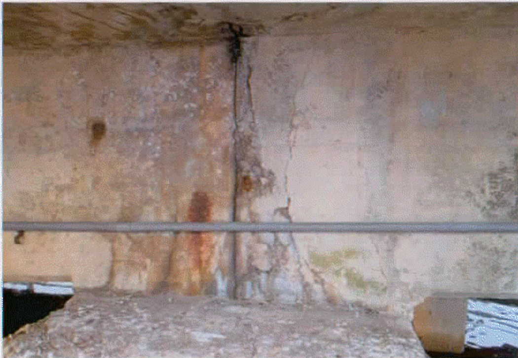
RIGHT SIDE GIRDER #4 AT BENT #2 SPAN #3 CRACKED, SPALLED AND DELMINATED
