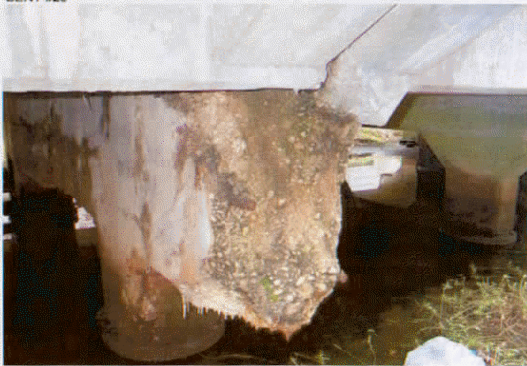
RIGHT END OF BENT #25 (HEAVY DETERIORATION)
