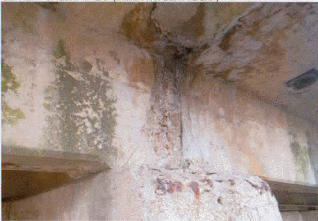
LEFT SIDE OF GIRDER #1 AT BENT #4 (DETERIORATION )
