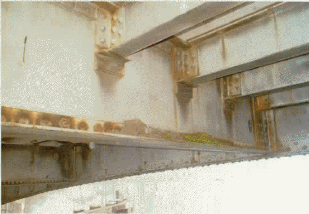
EXCESS DIRT ON BOTTOM FLANGE OF FLOOR BEAMS
