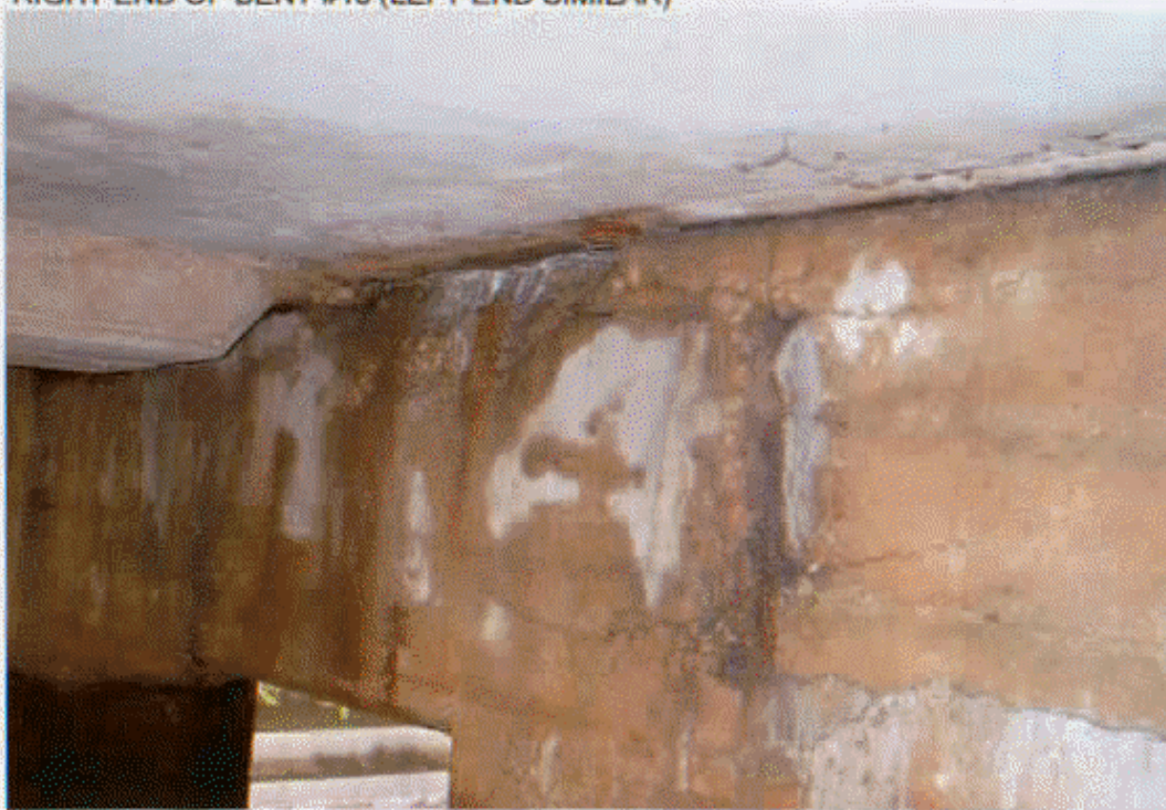
WEST FACE OF BENT#18 CAP (CRACKED, SPALLED AND DELMINATED AND WITH RE-STEEL EXPOSED)
