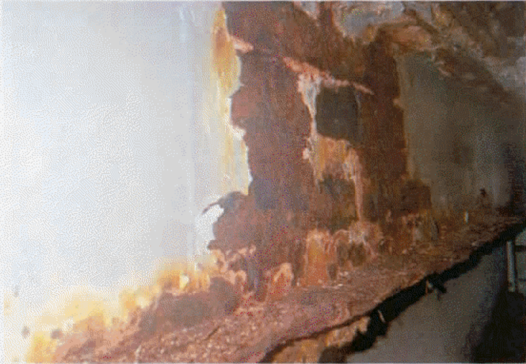
STRINGER #6 AT WEST END HEAVY SECTION LOSS WEBB 3/16" FLANGE 5"
