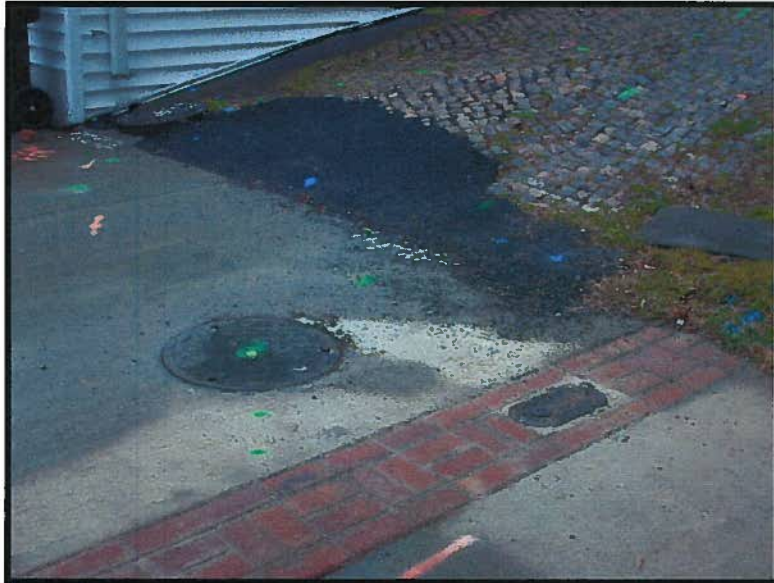
5 View of manholes and subsurface utilities on eastern side of Parcel 1 (Vestal Property).
