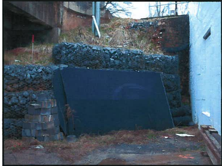
14 View of debris and retaining walls on western side of Parcel 1 (Haney Property).
