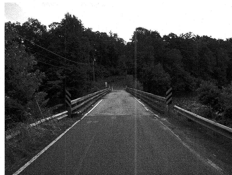
Photograph No. 12: This photograph was taken from the north approach, along the centerline of the -L- alignment, looking southeast.
