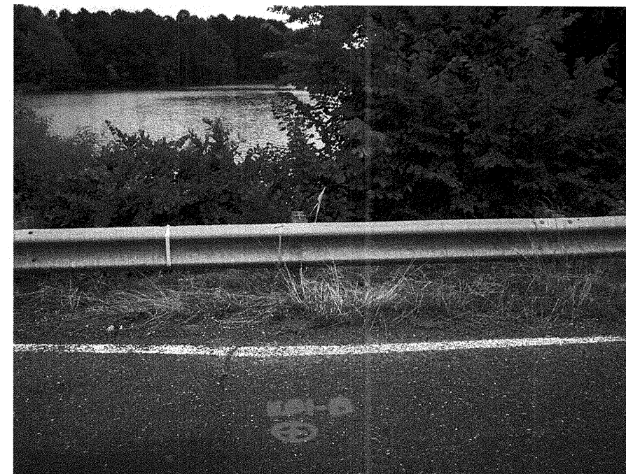
Photograph No. 3: This photograph was taken from the centerline of the -L- alignment, looking east, across End Bent No. 1.
