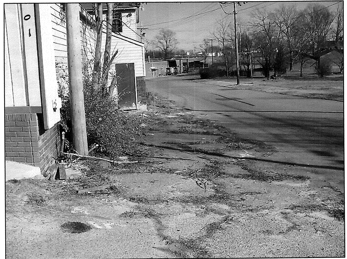
BENT 1, LOOKING LEFT TO RIGHT FROM INTERSECTION OF WILSON LEE BLVD AND ASHEVILLE AVE.
