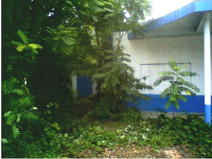
Photograph 1 – View of the west side of the vacant building on the Arnold Robbins property.
