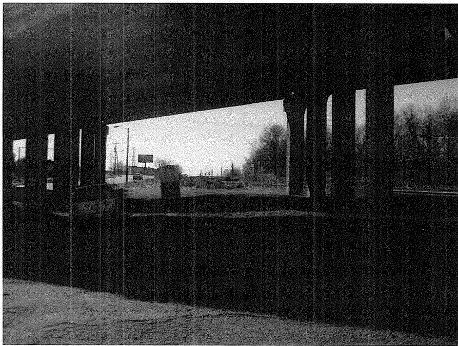
Photograph No. 10: This photograph was taken from the right side of the -L- alignment, looking south, across proposed Interior Bent No. 1.
