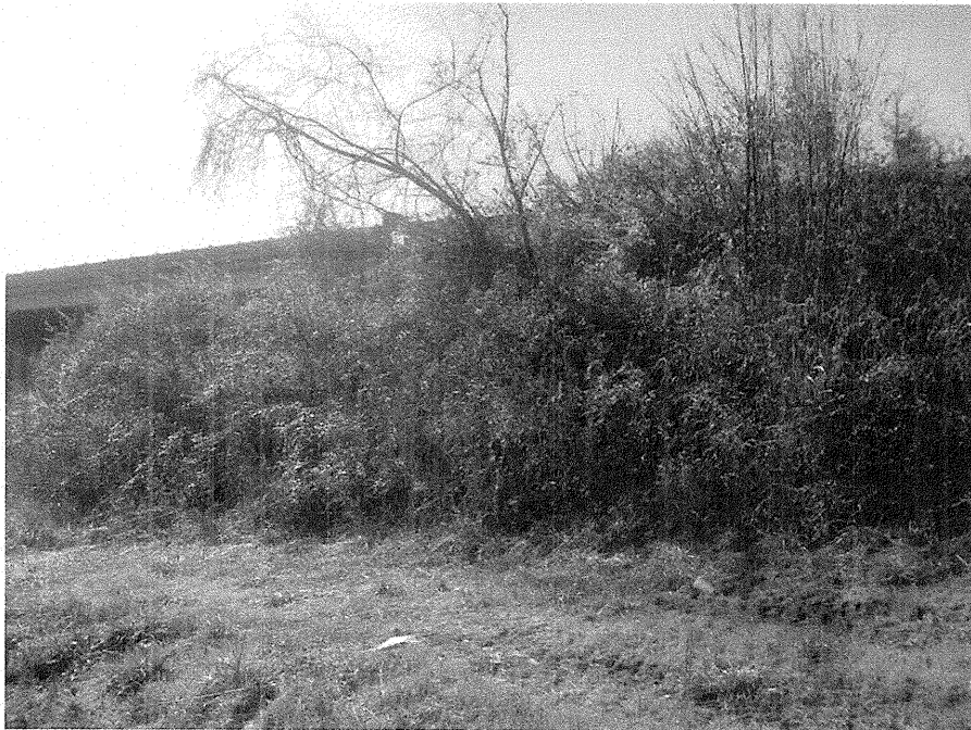
Photograph No. 14: This photograph was taken at the toe of the existing embankment from the right side of the -L- alignment, looking south, across proposed End Bent No. 2.
