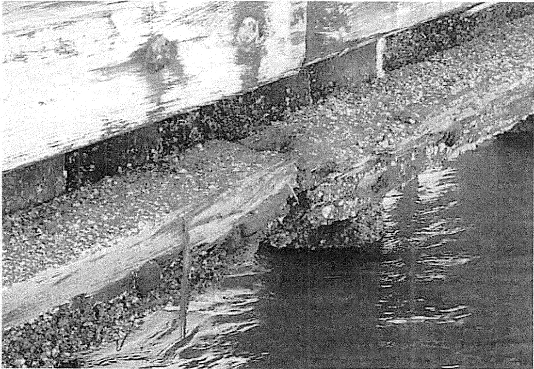
BORER DAMAGE LOWER WALERS
