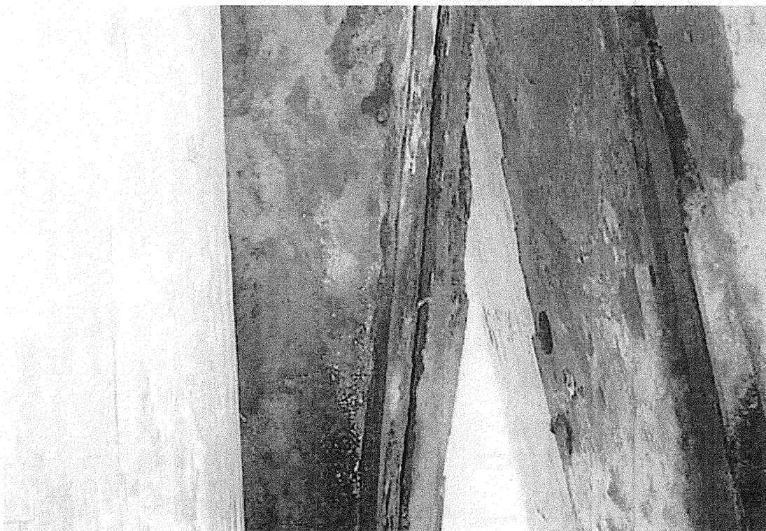
NE DOLPHIN RUSTED H-PILE
