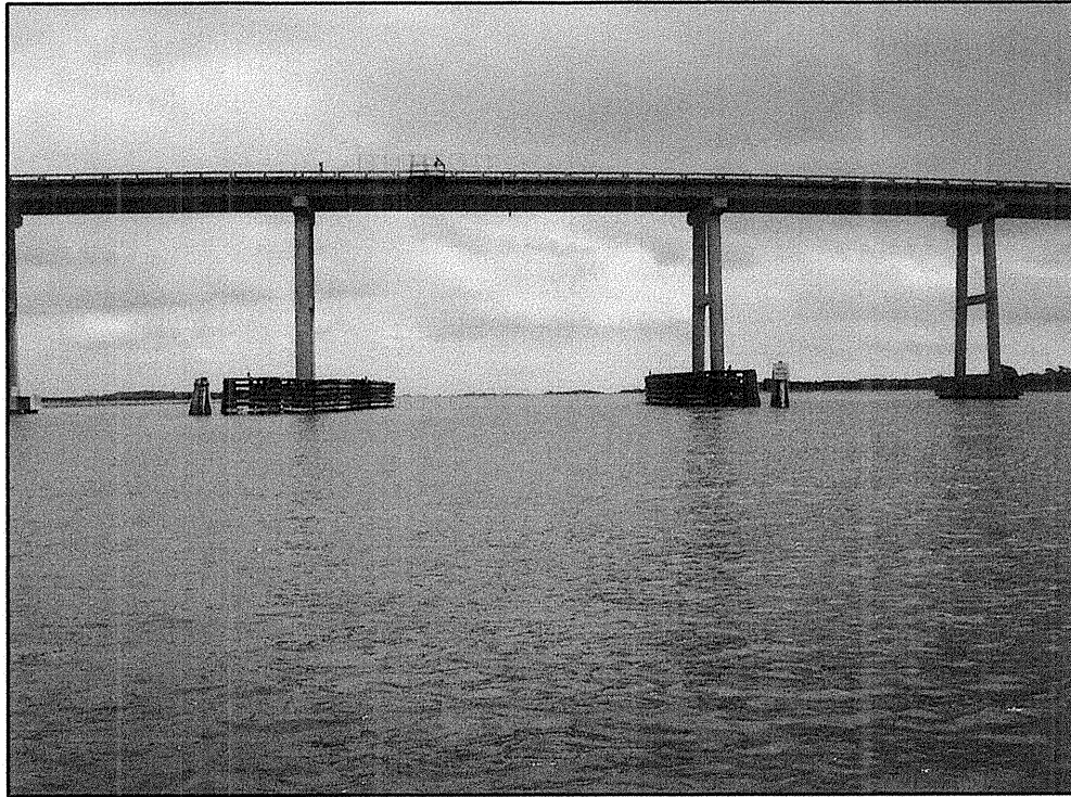
WEST OF BRIDGE #6 FACING EAST NORTH FENDER ON LEFT SOUTH FENDER ON RIGHT
