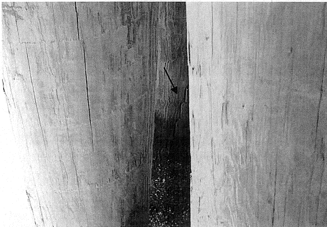
NE DOLPHIN BROKEN PILE
