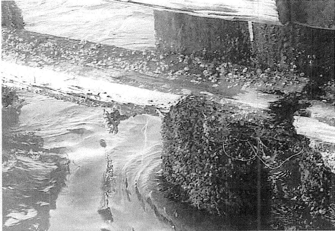
BORER DAMAGED LOWER WALERS
