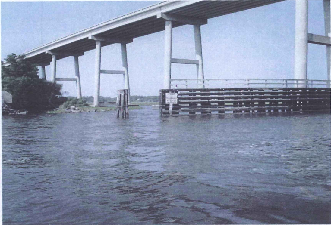
S.E. FLARE AND CLEARANCE MARKER
