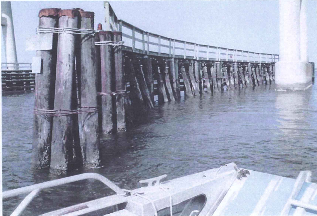
BACKSIDE NORTH FENDER
