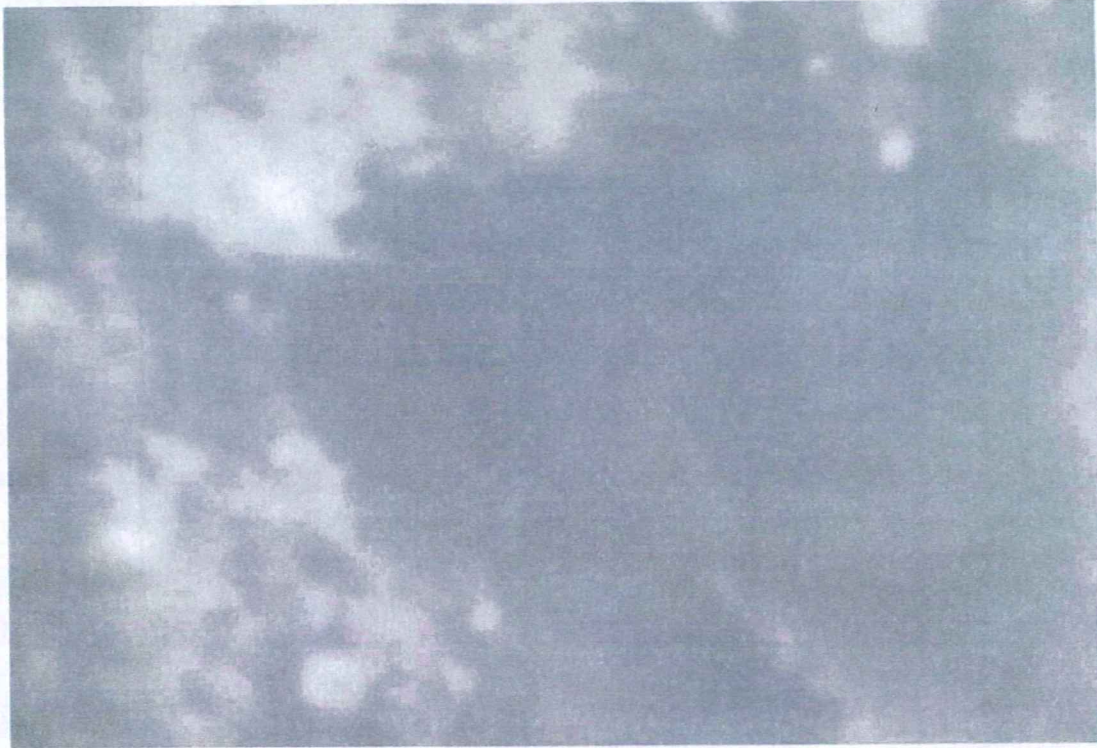
3" DEEP X 3" DIAMETER BORER HOLE IN PILE, S.FENDER
