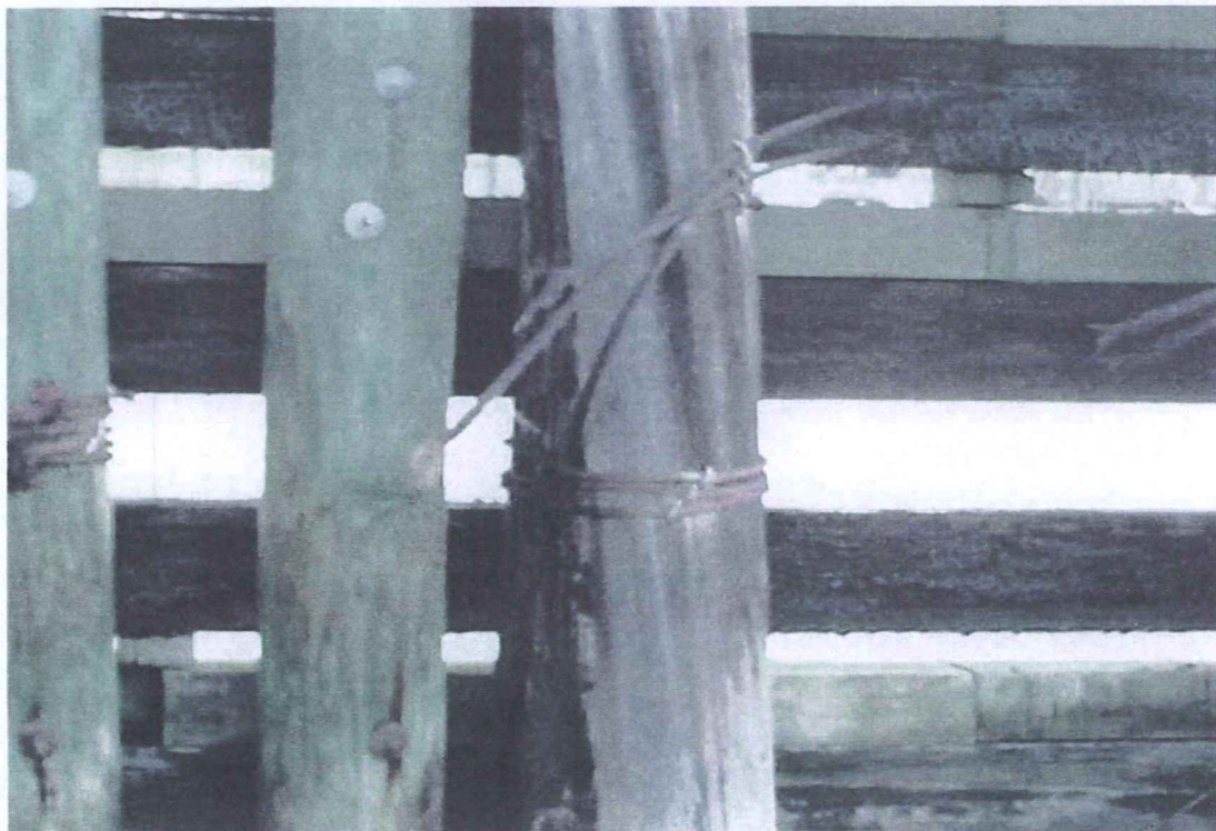
BROKEN RUSTED CABLE WRAPS, S.FENDER
