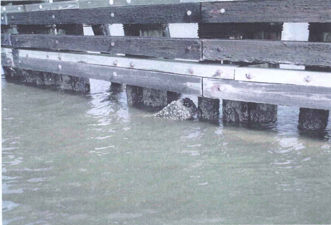
BROKEN HANGING WALER, N.FENDER
