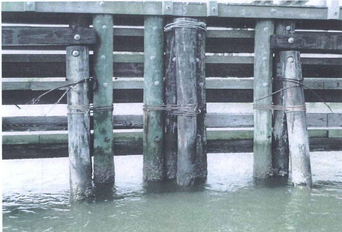
RUSTED BROKEN CABLE WRAPS
