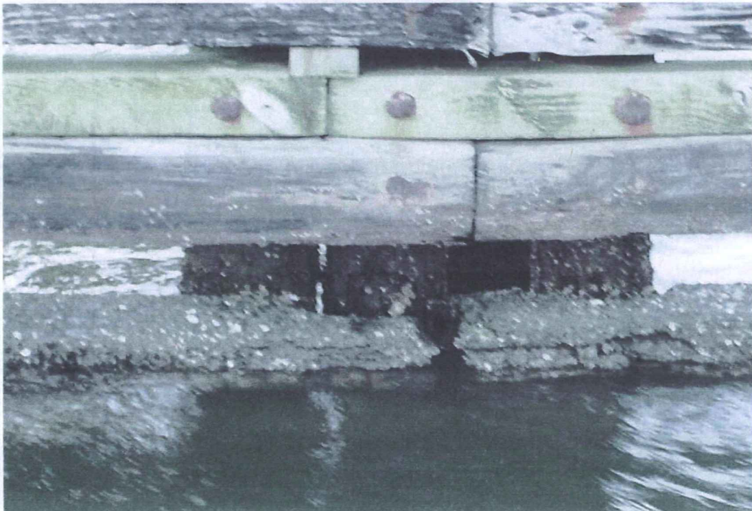
WALER DECAY, S.FENDER
