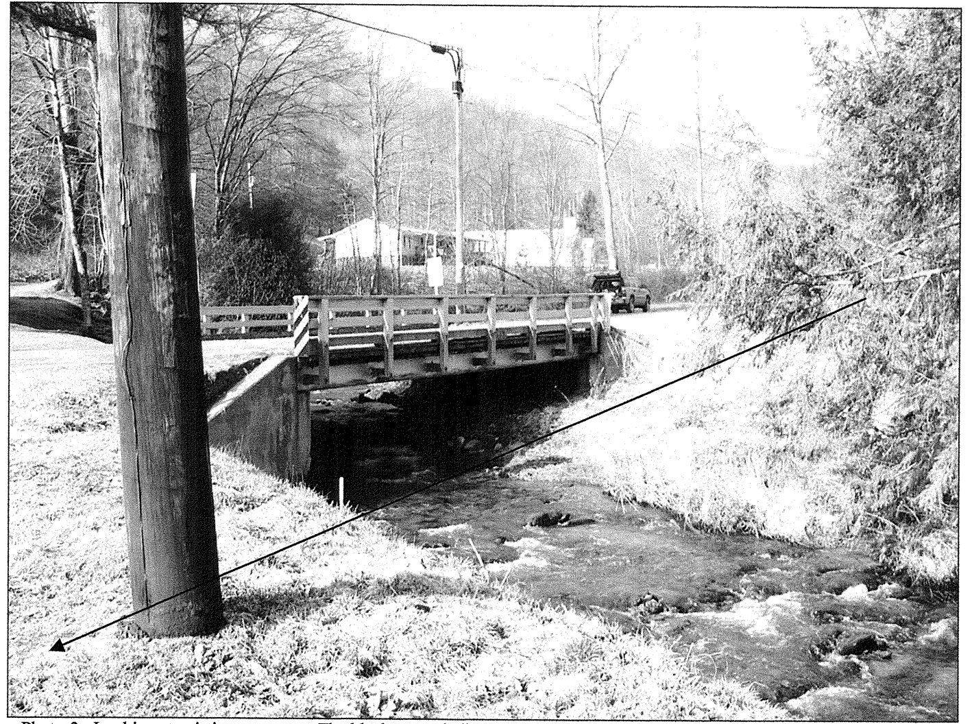
Photo-3: Looking at existing structure. The black arrow indicates the approximate location and orientation of -L- as it passes through the project area from right to left.
