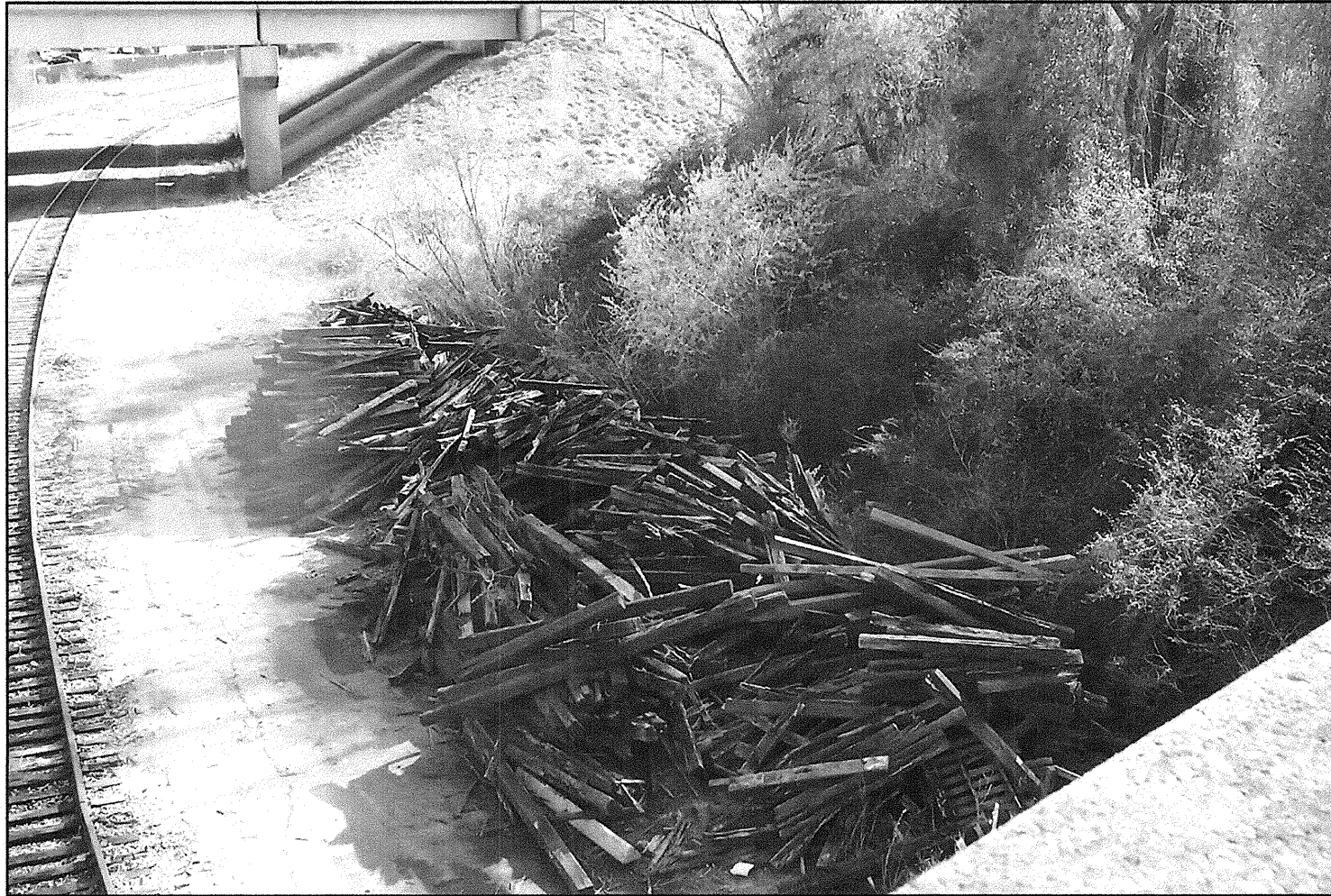
RETAINING WALL 1 (WESTERN SIDE) AREA LOOKING FROM EXISTING BRIDGE 26 TO THE SOUTH. NOTE: LARGE PILE OF CROSSTIES UPSTATION OF PROPOSED WALL.
