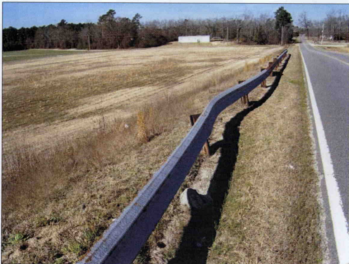
GUARDRAIL DAMAGE 14 FT. LONG AT SOUTHWEST CORNER
