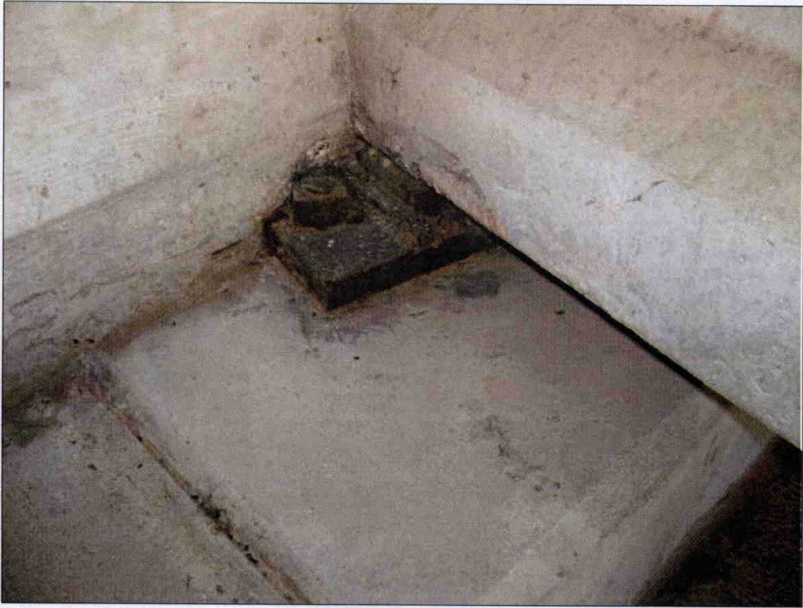
SURFACE RUST AT BEARING ASSEMBLY GIRDER 3 EB1
