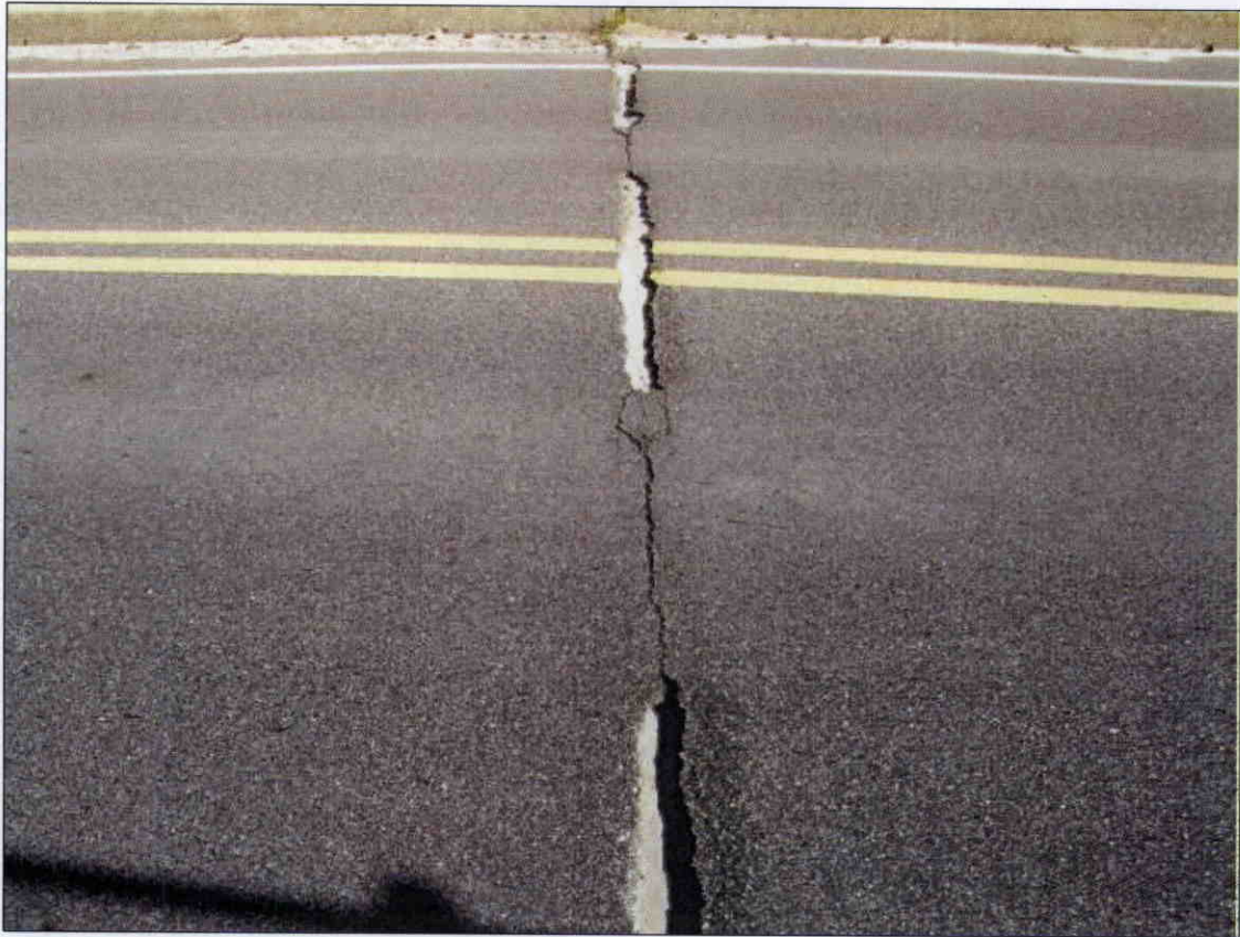
ASPHALT WEARING SURFACE CRACKING 3 IN. AND 4 IN. WIDE AT BENT 3 EXPANSION JOINT
