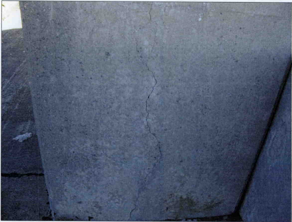
1/32 IN. VERTICAL CRACK ON NORTH FACE OF BENT 3 COLUMN 1 AT CENTER OF COLUMN
