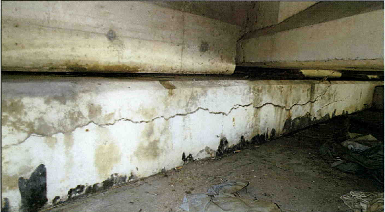
ABUTMENT 1 CAP LONGIT CRACK UP TO 1/2 INCH WIDE UNDER BAY 4
