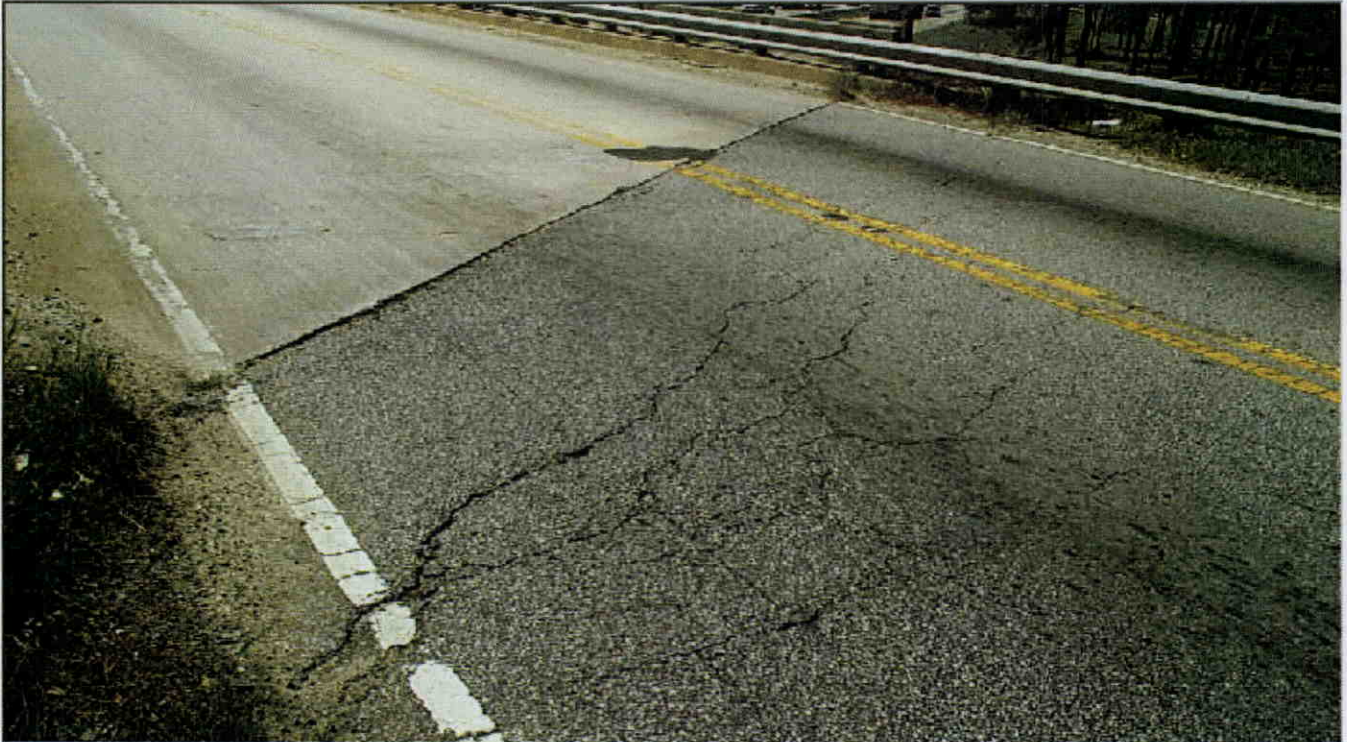
WEST APPROACH CRACKED AND SETTLED UP TO 1 IN. WITH ROUGH PAVEMENT
