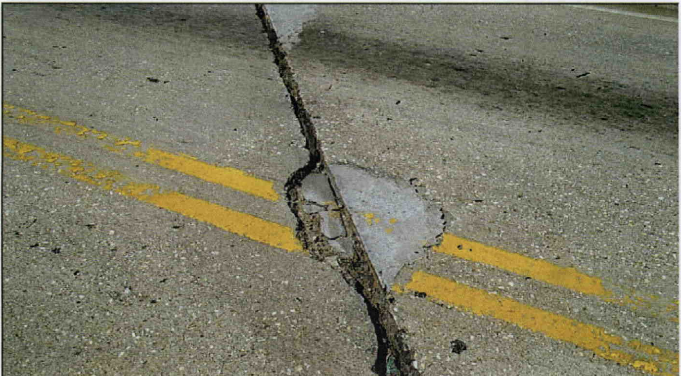
TOP OF DECK SPAN 4 AT PIER 3 JOINT IN.D IN.SPALLED
