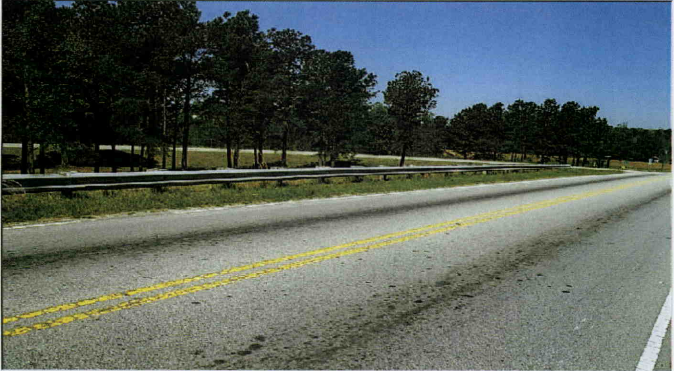
GUARDRAIL POSTS AT MIDWAY
