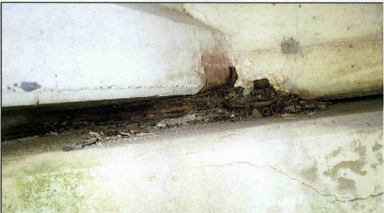
BEARING 5, ABUTMENT 1, HEAVY RUST WITH SECTION LOSS, ALL BEARINGS AT ABUTMENTS SIMILAR.
