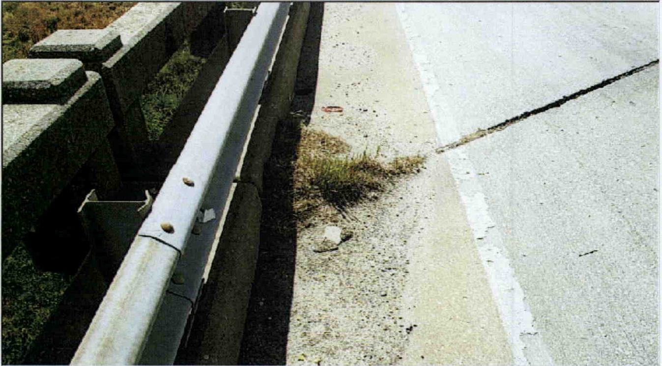
DEBRIS ALONG CURBS, SAND AND GRAVEL UP TO 4 INCHES DEEP SOME AREAS.
