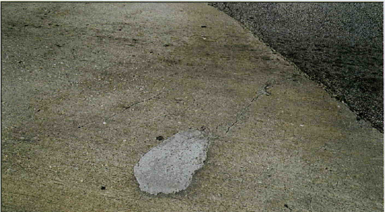
TOP OF DECK SPAN 1, DIAGONAL CRACKS, OTHER SPANS SIMILAR
