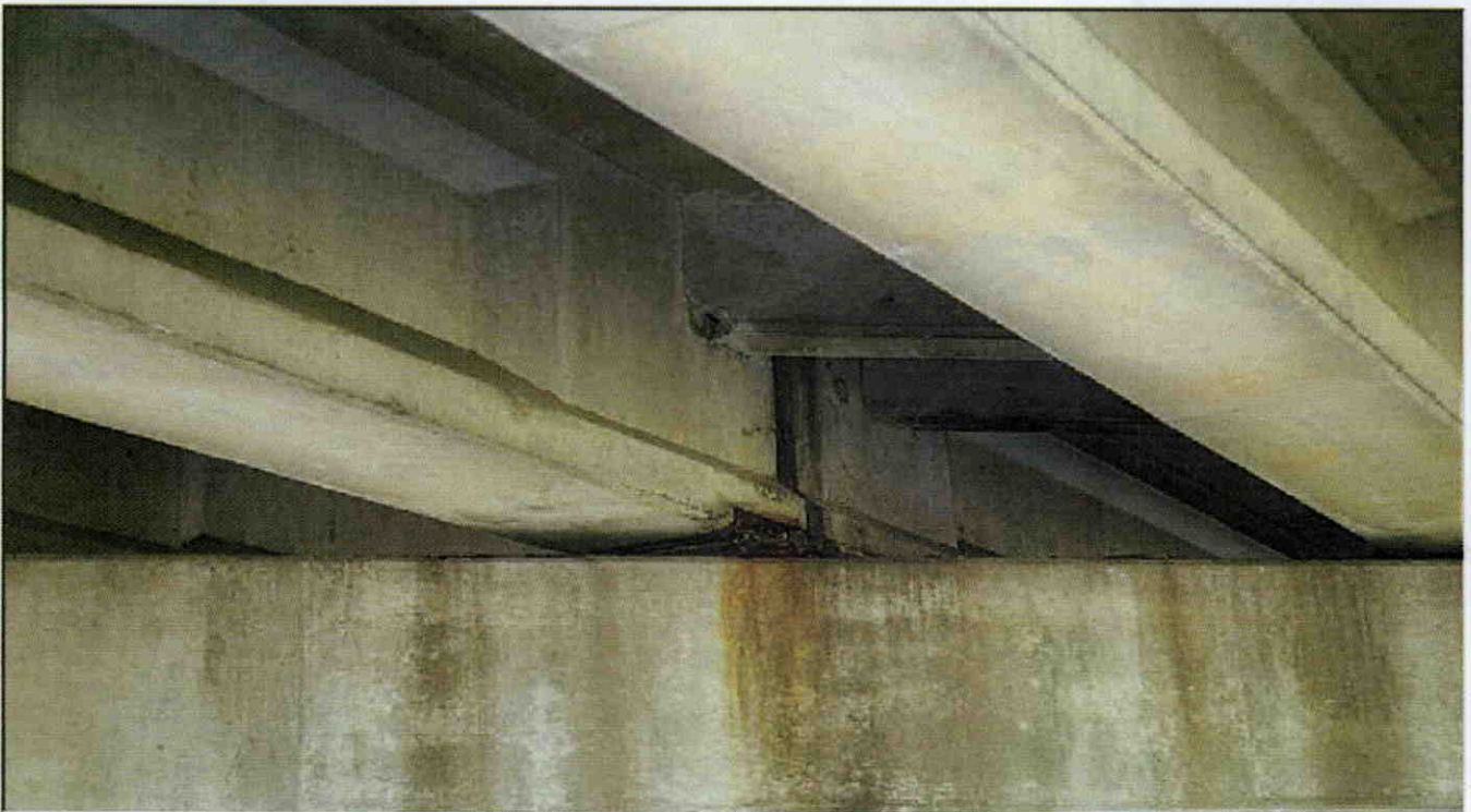
BEARING 3 AT PIER 1, HEAVY RUSTING AND FLAKING, ALL SIMILAR
