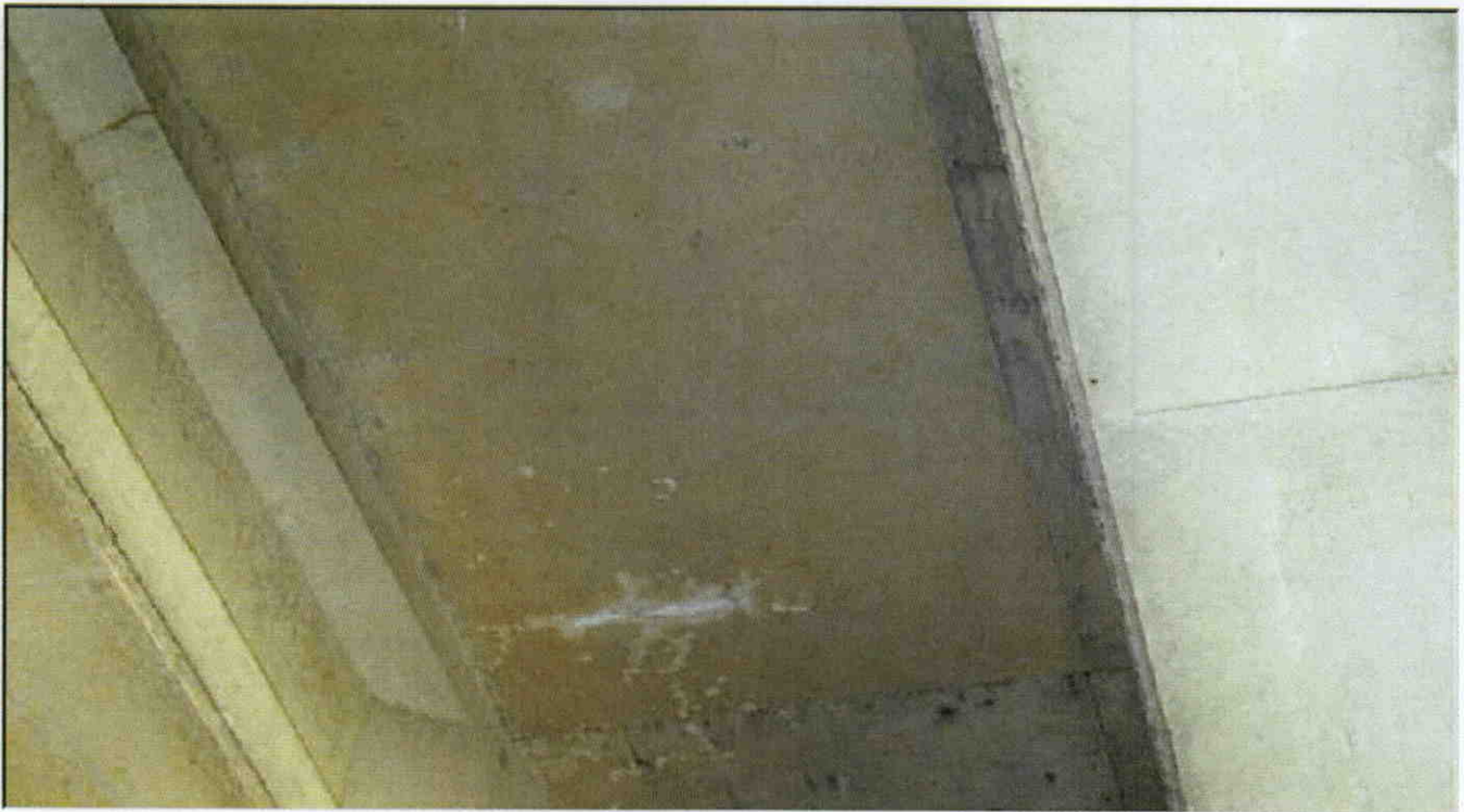
BOD, SPAN 1, BAY 4 TRANS CRACKS WITH EFFLO OTHER BAYS SIMILAR
