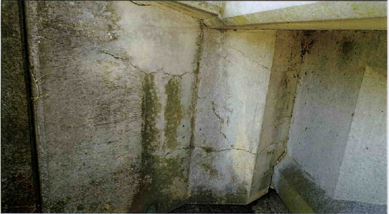
BACKWALLS ABUTMENT 1, LEFT OF GIRDER 1 MAP CRACKS WITH EFFLO, OTHERS SIMILAR.
