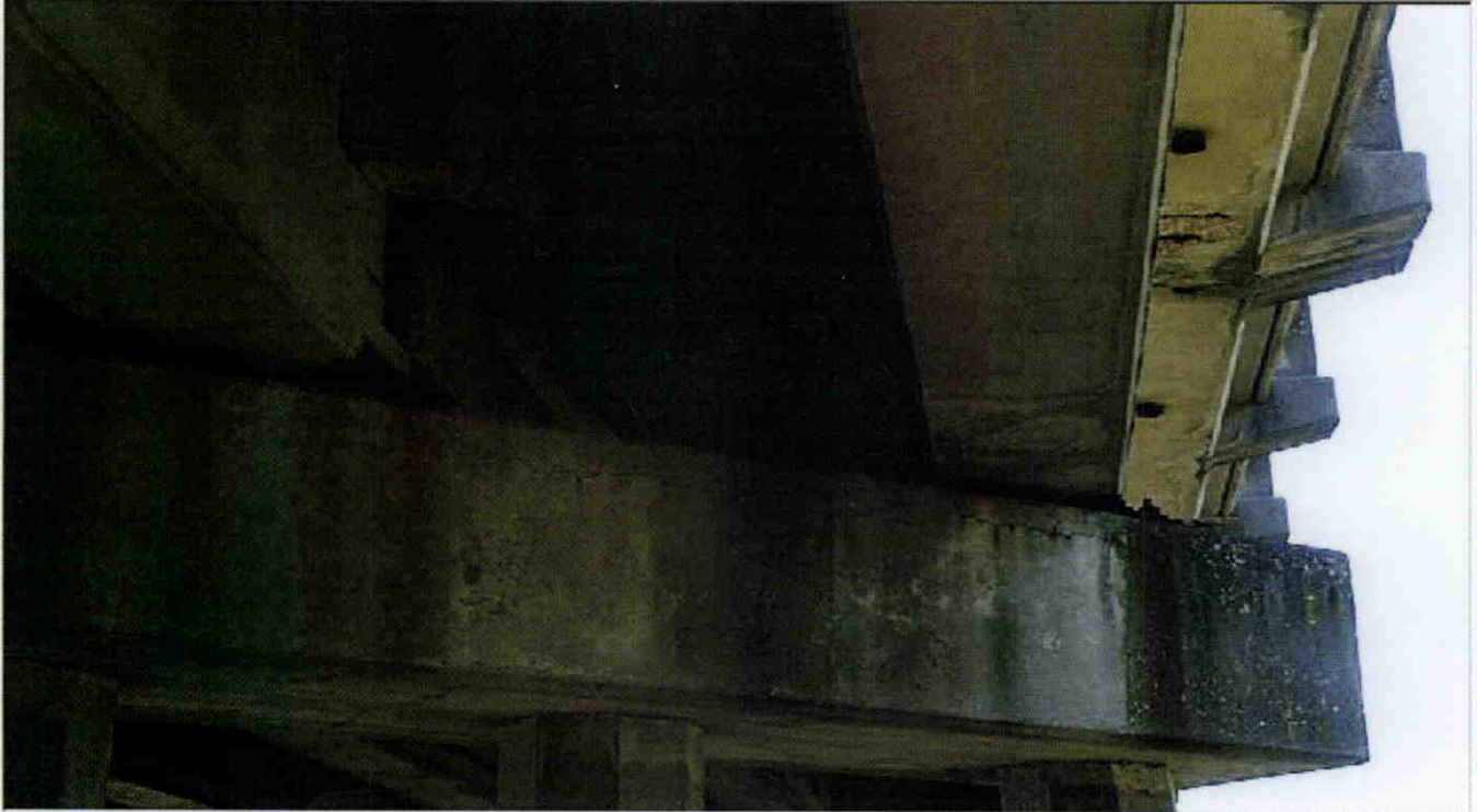
PIER 1 CAP SPAN 1 FACE LONGIT CRACKS, ALL CAPS SIMILAR
