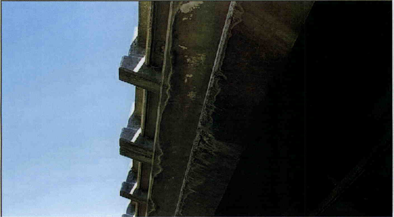
GIRDER 5, SPAN 3, SPALLS IN BOTTOM OF GIRDER.
