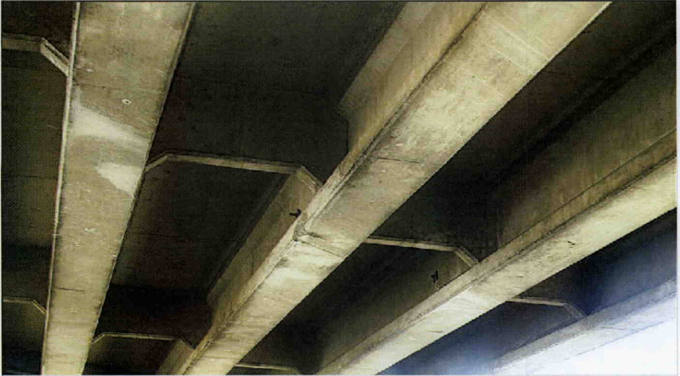
GIRDER 3, SPAN 3 SPALLED ON BOTTOM FROM HIGH LOAD..
