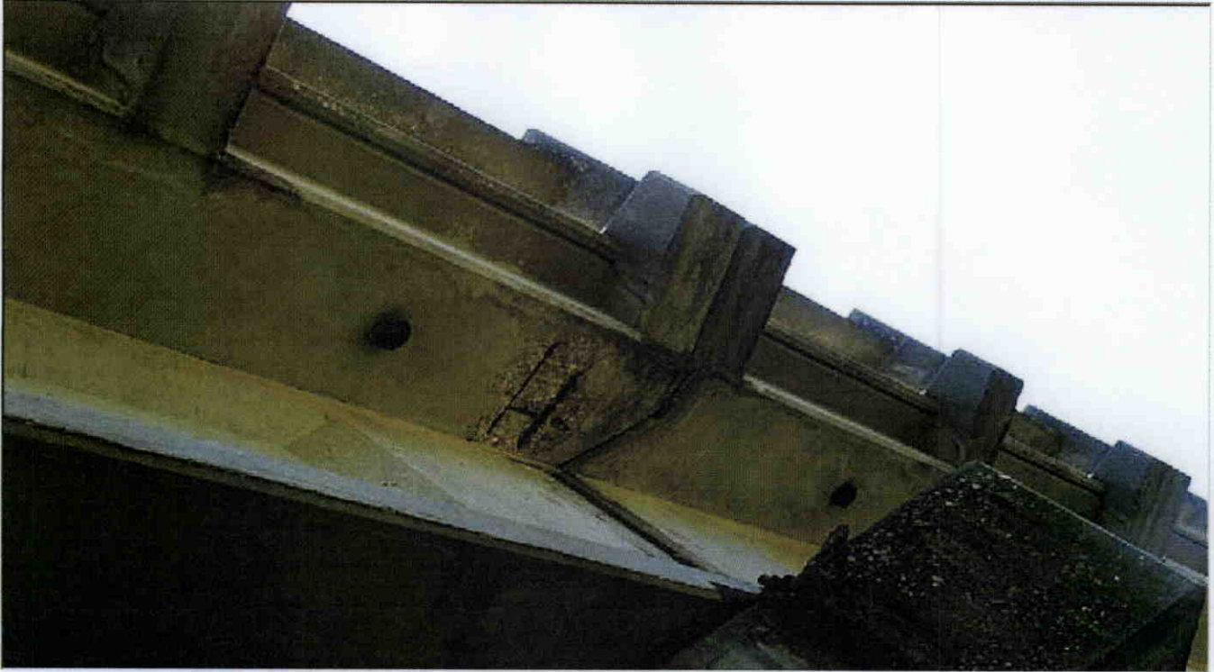
BOTTOM OF DECK SPAN 1, RIGHT OVERHANG SPALLED WITH REBAR EXPOSED, OTHER SPANS SIMILAR
