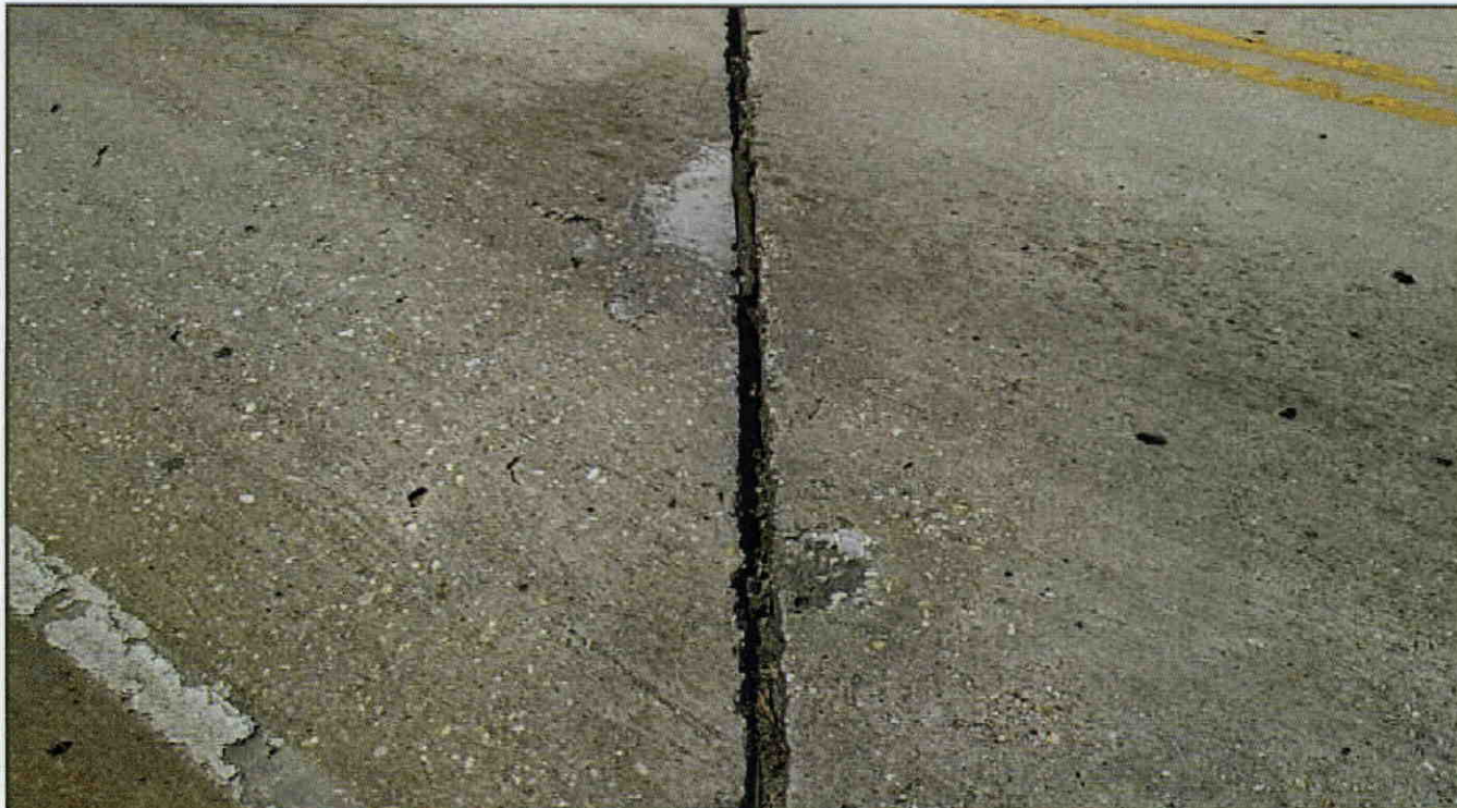
PIER 1 , EXPANSION JOINT MATERIAL MISSING, OTHERS SIMILAR
