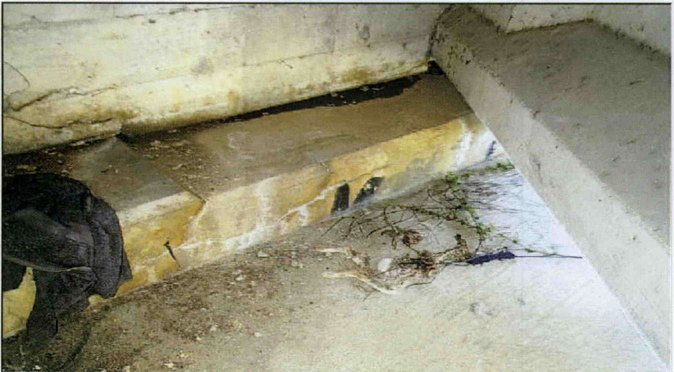
ABUTMENT 2 CAP IN BAY 4 MAP CRACKING WITH EFFLO
