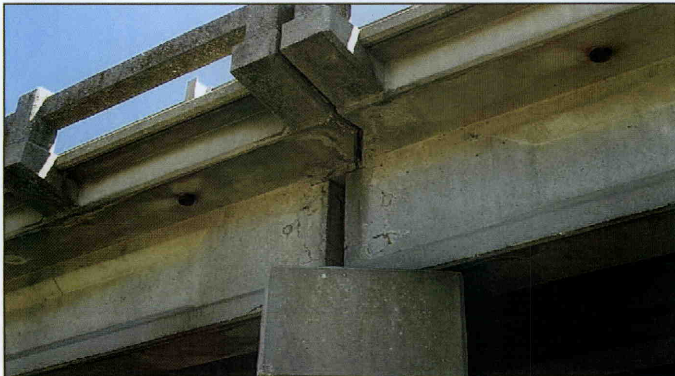
GIRDERS 5, SPANS 3 AND 4 AT PIER 3 MAP CRACKING ON ENDS WITH EFFLO STAINS.
