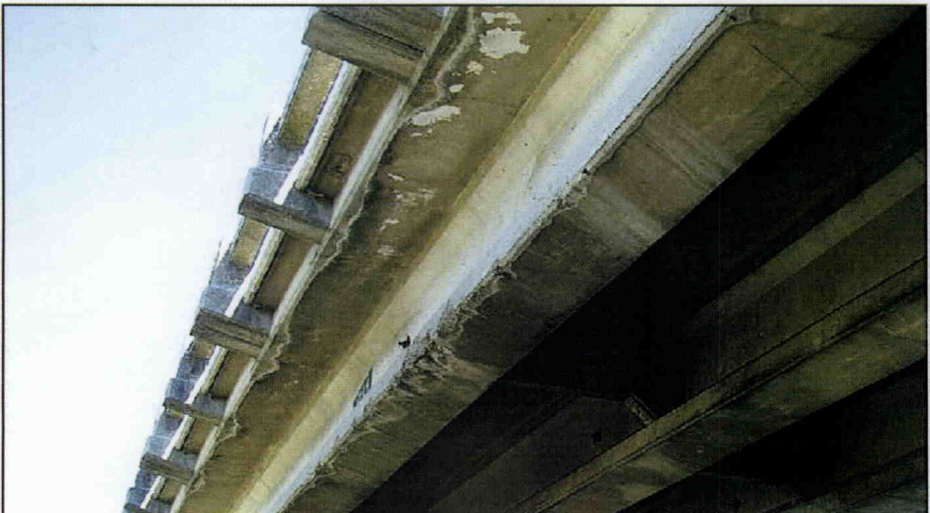
GIRDER 5, SPAN 3 BOTTOM RIGHT EDGE OF GIRDER SPALLED AND CHIPPED BBY HIGH LOADS.
