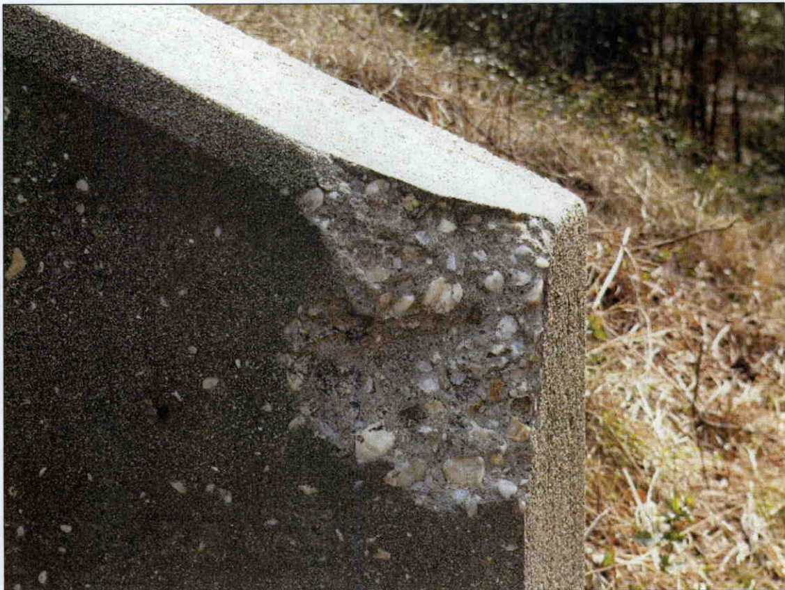
6 IN X 8 IN X 2 1/2 IN DEEP SPALL IN SOUTHEAST WINGWALL
