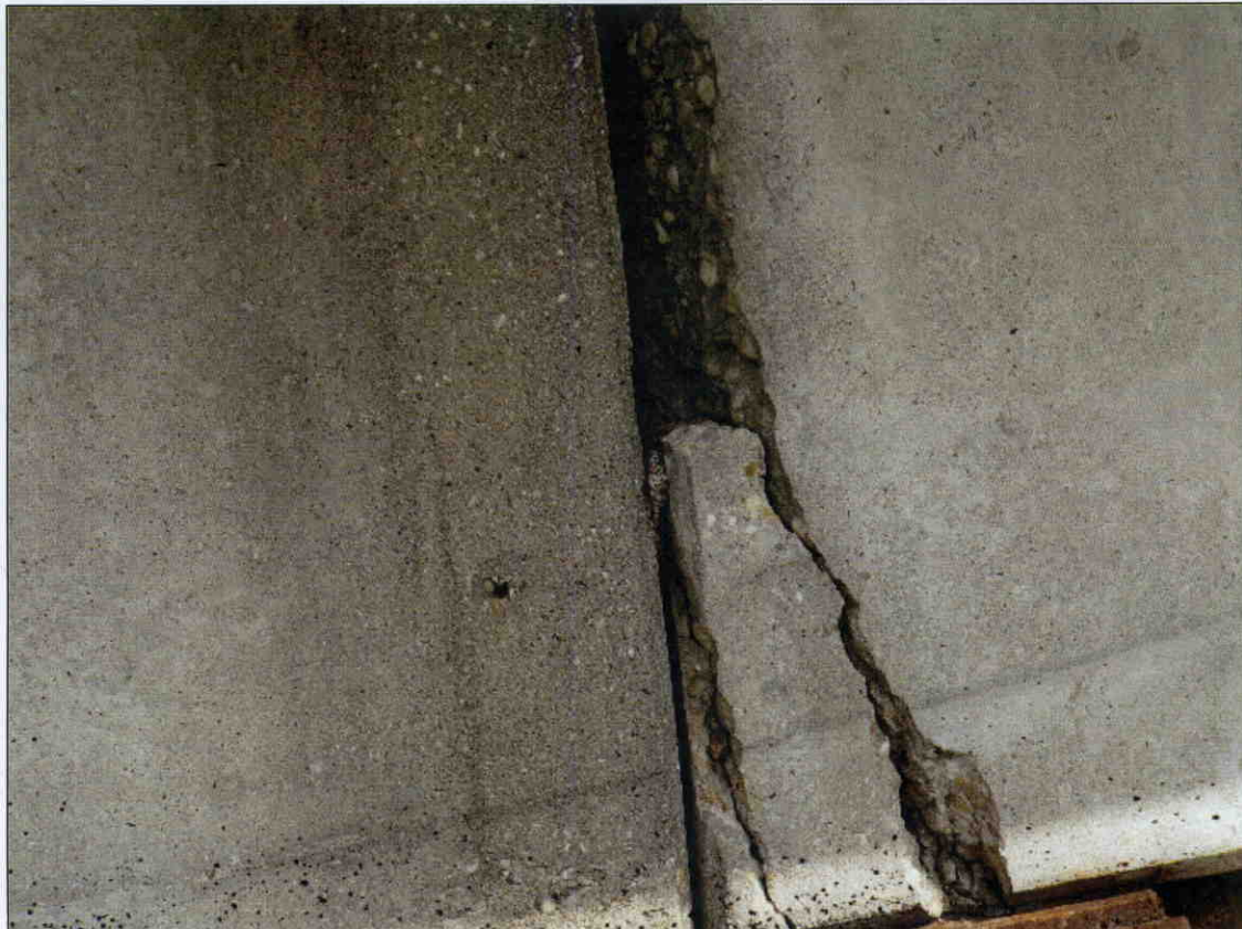
36 IN X 10 IN X 10 IN DEEP SPALL IN END OF GIRDER 4 AT BENT 2 IN SPAN 3
