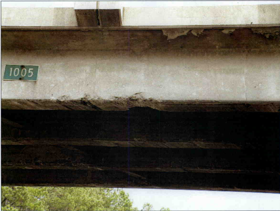
CHIPPING AND SPALLING OF GIRDER 4 DUE TO IMPACT DAMAGE IN SPAN 3, SIMILAR CONDITION AT GIRDERS 2 AND 3
