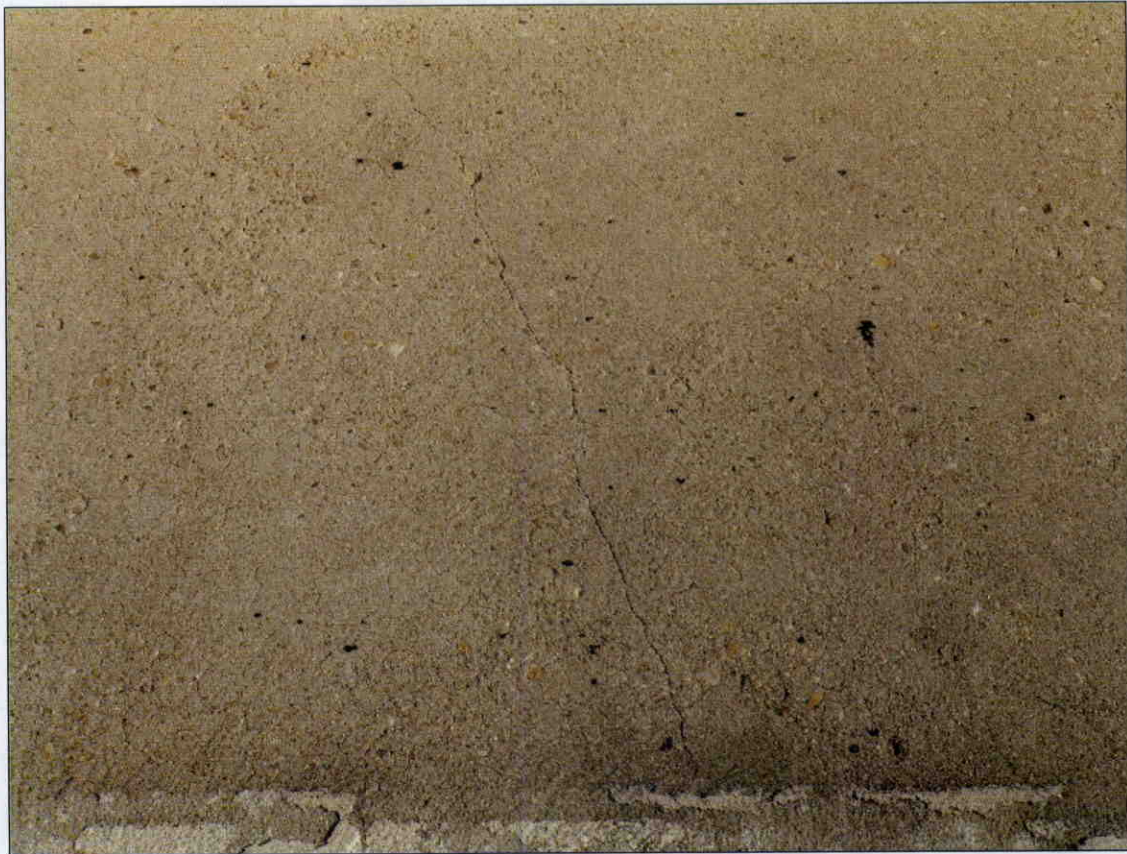
TRANSVERSE HAIRLINE CRACK IN TOP OF DECK AT VARIOUS LOCATIONS THROUGHOUT, SPAN 1 SHOWN
