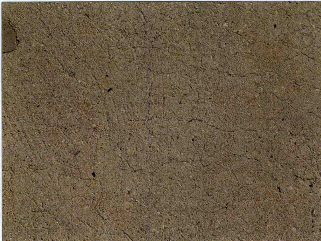
ROUGH AND WORN SURFACE WITH EXPOSED AGGREGATE AND HAIRLINE MAP CRACKING IN TOP OF DECK, SPAN 3 SHOWN, SIMILAR CONDITION THROUGHOUT
