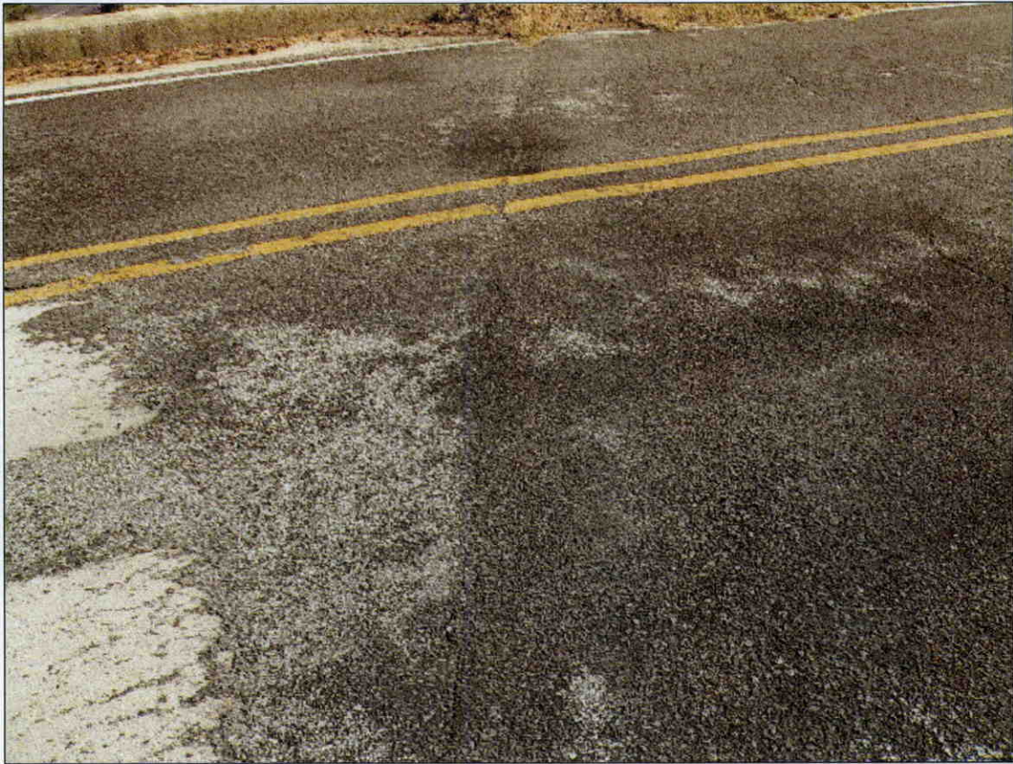
TRANSVERSE CRACK IN ASPHALT WEARING SURFACE ALONG END BENT 2 FILL FACE
