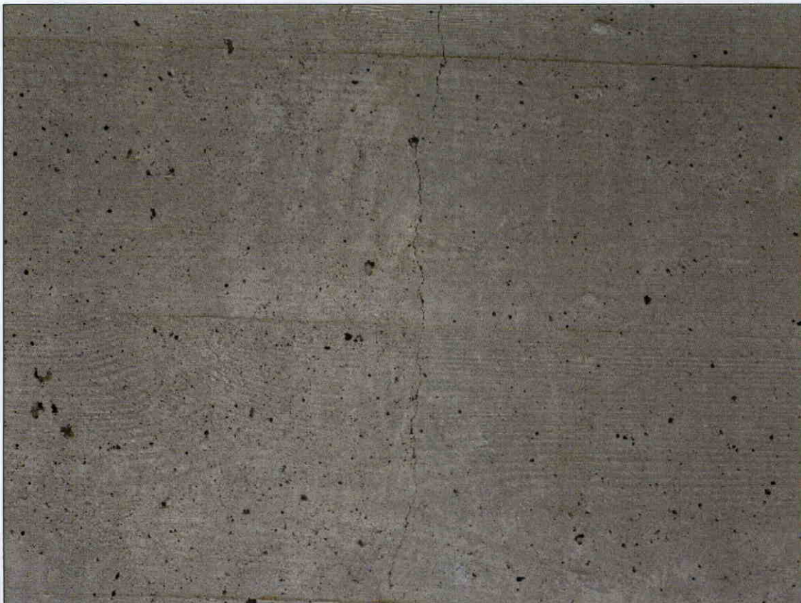
VERTICAL HAIRLINE CRACK IN FACE OF GIRDER 4 IN SPAN 1, SIMILAR CRACKS AT VARIOUS LOCATIONS THROUGHOUT
