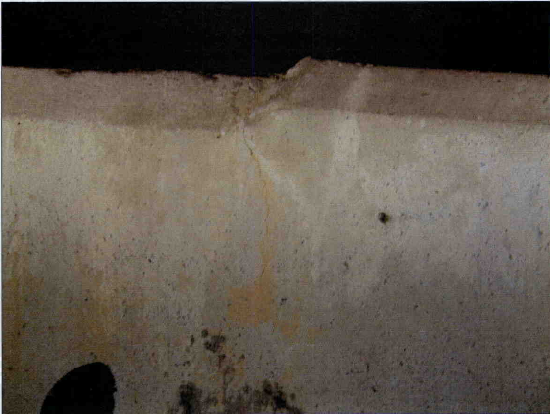
VERTICAL HAIRLINE CRACK IN FACE OF END BENT 1 CAP AT STEP, SIMILAR CRACKS AT END BENT 2
