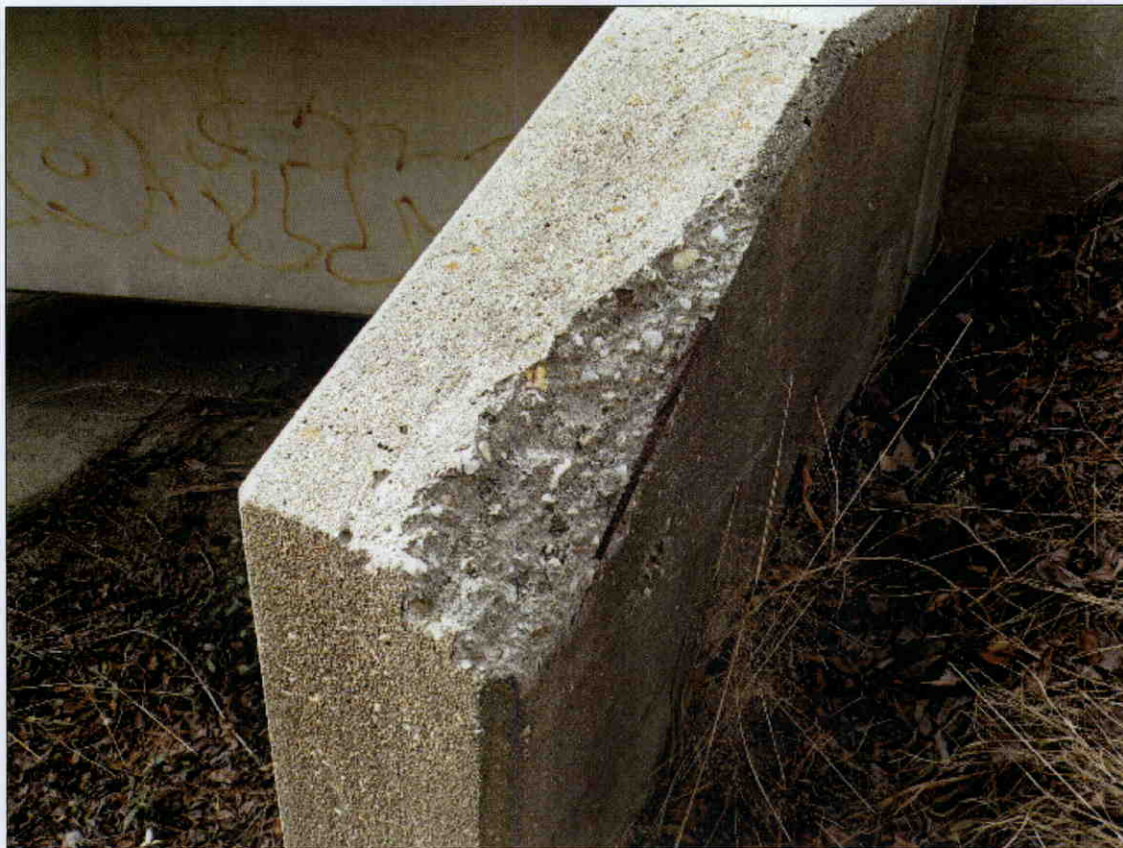
5 IN X 19 IN X 3 IN DEEP SPALL WITH EXPOSED REBAR IN NORTHWEST WINGWALL
