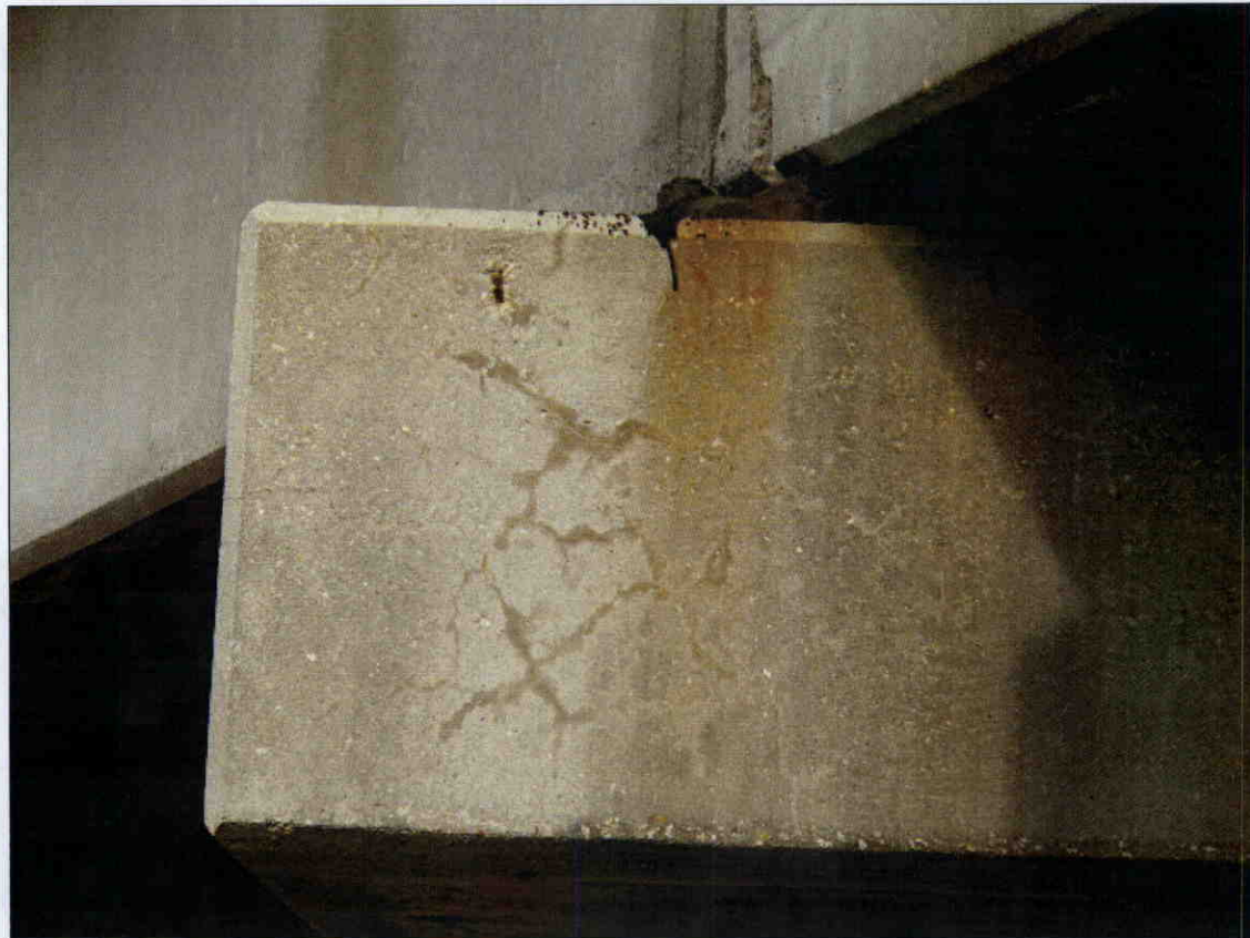
HAIRLINE MAP CRACKING WITH EFFLORESCENCE IN FACE OF BENT 2 CAP, SPAN 3 SIDE UNDER GIRDER 4
