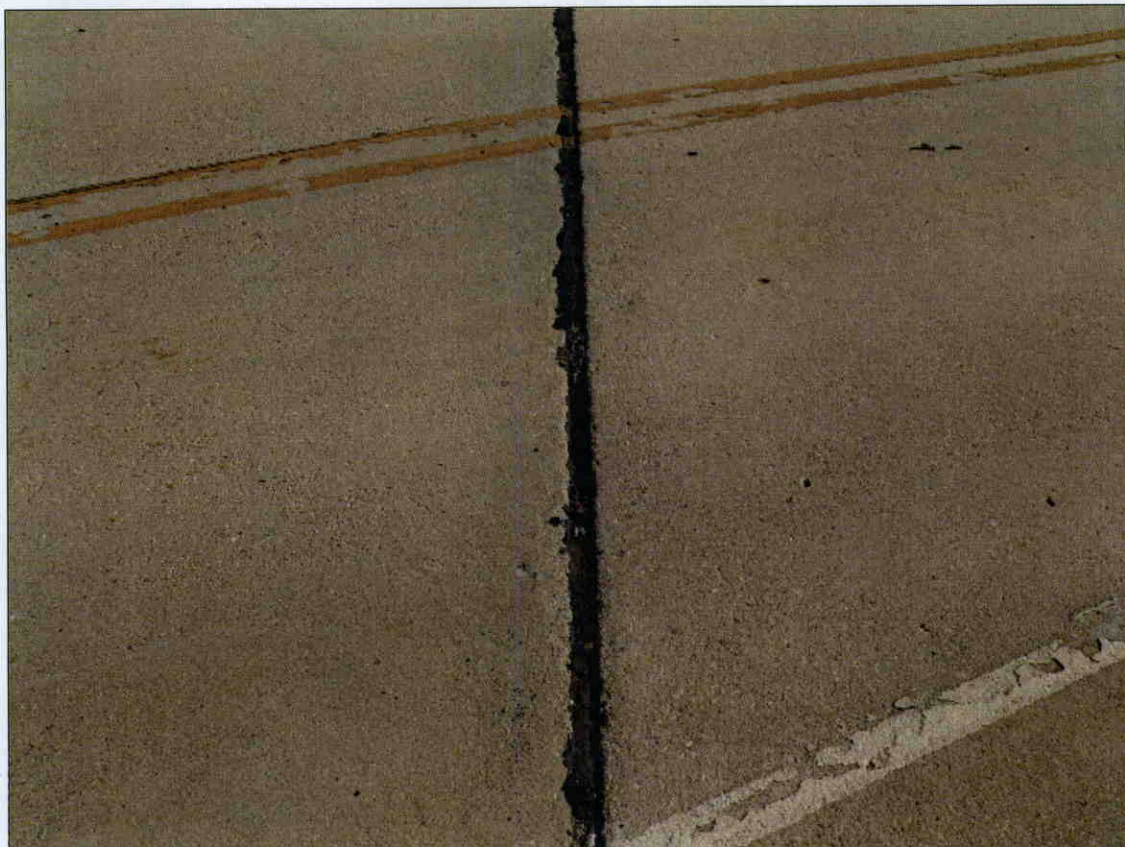
DRIED AND MISSING JOINT MATERIAL AND JOINT SEALER ALONG DECK EXPANSION JOINT AT BENT 1, SIMILAR CONDITION AT DECK EXPANSION JOINT AT BENTS 2 AND 3
