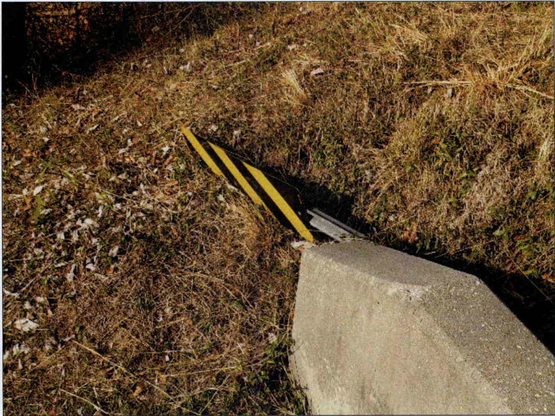
DAMAGED DELINEATOR AT SOUTHWEST CORNER
