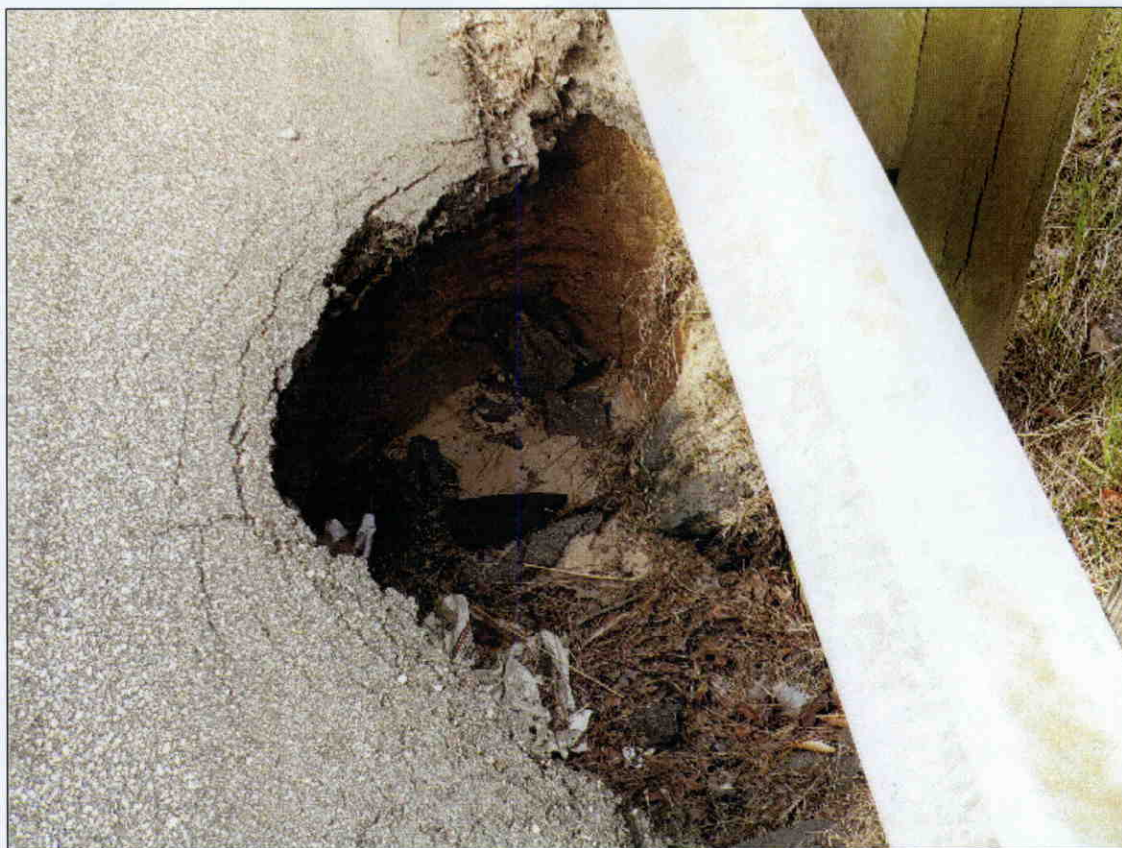
5 FT X 4.5 FT X 2 FT DEEP AREA OF SHOULDER EROSION AT GURDRAIL POST APPROACHING BENT 1 ON SBL I 95
