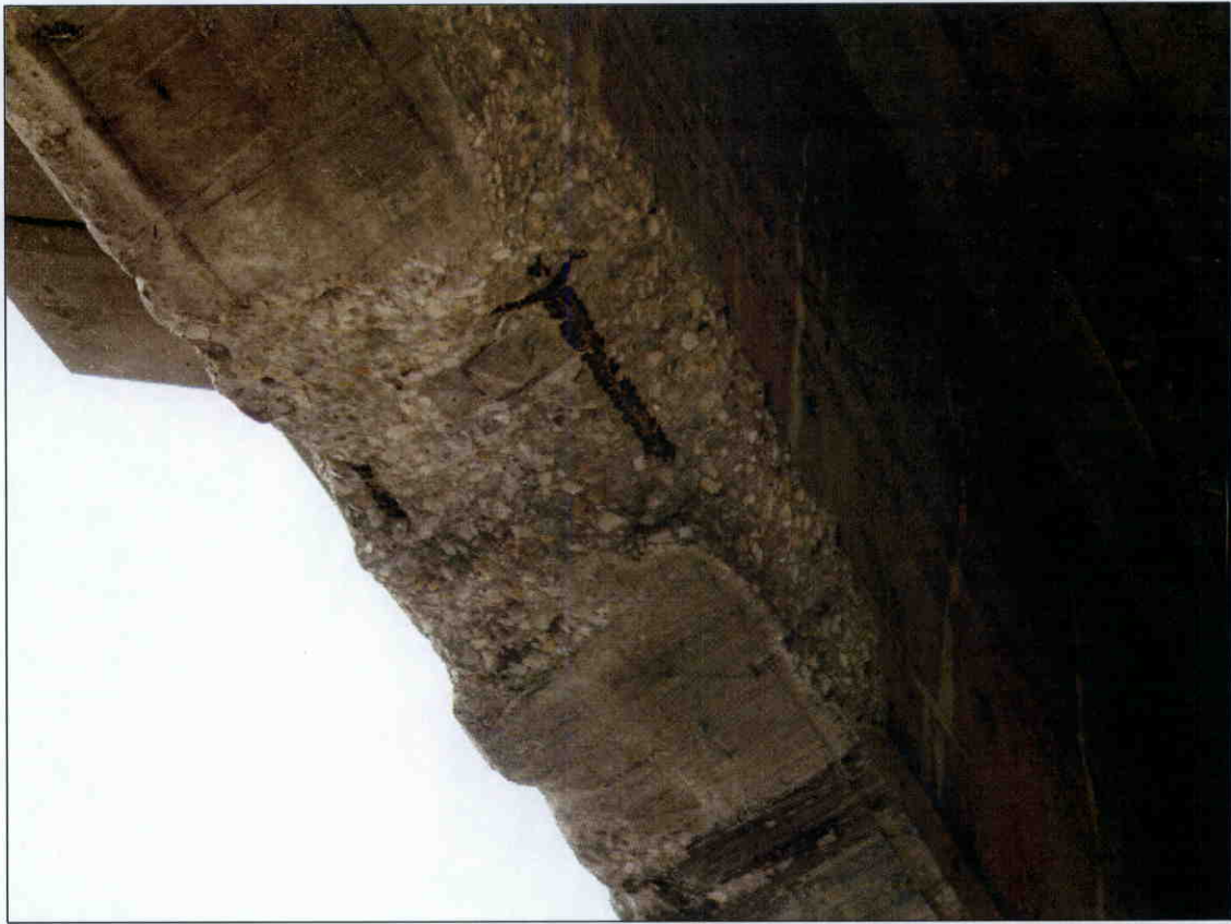
18 IN X 36 IN X 2 IN DEEP SPALL WITH EXPOSED REBAR IN BOTTOM OF GIRDER 4 IN SPAN 3, PROMPT ACTION
