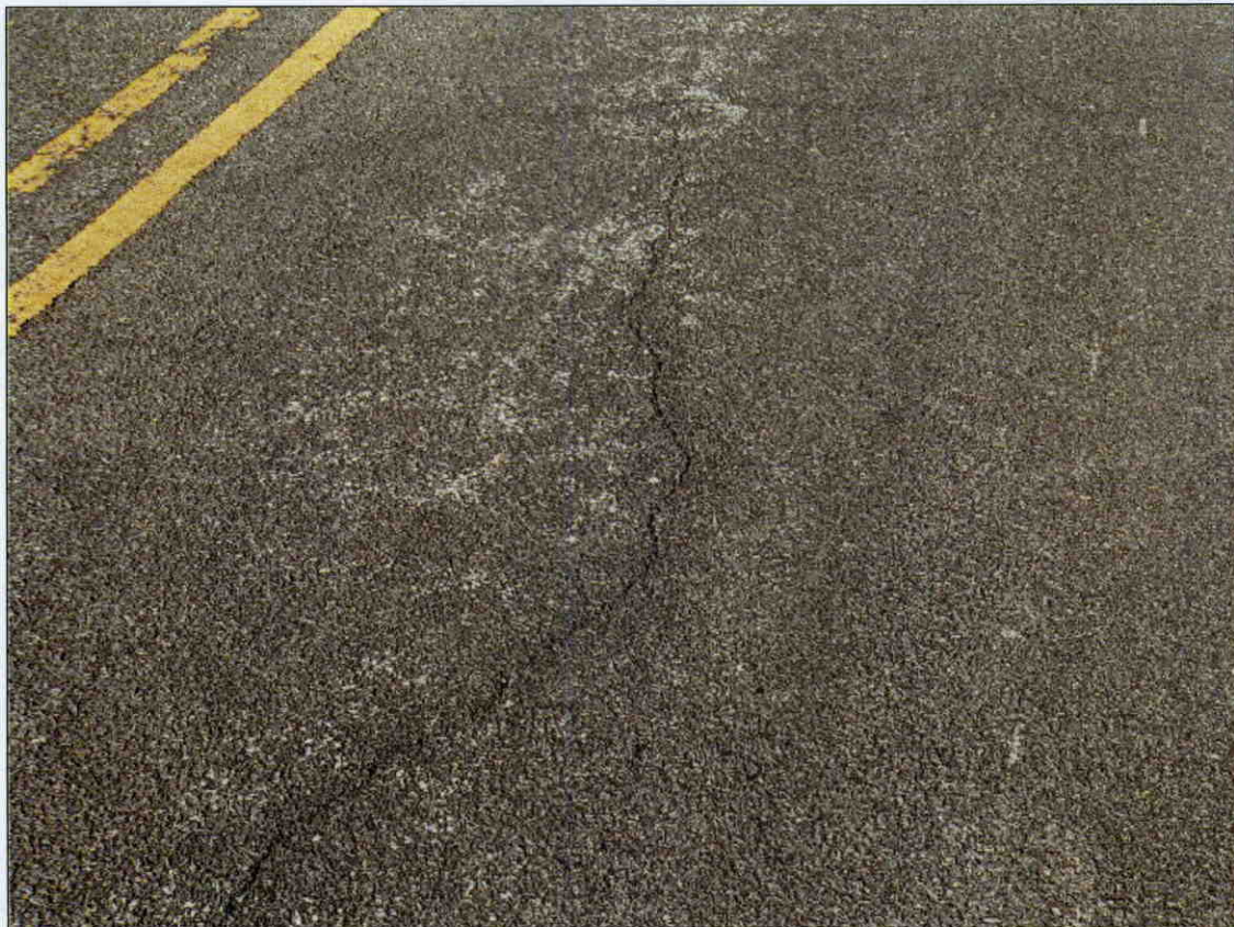
LONGITUDINAL CRACK IN ASPHALT WEARING SURFACE AT EAST APPROACH
