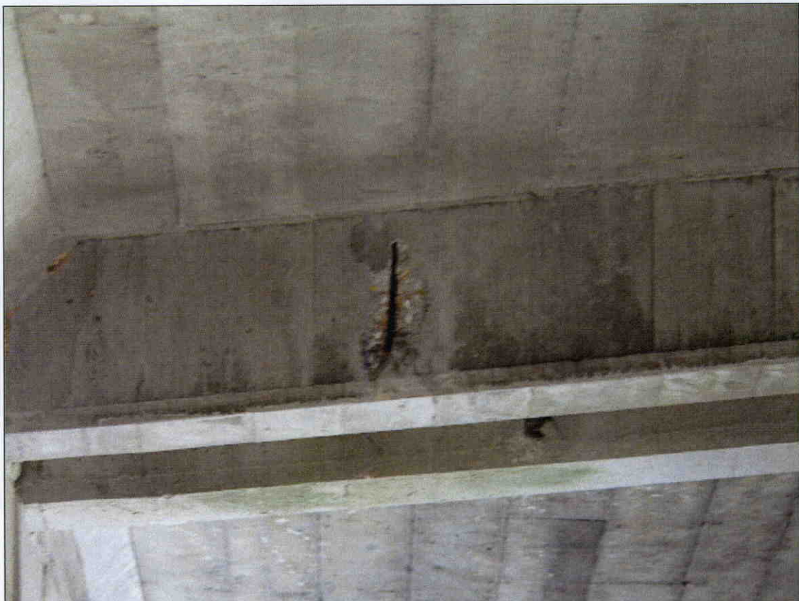
4 IN X 8 IN X 1/2 IN DEEP SPALL WITH EXPOSED REBAR IN END DIAPHRAGM AT BENT 3, BAY 1, SPAN 4 SIDE
