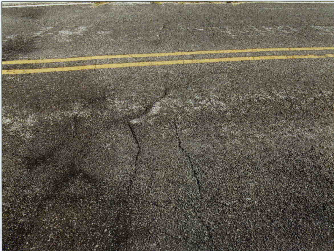
TRANSVERSE CRACKS IN ASPHALT WEARING SURFACE AT EAST APPROACH WITH 1/2 IN OF SETTLEMENT
