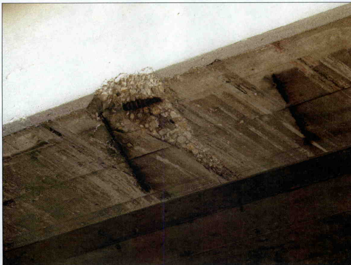
6 IN X 18 IN X 2 IN DEEP SPALL WITH EXPOSED REBAR IN BOTTOM EDGE OF GIRDER 4 IN SPAN 3, PROMPT ACTION
