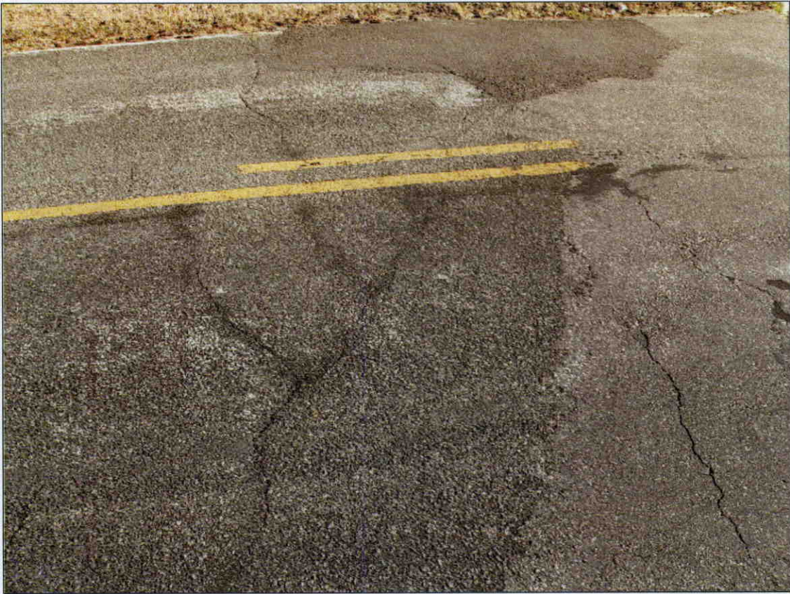
TRANSVERSE CRACKS IN ROUGH AND PATCHED ASPHALT WEARING SURFACE AT WEST APPROACH WITH 1/2 IN OF SETTLEMENT
