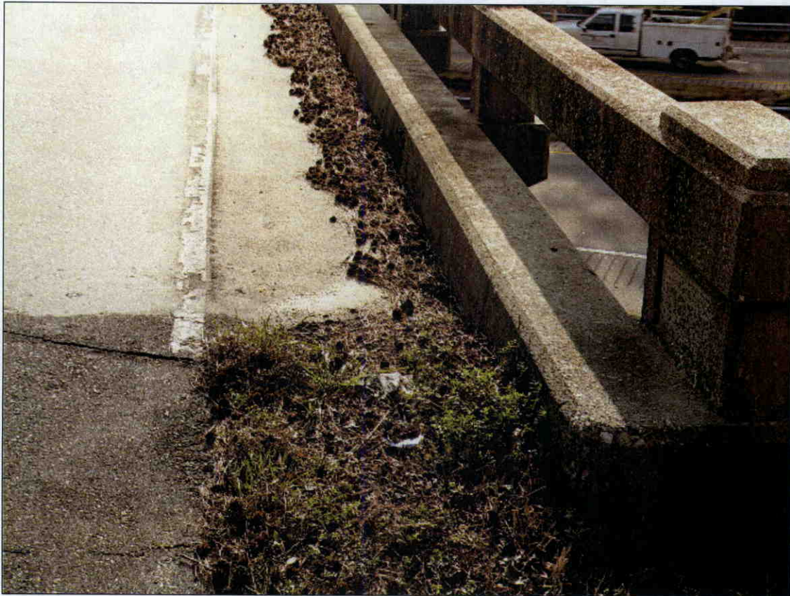
DIRT AND DEBRIS WITH VEGETATION GROWING ALONG SOUTH CURB, SIMILAR CONDITION AT NORTH CURB
