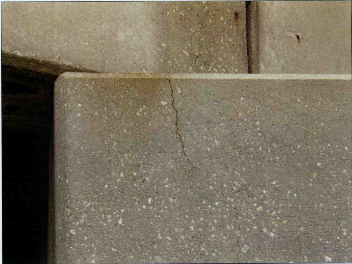
VERTICAL HAIRLINE CRACK IN SOUTH END OF BENT 3 CAP
