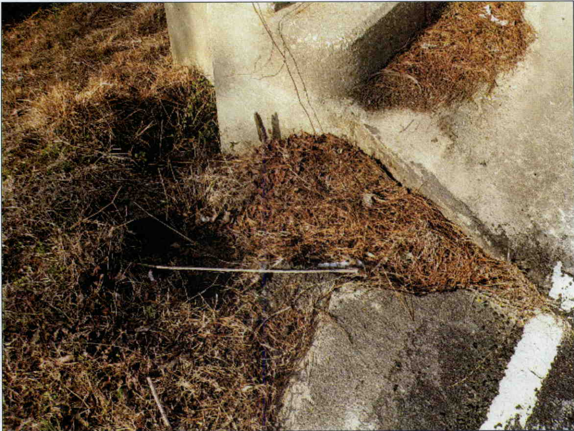
2.5 FT X 10 FT X 2.5 FT DEEP AREA OF SLOPE EROSION AT SOUTHEAST APPROACH
