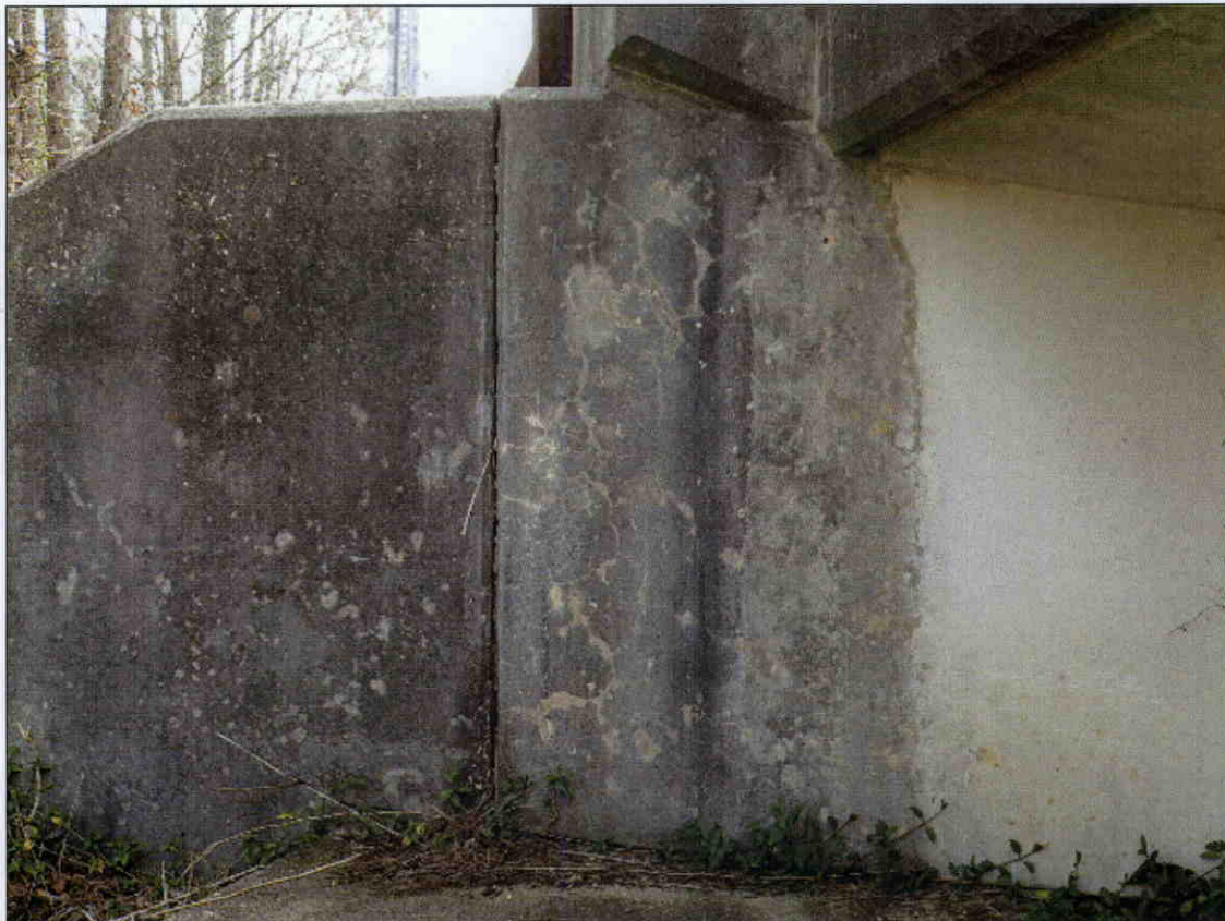
HAIRLINE MAP CRACKING WITH EFFLORESCENCE IN LEFT SIDE OF END BENT 2 CURTAINWALL
