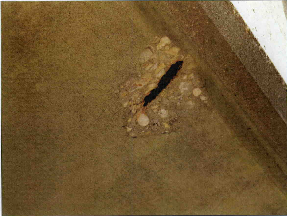
6 IN X 6 IN X 1 IN DEEP SPALL WITH EXPOSED REBAR IN BOTTOM DECK OVERHANG, AT VARIOUS LOCATIONS ALONG SOUTH OVERHANG IN SPAN 4
