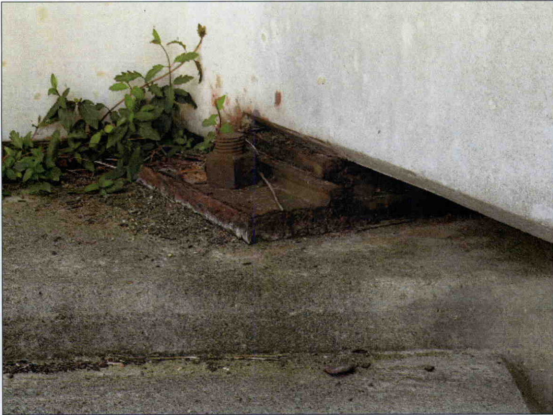
RUST AND DELAMINATION OF BEARING AT GIRDER 1 AT END BENT 2, BEARING AT GIRDER 4 SIMILAR
