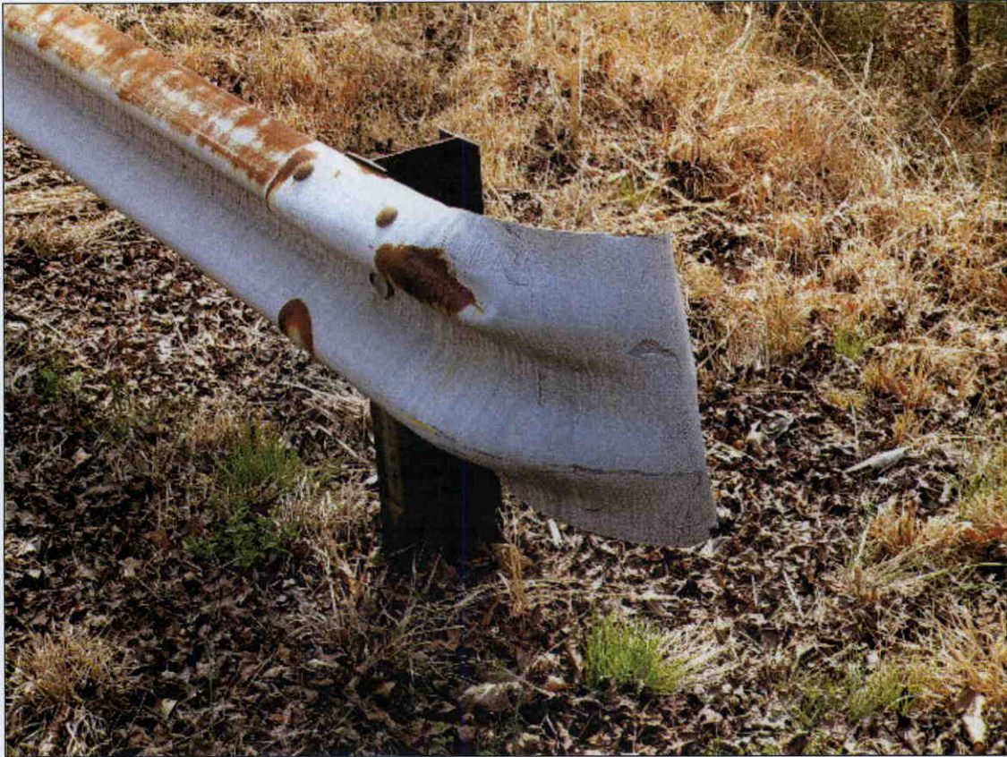
IMPACT DAMAGE TO APPROACH GUARDRAIL END TREATMENT AT SOUTHWEST CORNER
