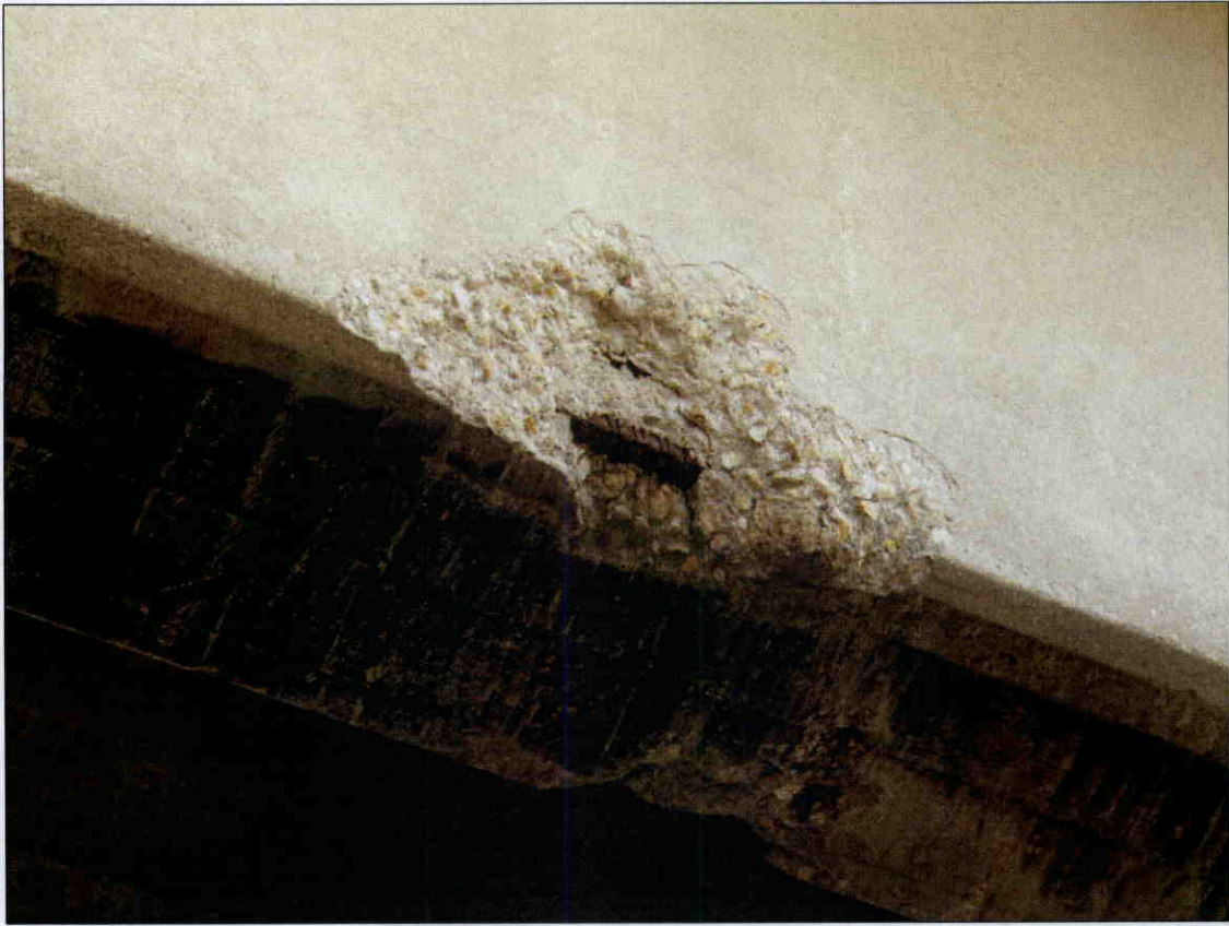
12 IN X 18 IN X 2 IN DEEP SPALL WITH EXPOSED REBAR IN BOTTOM EDGE OF GIRDER 4 IN SPAN 2, PROMPT ACTION
