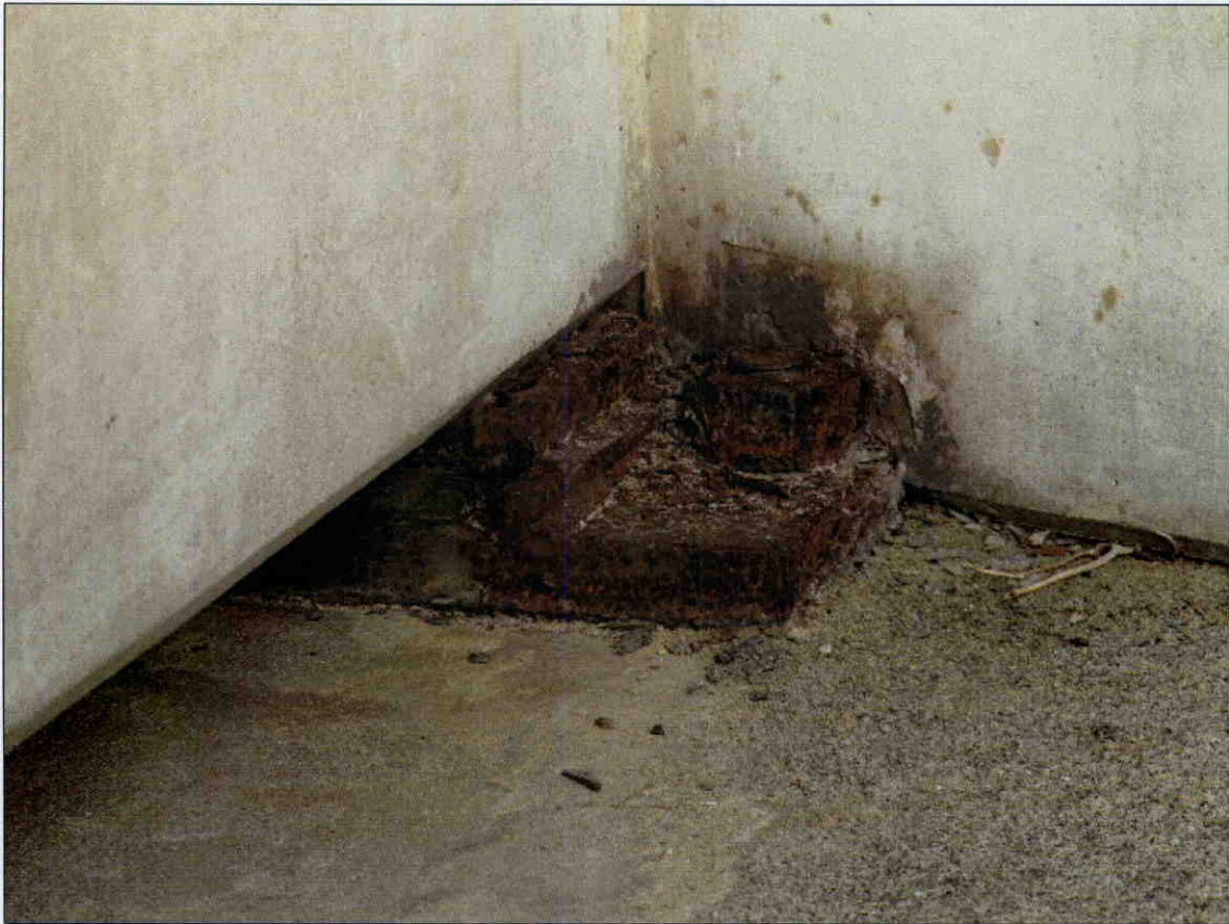
RUST AND DELAMINATION IN BEARING AT GIRDER 1 AT END BENT 1, BEARING AT GIRDER 4 SIMILAR
