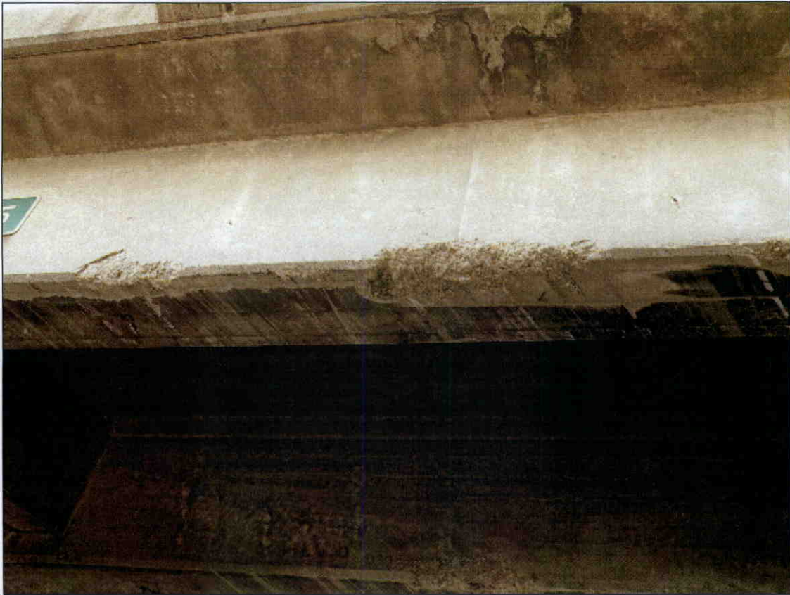
CHIPPING AND SPALLING OF GIRDER 1 DUE TO IMPACT DAMAGE IN SPAN 2, SIMILAR CONDITION IN GIRDERS 2, 3, AND 4
