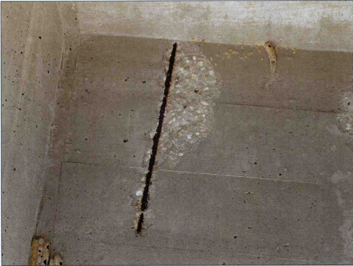
6 IN X 21 IN X 1/2 IN DEEP SPALL WITH EXPOSED REBAR IN FACE OF GIRDER 4 IN SPAN 1, SIMILAR SPALLS IN GIRDERS 1 AND 4 THROUGHOUT SPAN 1
