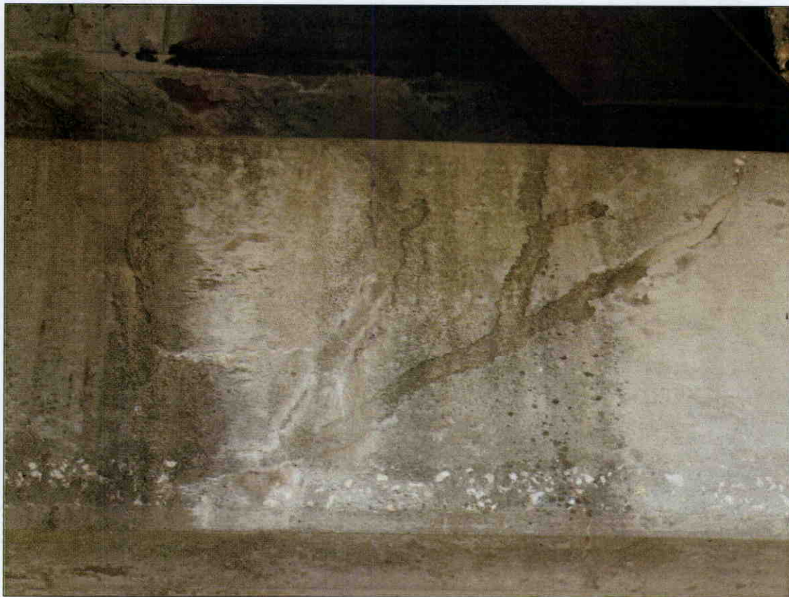
DIAGONAL HAIRLINE CRACK IN FACE OF BENT 1 CAP AT BEAM 2, SPAN 2 SIDE
