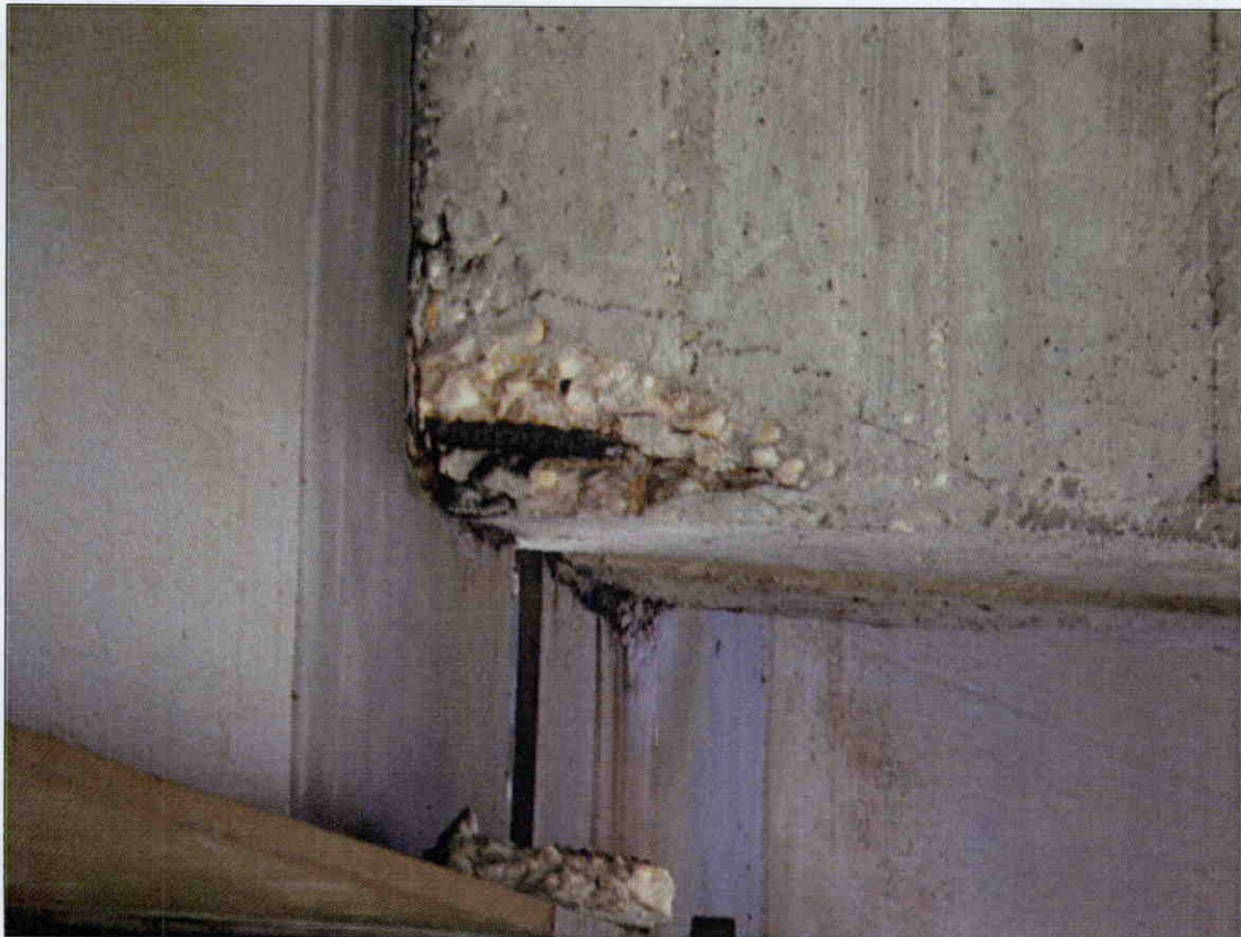
6 IN X 10 IN X 2 IN SPALL WITH EXPOSED REBAR IN BOTTOM OF END DIAPHRAGM AT BENT 3, SPAN 4 SIDE, BAY 2
