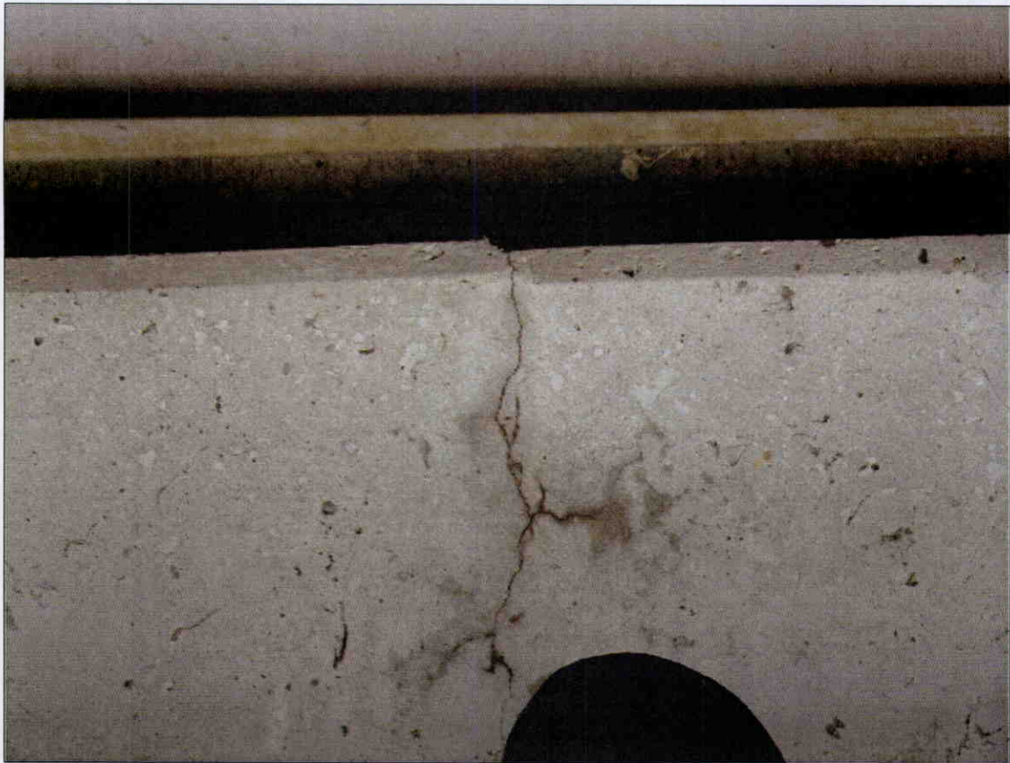
VERTICAL HAIRLINE CRACK IN FACE OF END BENT 2 CAP AT STEP, SIMILAR CRACKS AT STEPS AT END BENTS 1 AND 2.
