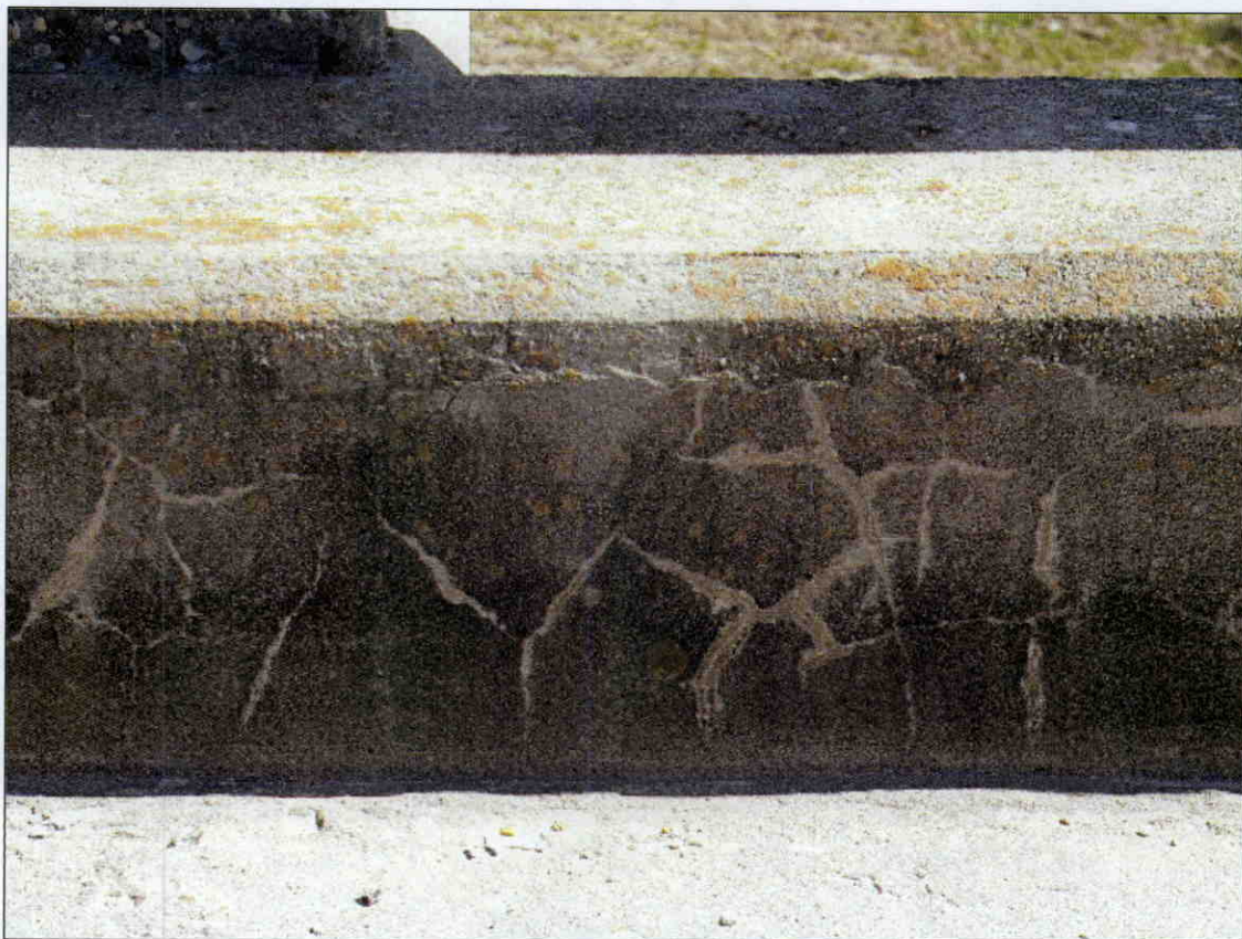
HAIRLINE MAP CRACKING WITH EFFLORESCENCE IN FACE OF CURB AT VARIOUS LOCATIONS THROUGHOUT
