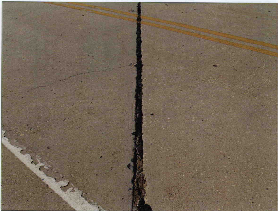
DRIED AND MISSING JOINT SEALER ALONG DECK EXPANSION JOINT AT BENT 1
