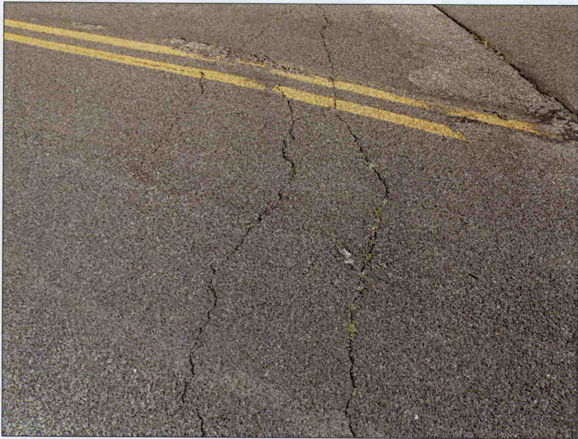
TRANSVERSE CRACKS IN ASPHALT WEARING SURFACE AT WEST APPROACH
