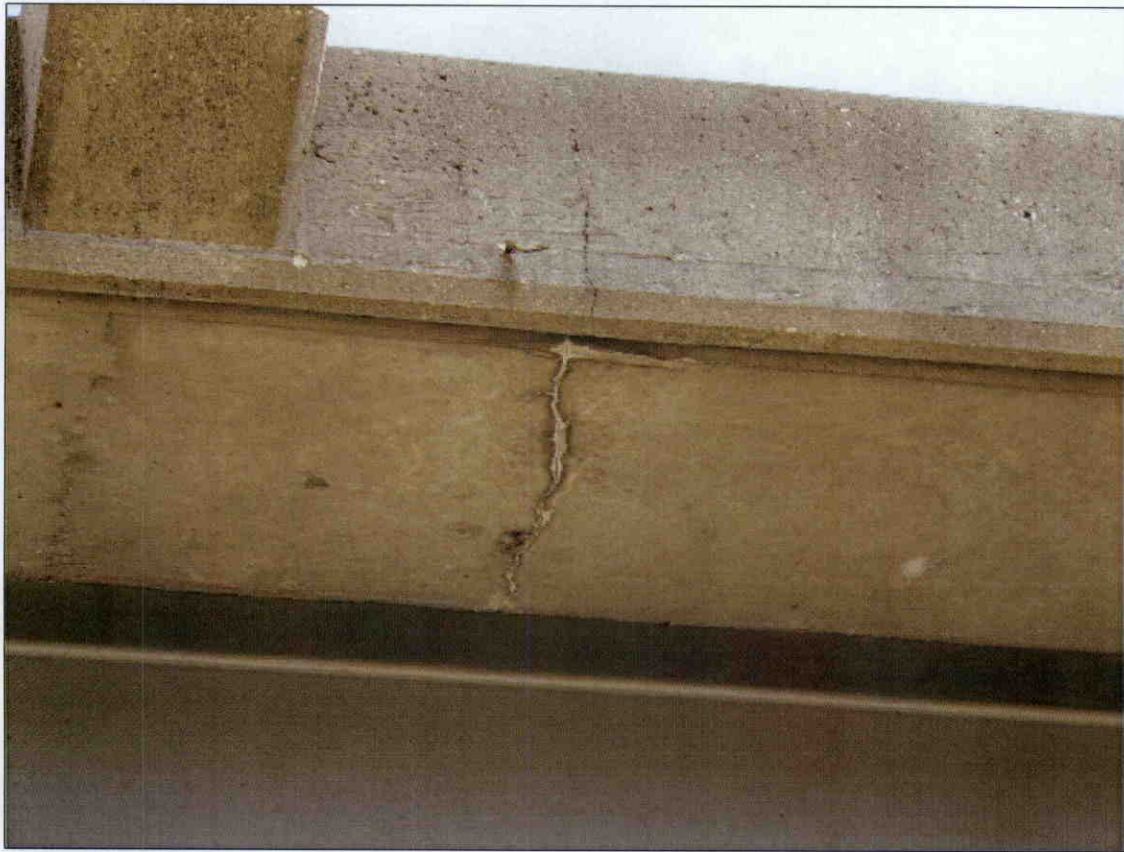
TRANSVERSE HAIRLINE CRACK WITH EFFLORESCENCE IN BOTTOM OF DECK OVERHANG BOTH SIDES AT VARIOUS LOCATIONS
