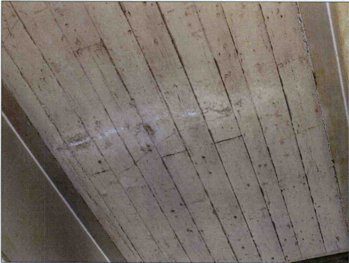
TRANSVERSE HAIRLINE CRACK WITH EFFLORESCENCE IN BOTTOM OF DECK, SPAN 4, SIMILAR CRACKS THROUGHOUT
