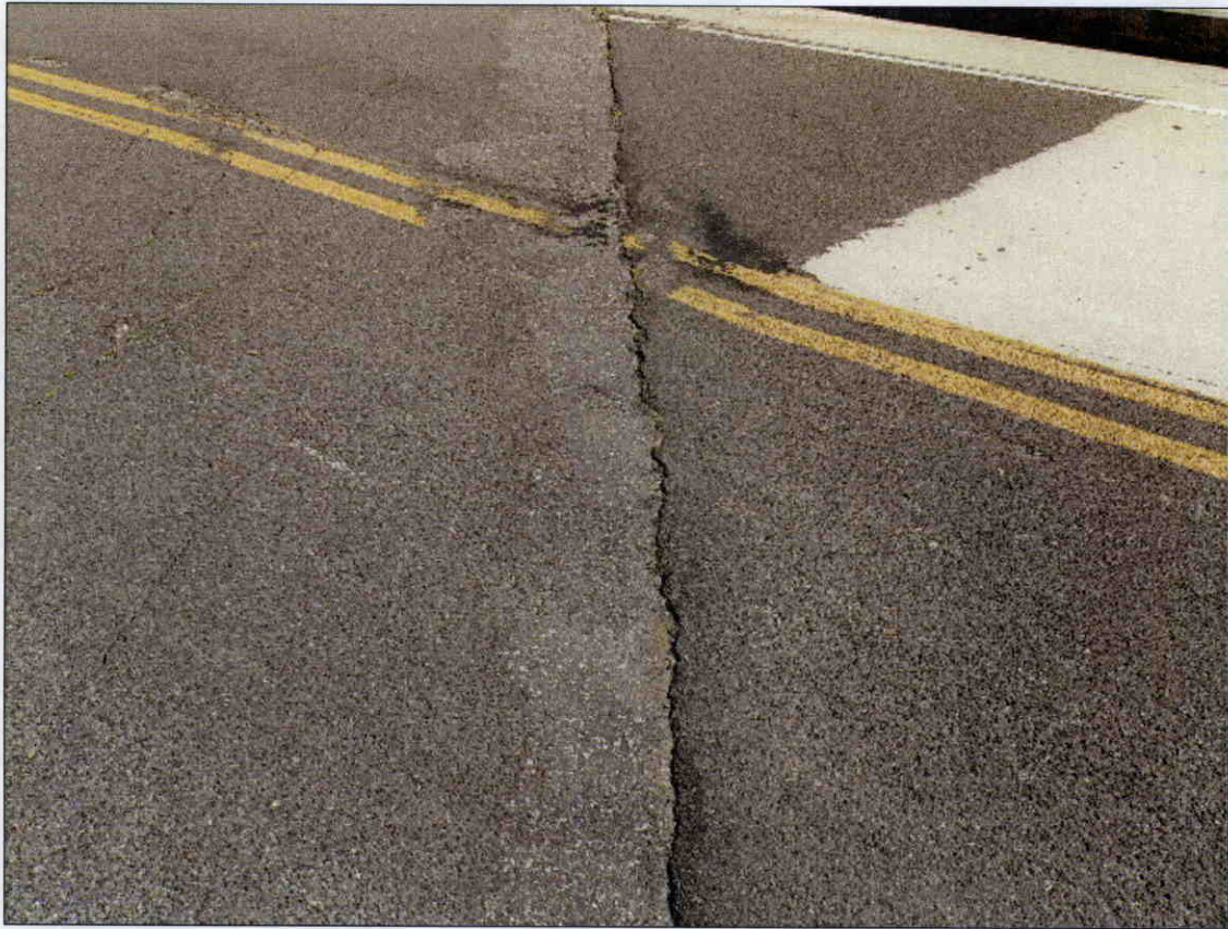
TRANSVERSE CRACK IN ASPHALT WEARING SURFACE ALONG END BENT 1 FILL FACE WITH 1/2 IN OF SETTLEMENT
