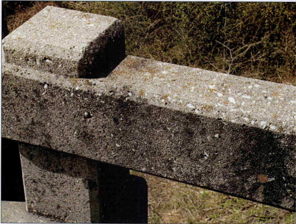
WEATHERING AND SCALING OF BRIDGE RAIL WITH EXPOSED AGGREGATE
