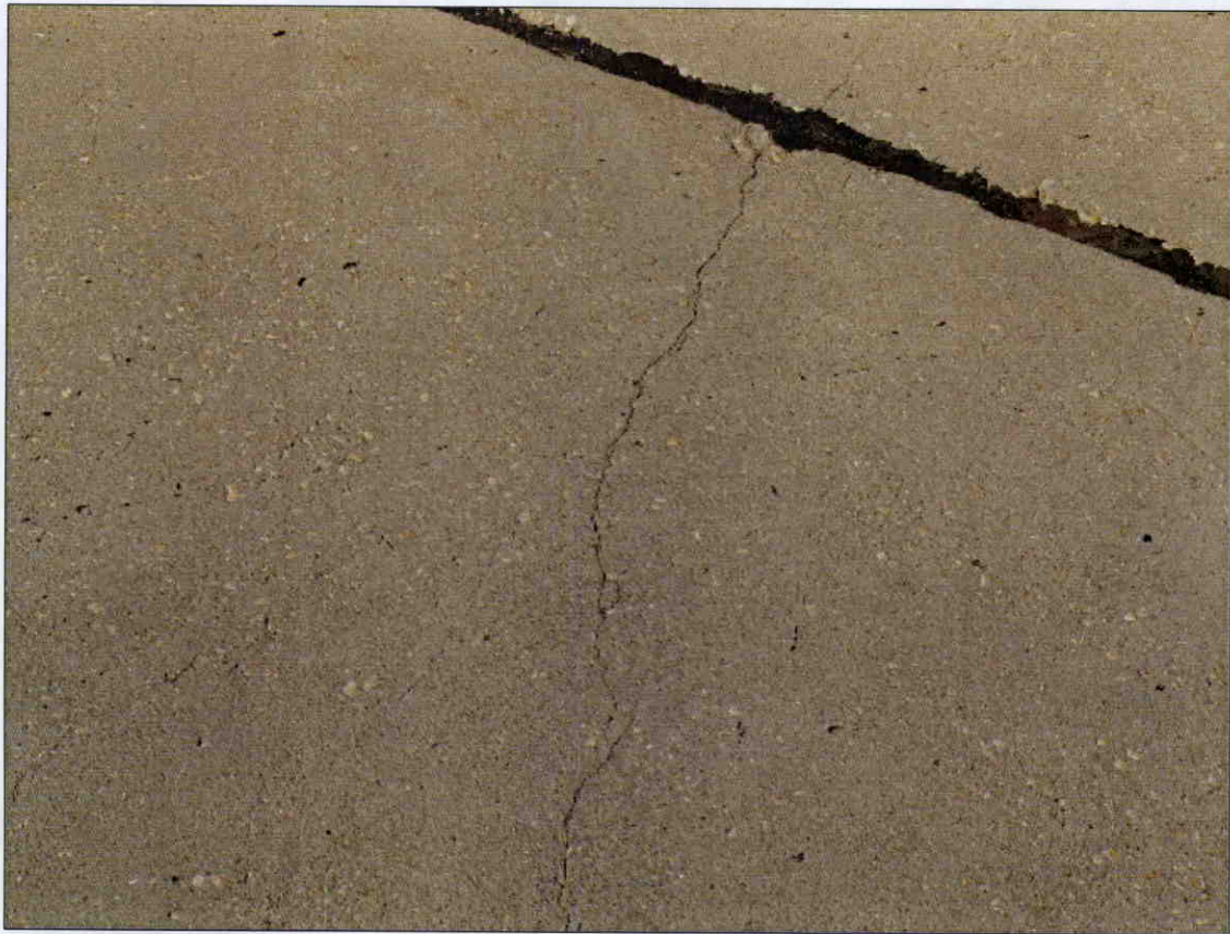
HAIRLINE TO 1/16 IN CRACK IN TOP OF DECK, EXTENDING 6 FT FROM DECK EXPANSION JOINT AT BENT 1, SIMILAR CRACKS AT ALL DECK EXPANSION JOINTS
