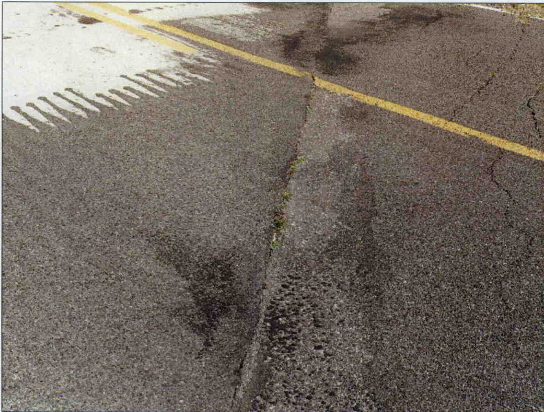
TRANSVERSE CRACK IN ASPHALT WEARING SURFACE ALONG END BENT 2 FILL FACE WITH 1/2 IN OF SETTLEMENT
