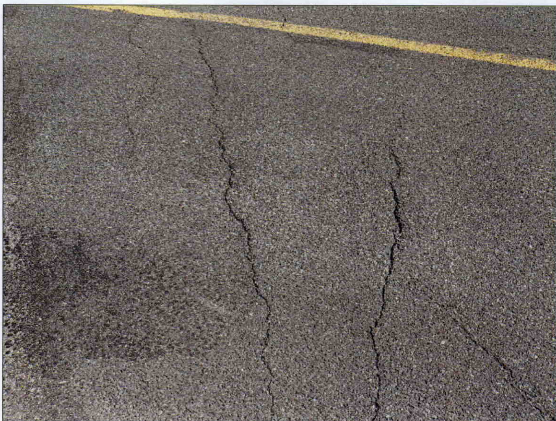
TRANSVERSE CRACKS IN ASPHALT WEARING SURFACE AT EAST APPROACH
