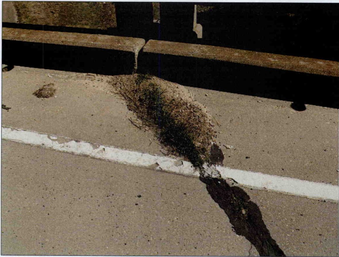
DIRT AND DEBRIS WITH VEGETATION GROWING IN SHOULDER AREA OF DECK EXPANSION JOINT AT BENT 3, SIMILAR CONDITION AT ALL DECK EXPANSION JOINTS
