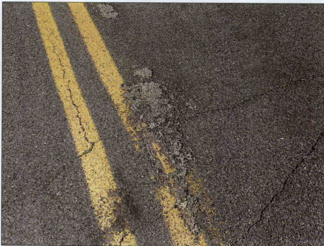
AREAS OF 1/2 IN DEEP SCARED PAVEMENT AT WEST APPROACH
