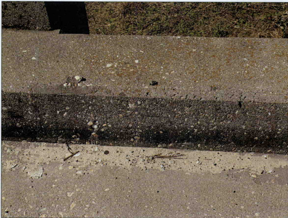
WEATHERING AND SCALING OF CURB WITH EXPOSED AGGREGATE
