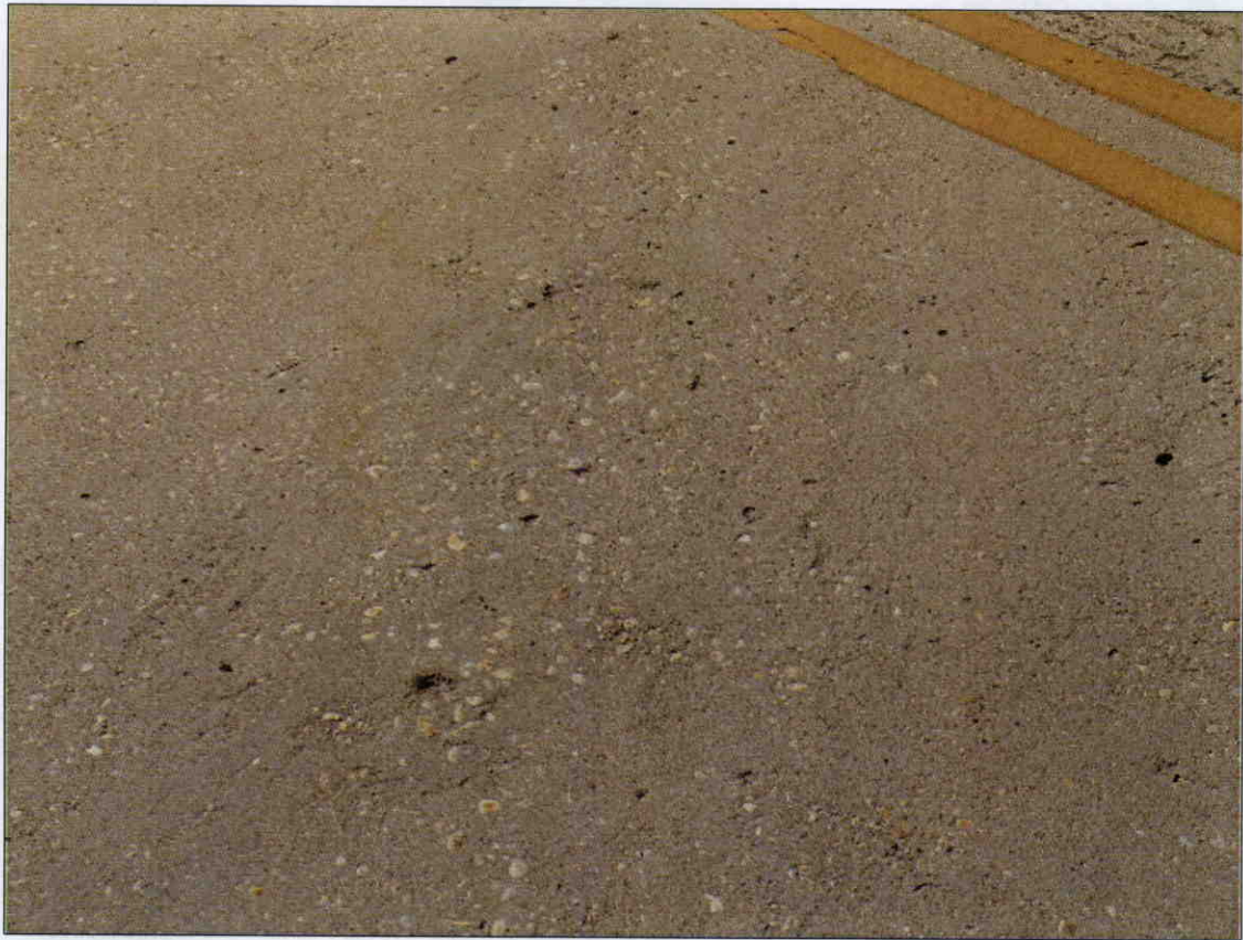
ROUGH AND WORN SURFACE WITH EXPOSED AGGREGATE IN TOP OF DECK, SPAN 1 SHOWN, SIMILAR CONDITION THROUGHOUT
