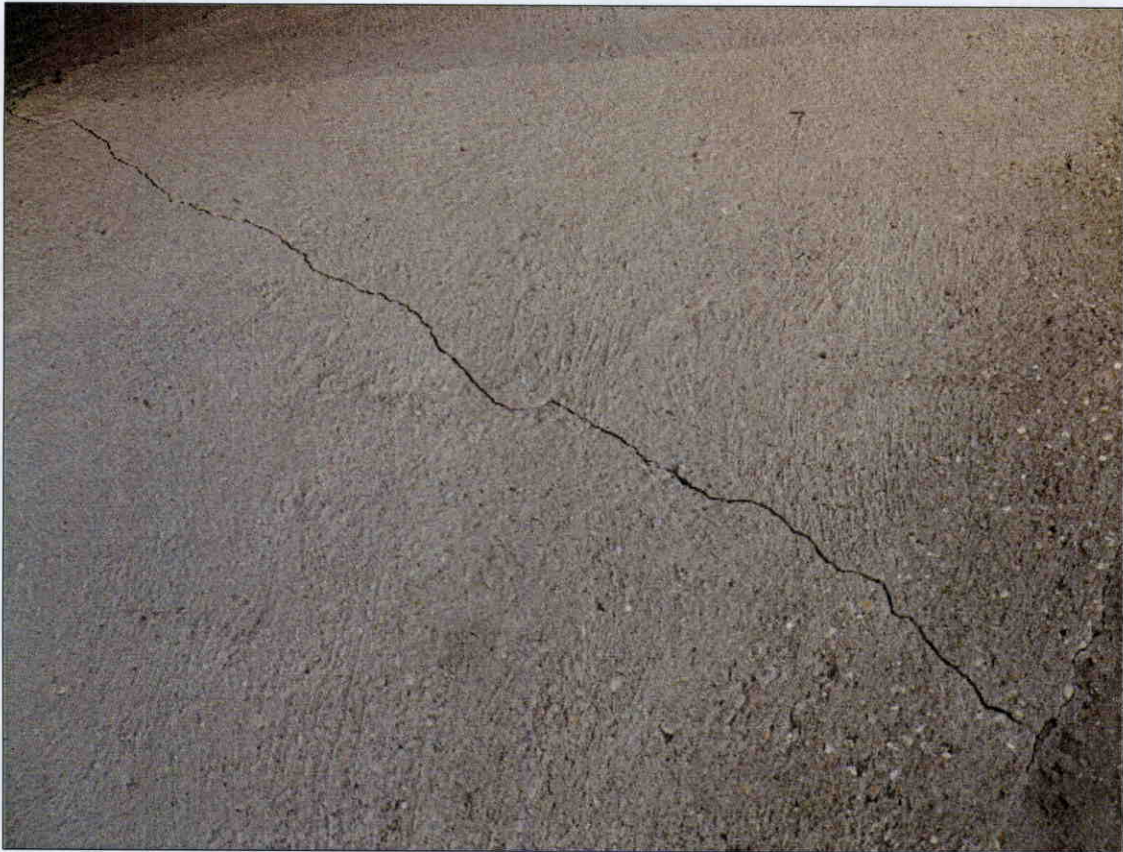
5 FT LONG X 1/8 IN HORIZONTAL CRACK IN SLOPE PROTECTION AT END BENT 2
