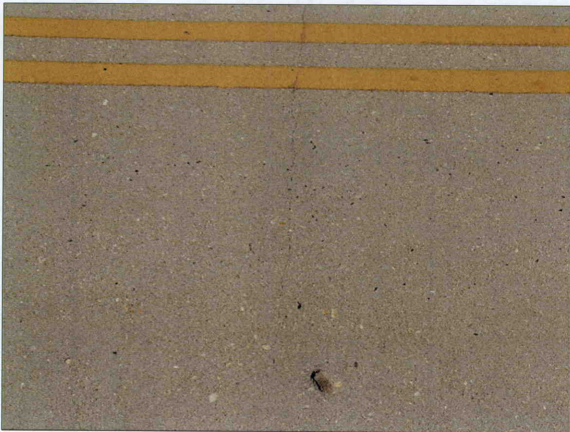
TRANSVERSE HAIRLINE CRACK IN TOP OF DECK, SPAN 2, SIMILAR CRACKS THROUGHOUT
