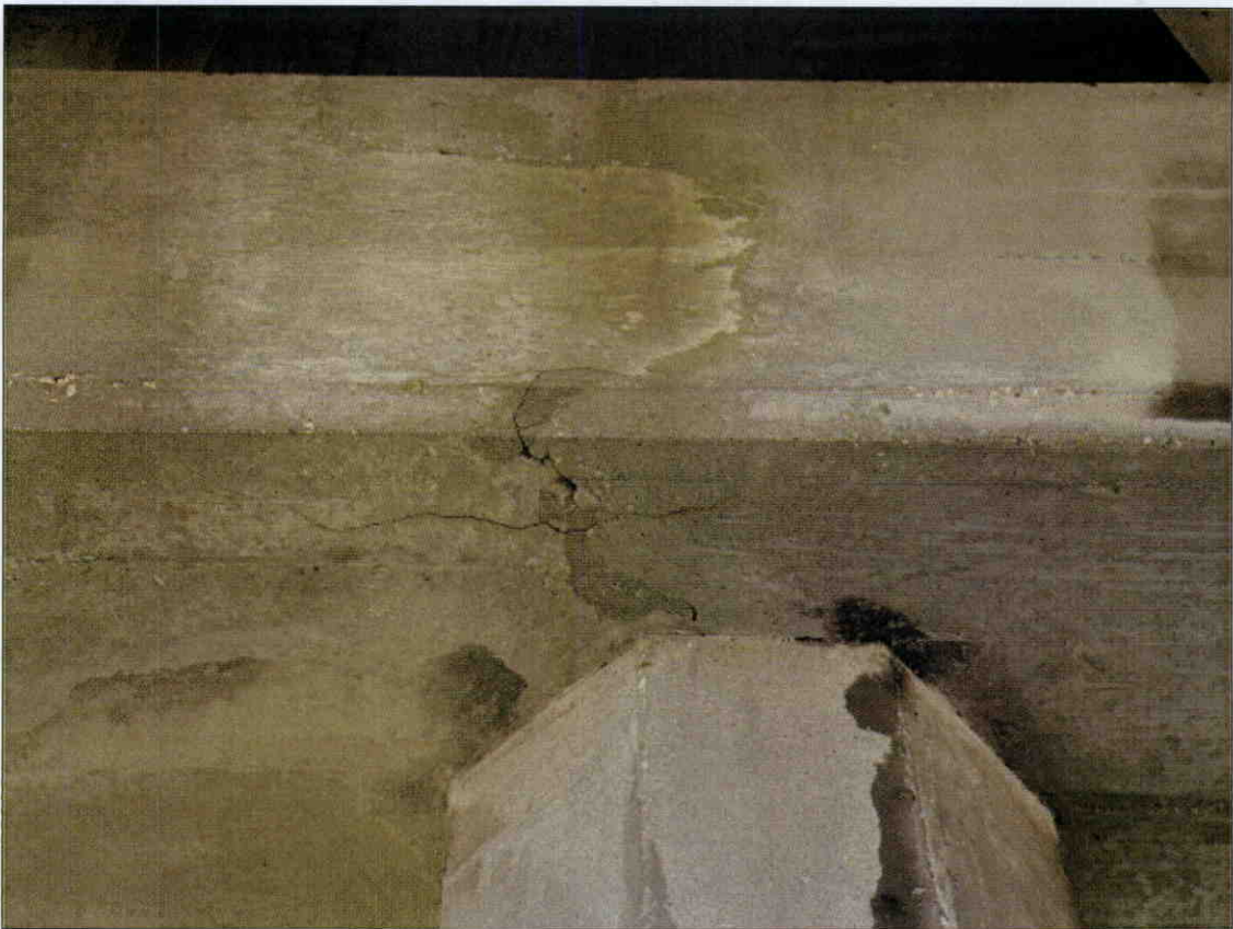
LONGITUDINAL HAIRLINE CRACK IN BOTTOM OF BENT 3 CAP AT PILE 2, SIMILAR CRACK AT BENT 1, PILE 1
