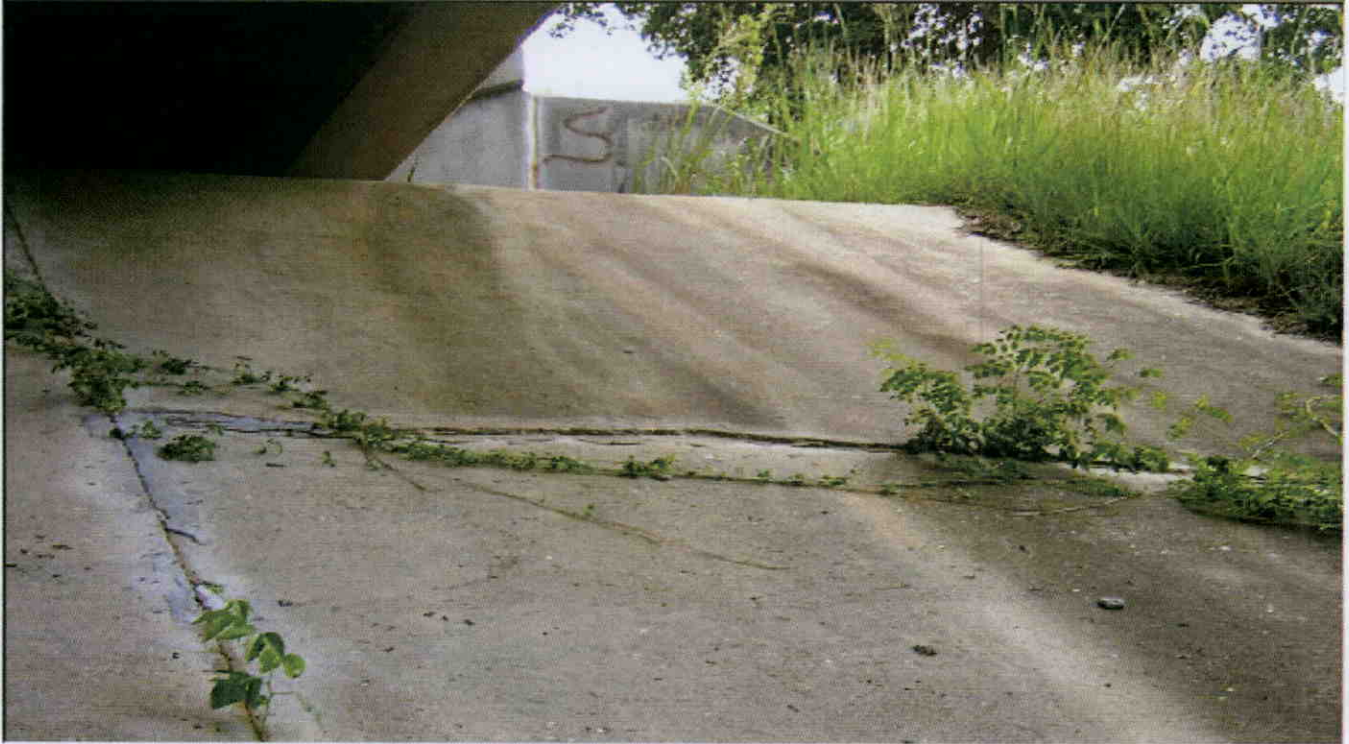
BROKEN AND SETTLED SLOPE SLABS AT RIGHT SIDE, EAST SLOPE
