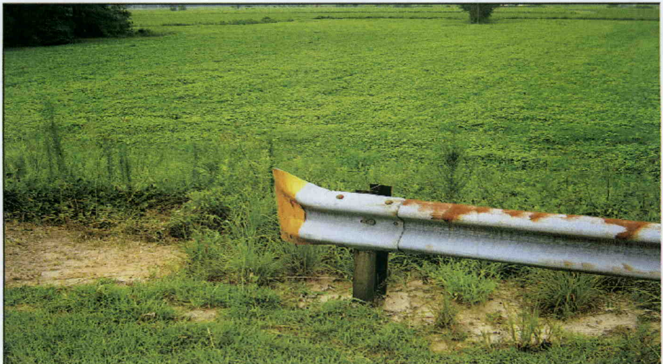
TERMINAL GUARDRAIL END
