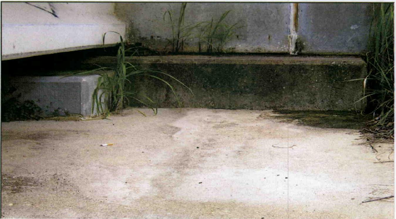
FILL LEAKAGE AT EB2, SIM. AT EB1
