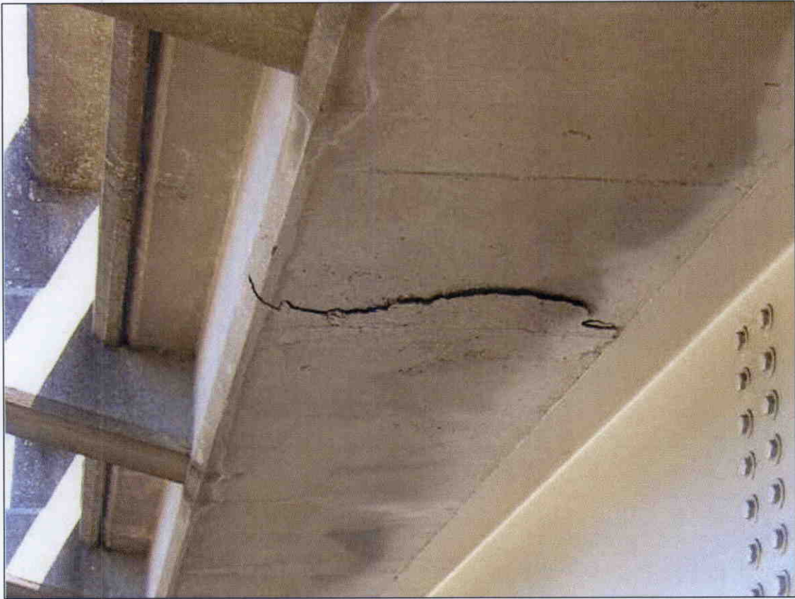
SPALLING IN OVERHANG LEFT SIDE SPAN 1 MIDSPAN.
