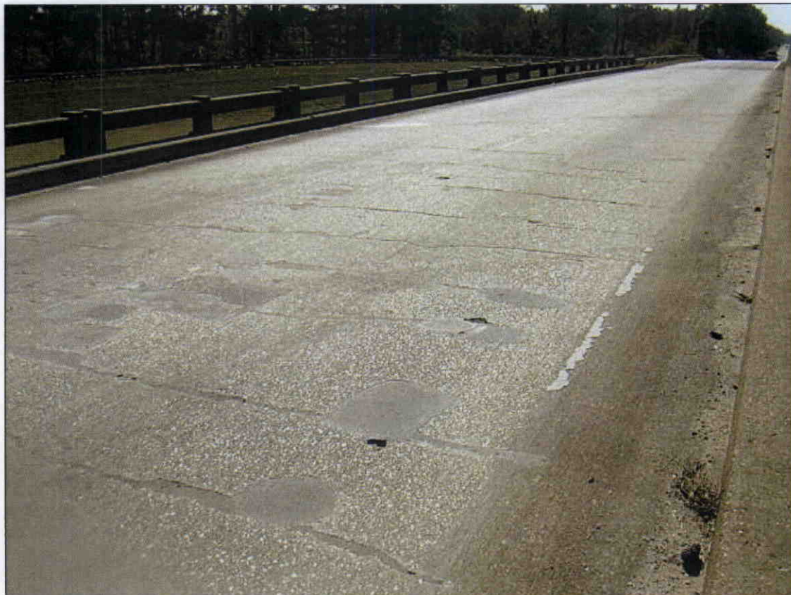
DECK POP OUTS AT SPAN 3.
