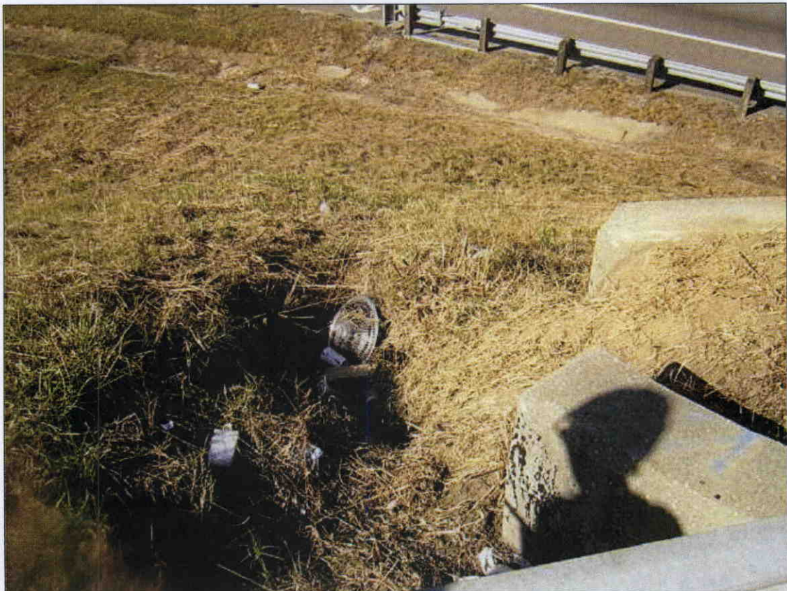
EROSION AT SOUTHWEST CORNER
