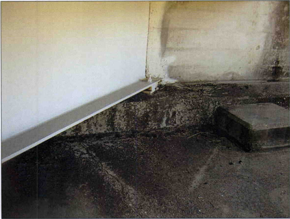
LEAKAGE EVIDENT AT SOUTHWEST CORNER ABUT. 1.
