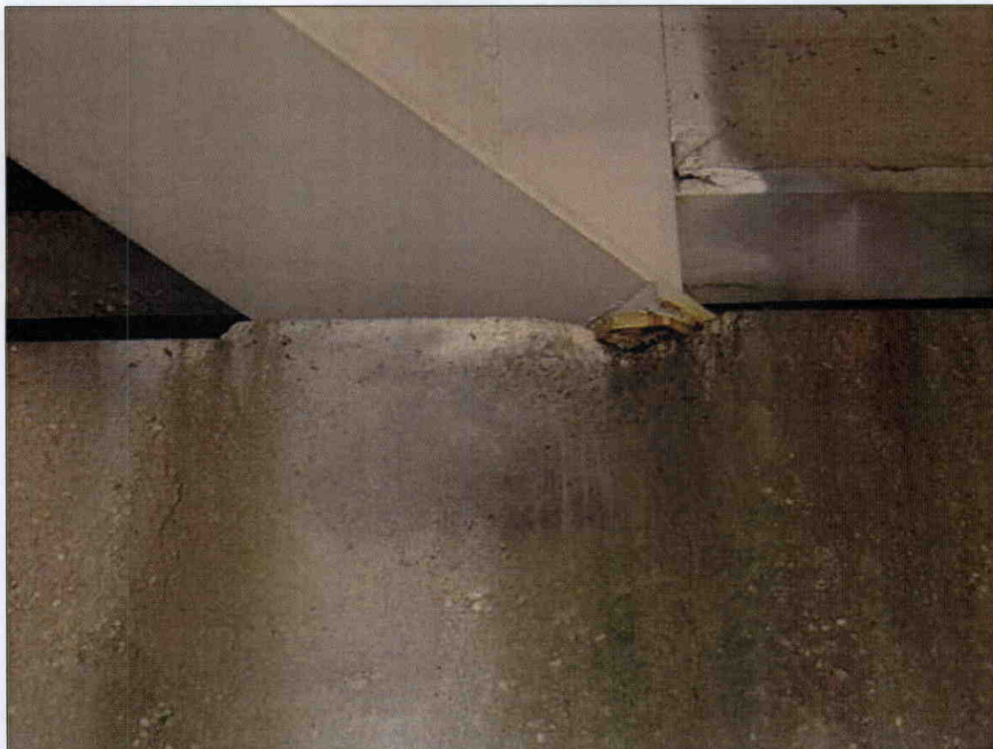
SPALLING IN PIER 2 CAP UNDER BM. 2 SOUTH FACE WITH 75 PERCENT BRG REMAINING.
