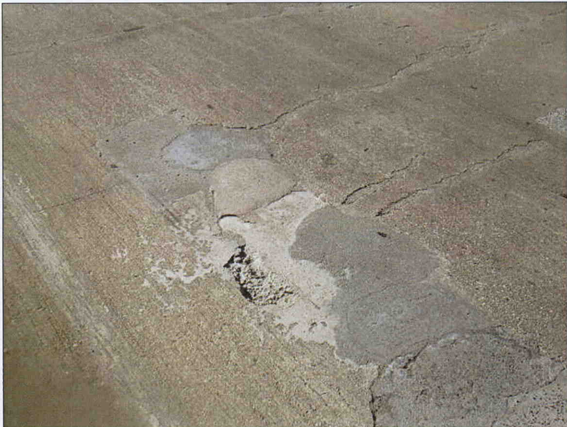
DECK PATCHWORK BEGINNING TO SPALL AND DETERIORATE AT SPAN 3 NBL.
