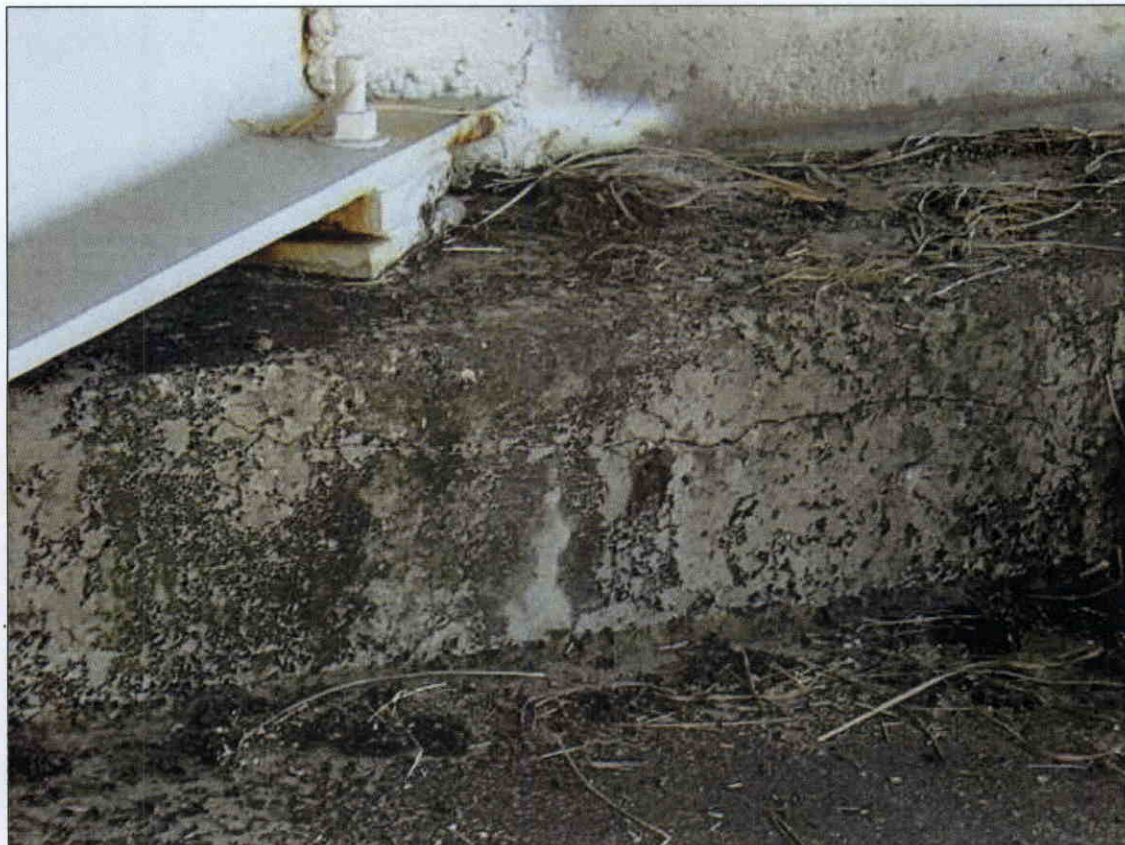
CRACKING AT LEFT END OF ABUT. 1 CAP.
