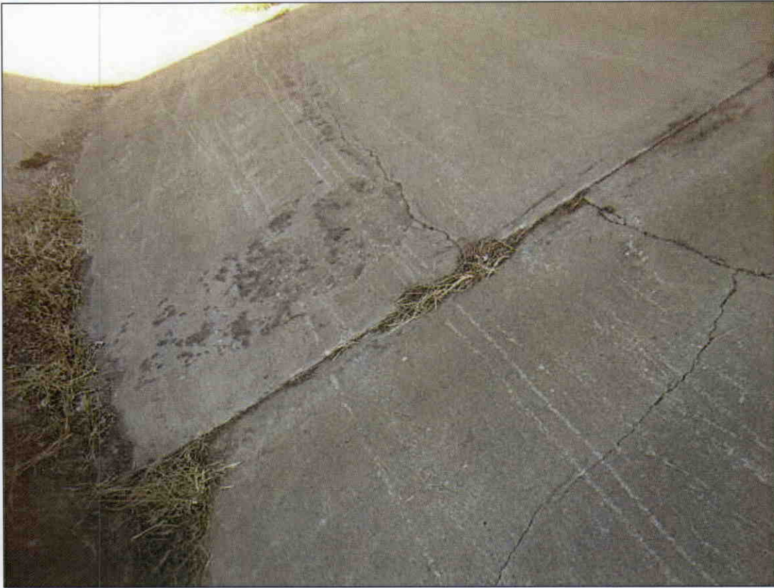
SETTLEMENT 1 INCH AT SOUTH SLOPE SLABS
