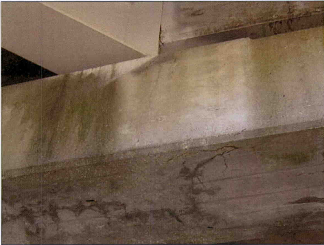
CRACKING IN BOTTOM FACE PIER 2 CAP BETWEEN COLS. 1 AND 2.
