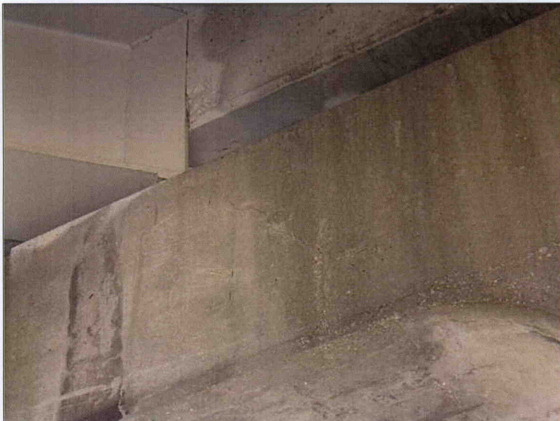
DIAGONAL CRACKING AT PIER 2 CAP UNDER BM.2 ON NORTH FACE. SOUTH FACE SIM.
