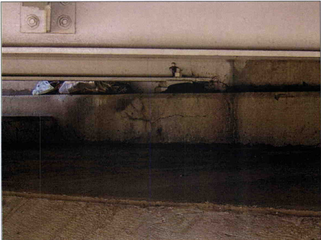
CRACKING AT ABUT. 1 CAP UNDER BM. 4.
