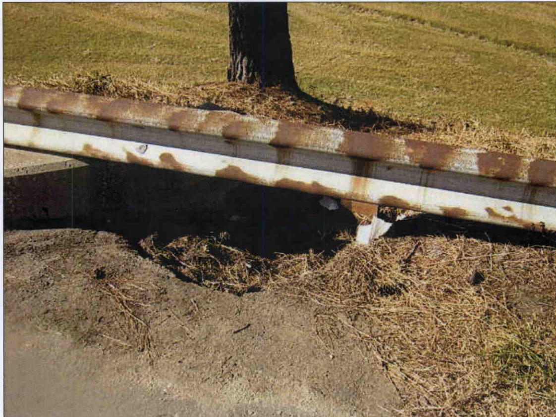
EROSION AT NORTHWEST CORNER
