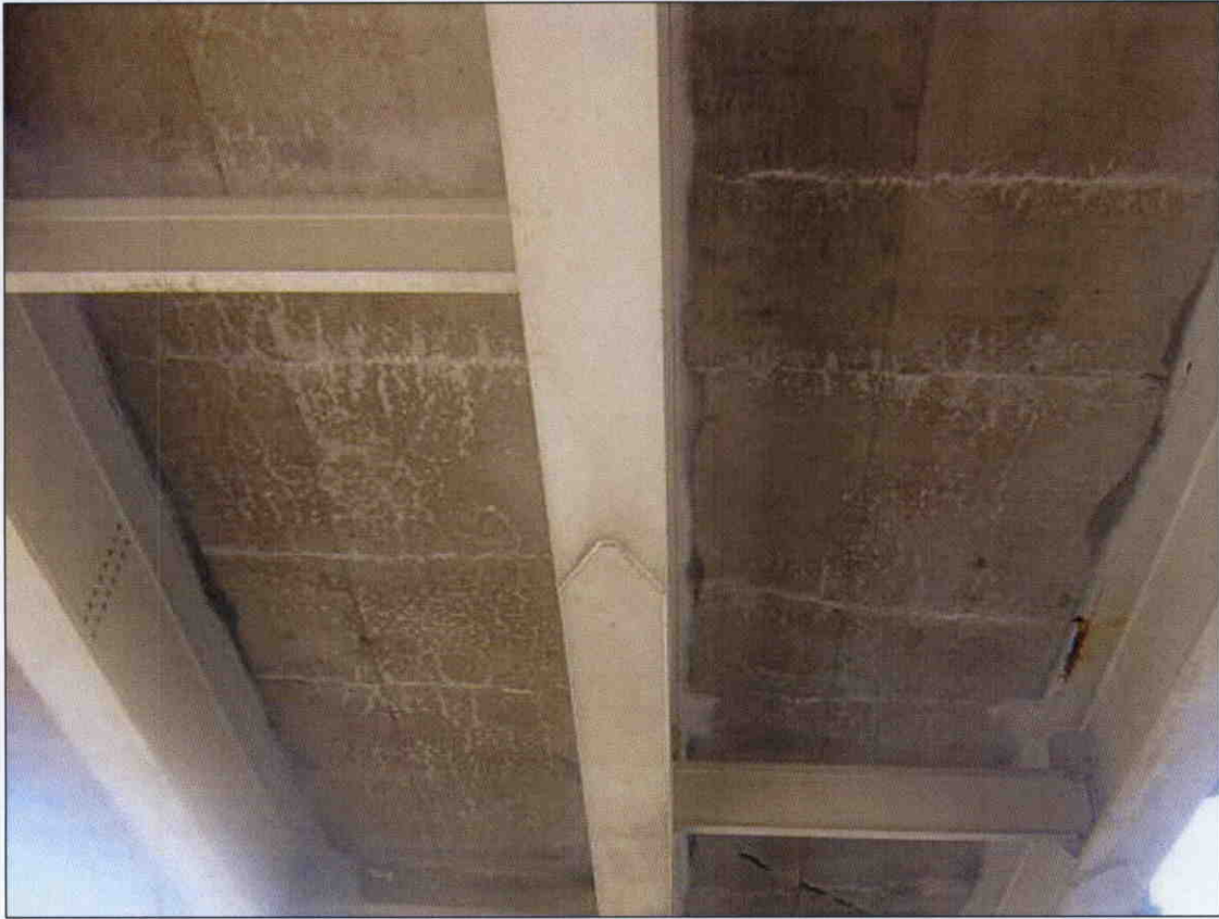
TRANSVERSE CRACKING WITH EFFLO AT EACH SPAN. PHOTO AT SPAN 3
