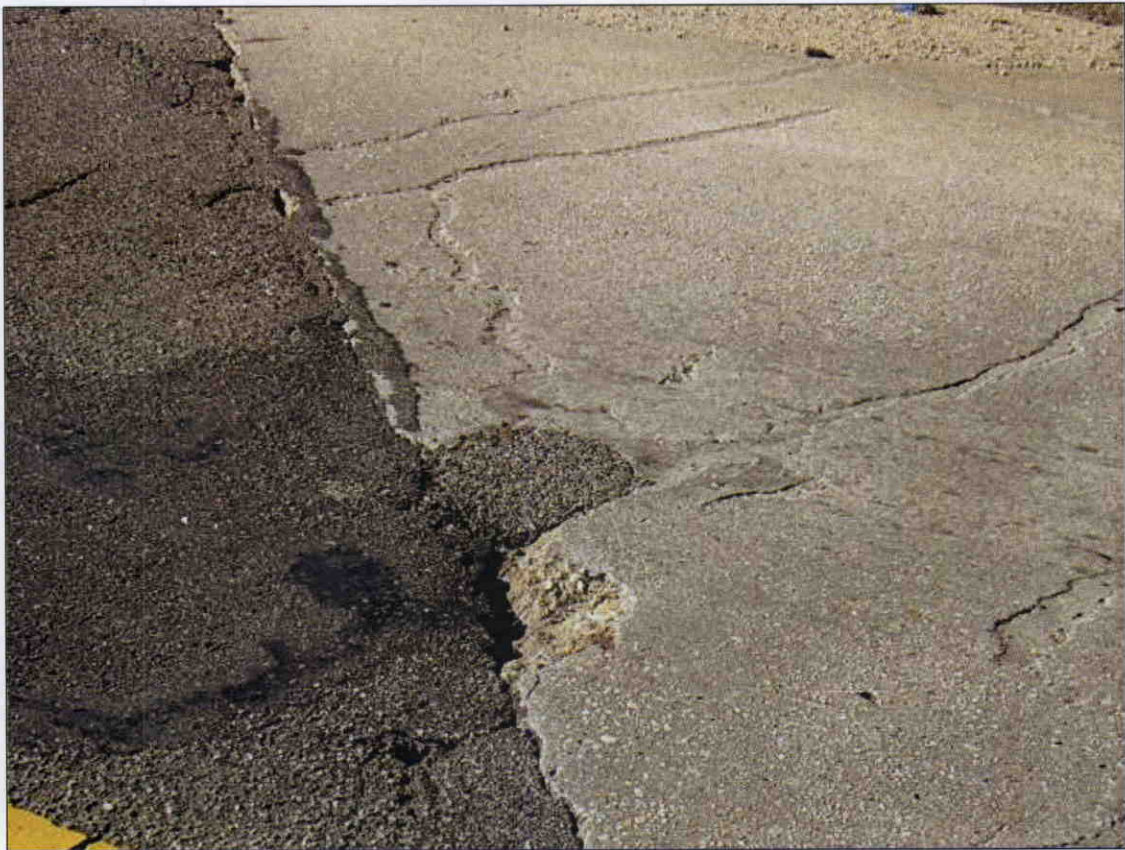
SPALLING IN DECK ALONG APPROACH END OF SPAN 1.
