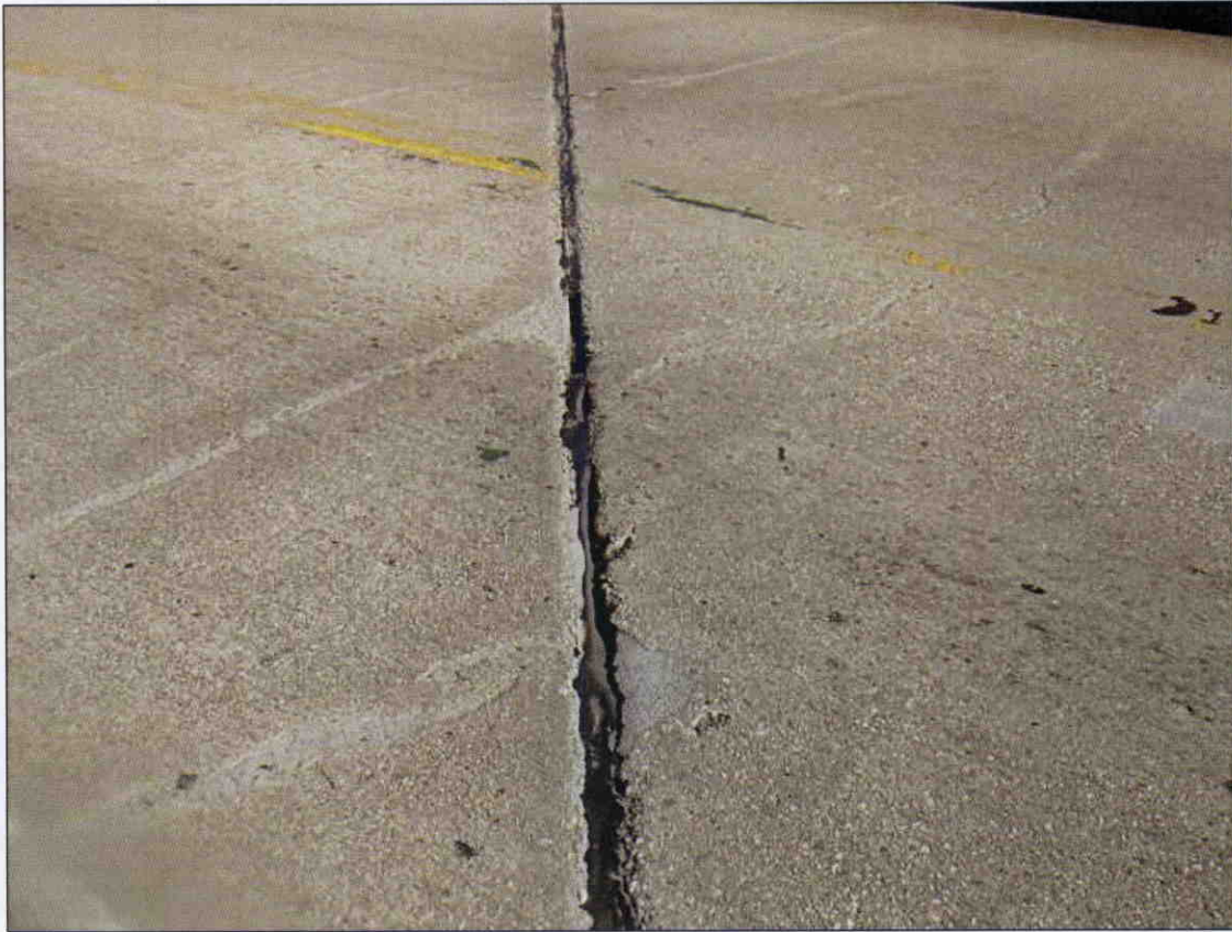
DETERIORATED JOINT AT PIER 3
