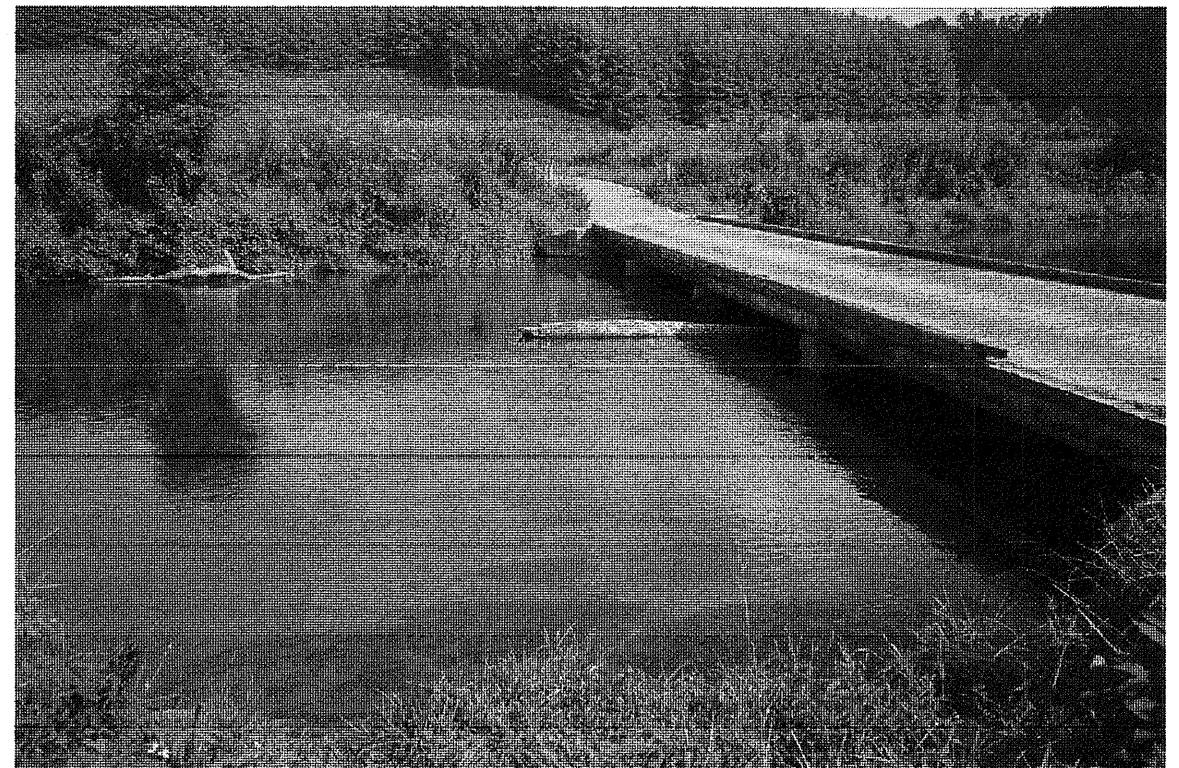
Looking Back At New Bridge Alignment -L- From East Bank of River
