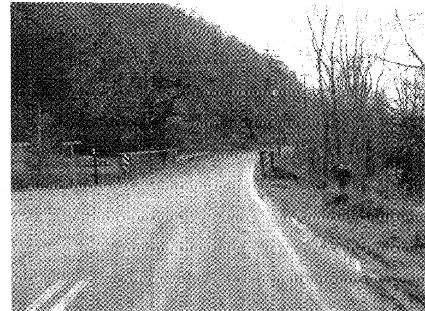
Photograph No. 14: This photograph was taken from the northwest approach along the centerline of the -L- alignment, looking southeast.
