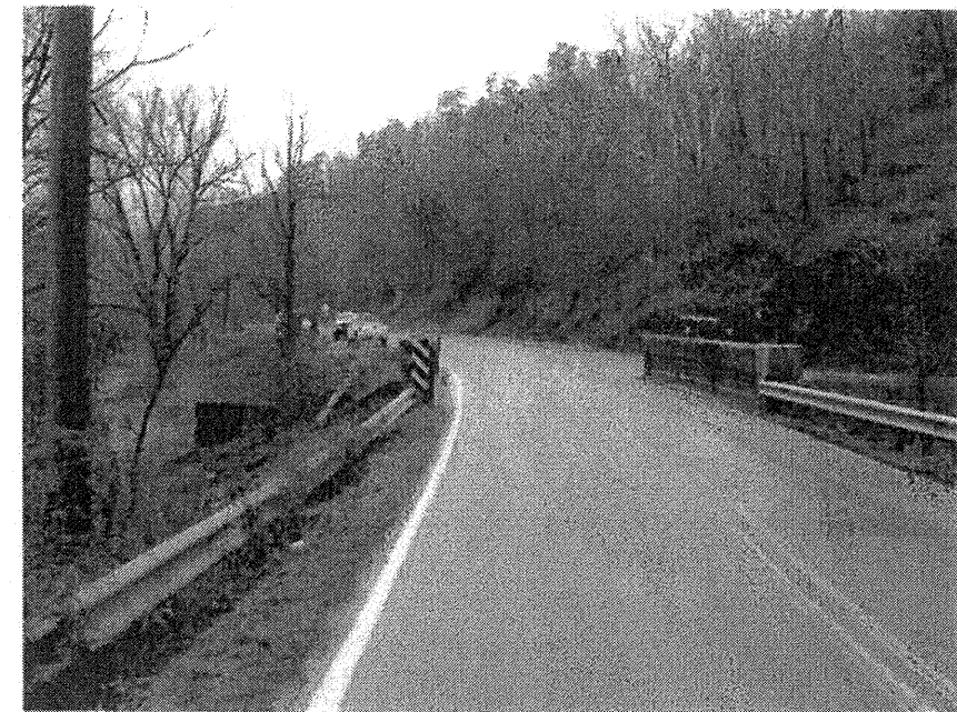
Photograph No. 1: This photograph was taken from the southeast approach along the centerline of the -L- alignment, looking northwest.
