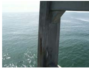
Delaminated Column with Rust Stains
