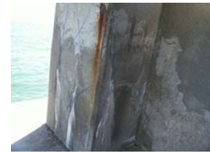
Delaminated Column with Rust and Efflorescence Stains
