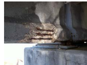
Spall at End of Girder
