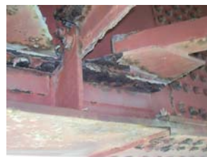
Corroded Gusset Plates on Steel Main Span
