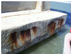
Delaminated Pile Cap with Heavy Rust Stains
