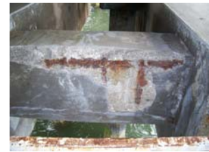
Spalled and Delaminated Crutch Bent Strut
