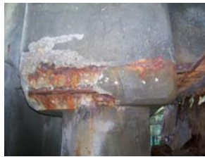
Spalled and Delaminated Sub-cap
