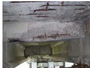
Spalled Deck and End Diaphragm
