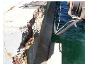
Spalled Sub-Girder with Heavy Rust Stains
