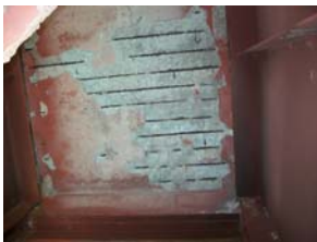
Spalled Concrete Deck Underside
