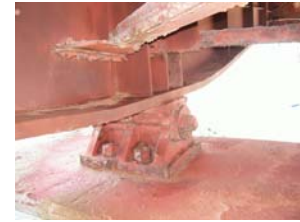
Corroded Lateral Bracing and Bearing
