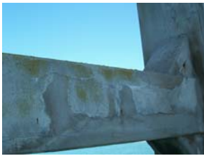
Delaminated High Level Bent Strut
