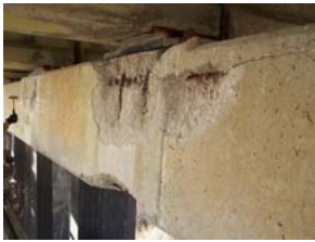
Spalled and Delaminated Bent Cap
