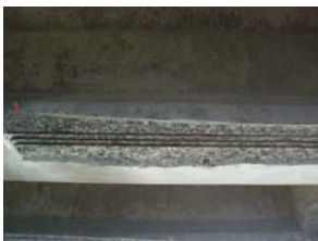
Spall with Exposed Strands on Girder (Prepared for Repair)
