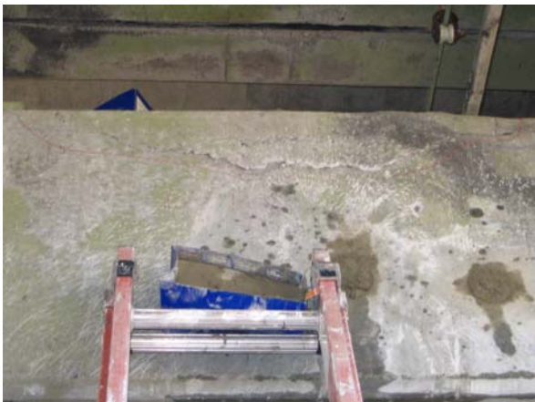
Bent 7; Crack on north face
