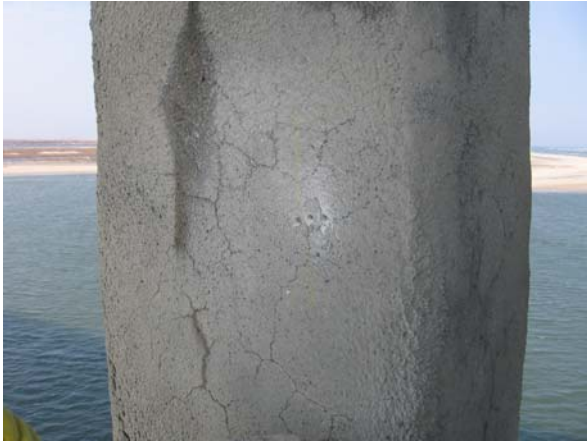
Bent 135, East column: east interior side, top 1/2
