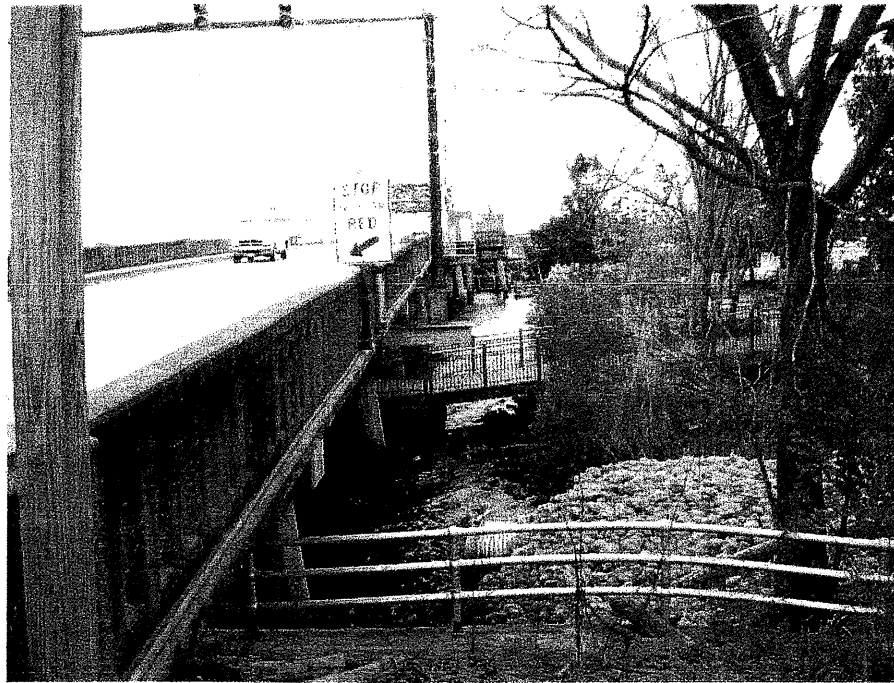
Photograph No. 13: This photograph was taken from left of the -L- alignment, looking south, along the existing bridge.
