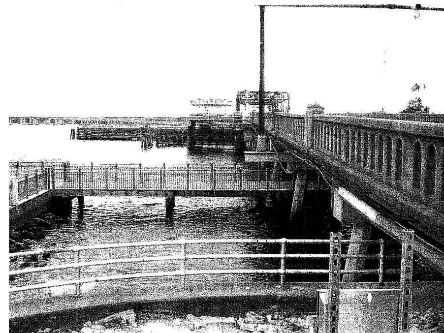
Photograph No. 12: This photograph was taken from right of the -L- alignment, looking south, along the existing bridge.
