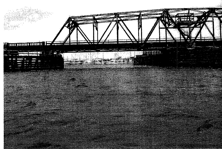
Photograph No. 7: This photograph was taken from right of the -L- alignment, looking west, at proposed Interior Bent No. 13.
