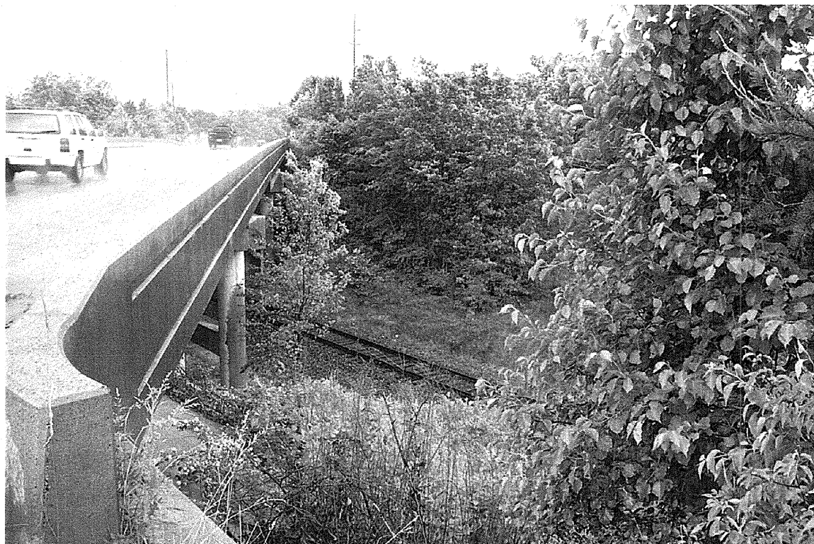
Photograph 2: View 9m Right of -L- From Top of Embankment at End Bent-1
